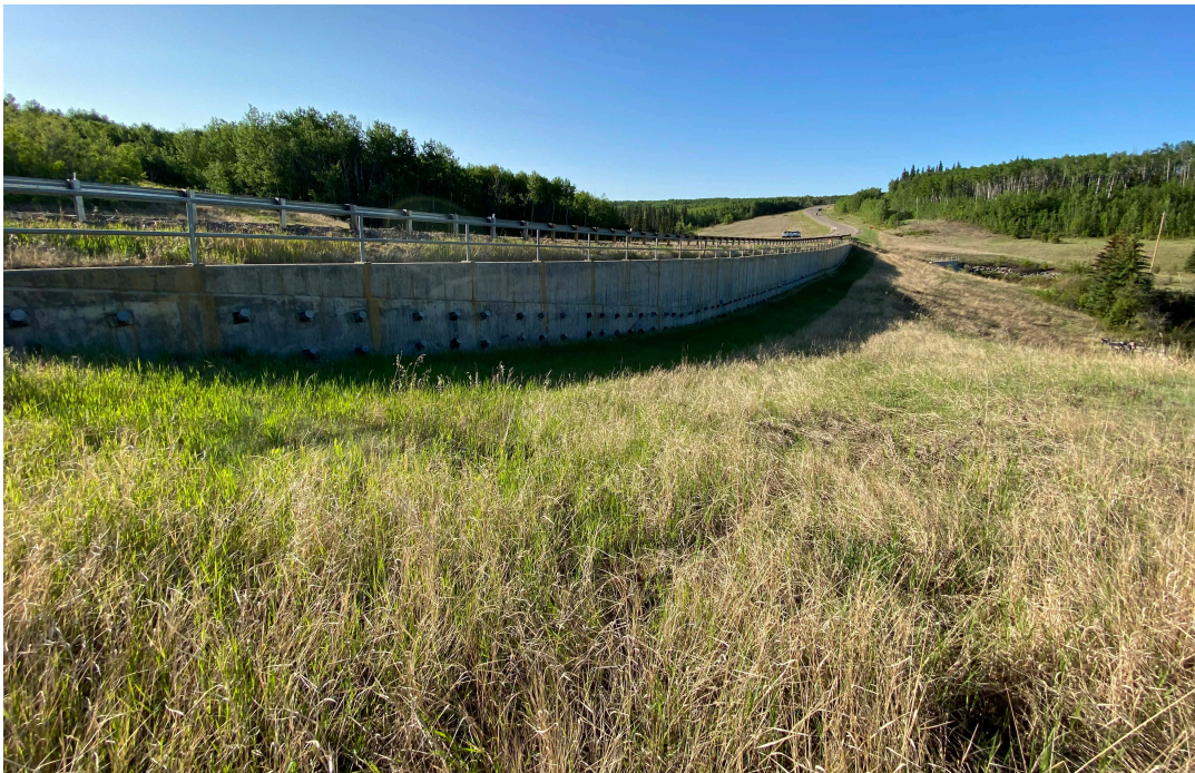
Photo 6 - Looking south along the upper pile wall and downslope embankment at Site 3.
