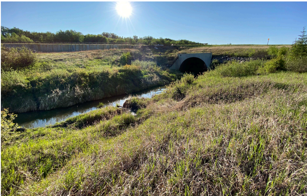
Photo 4 – Looking east at the body and scarp face of the slide between the south end of the pile wall and the arch culvert at Site 3.
