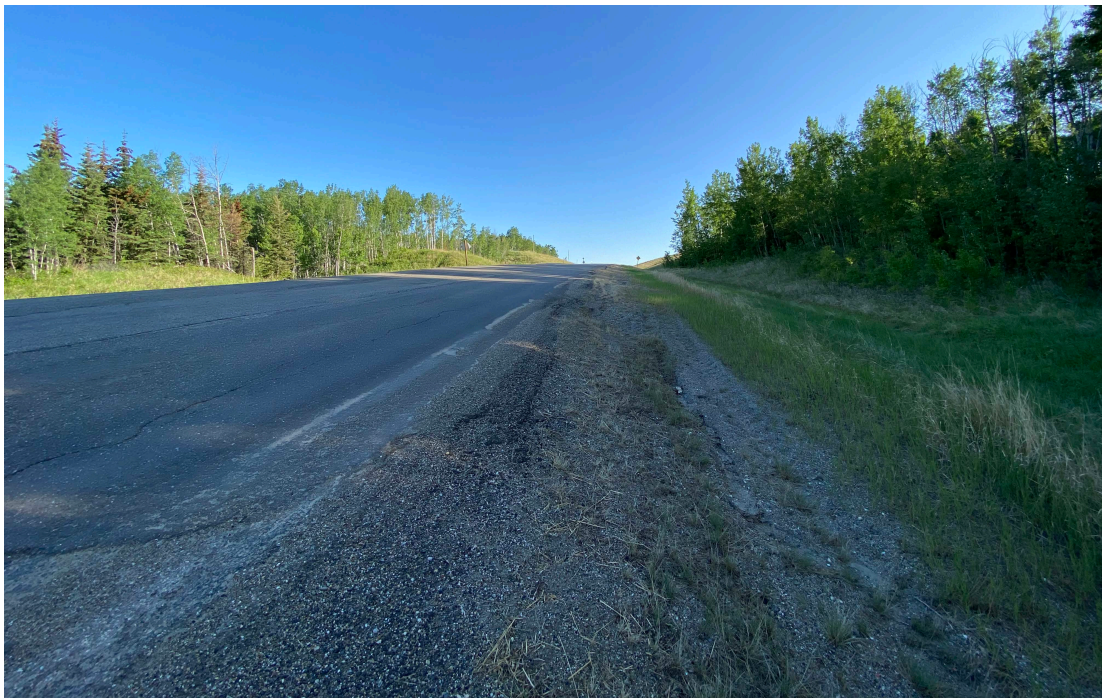
Photo 10 - Looking north along the east highway edge at where the slide scarp crosses the highway at Site 6.
