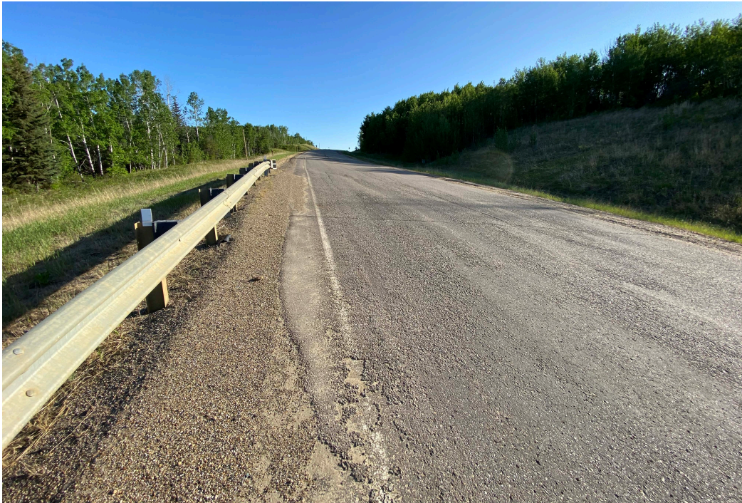
Photo 7 – Looking north along the highway at the north end of the guardrail and former patching at Site 5.
