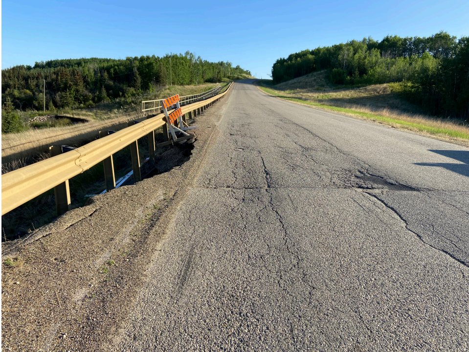
Photo 1 – Looking north along the highway south of the upper pile wall at the landslide that developed at Site 3.
