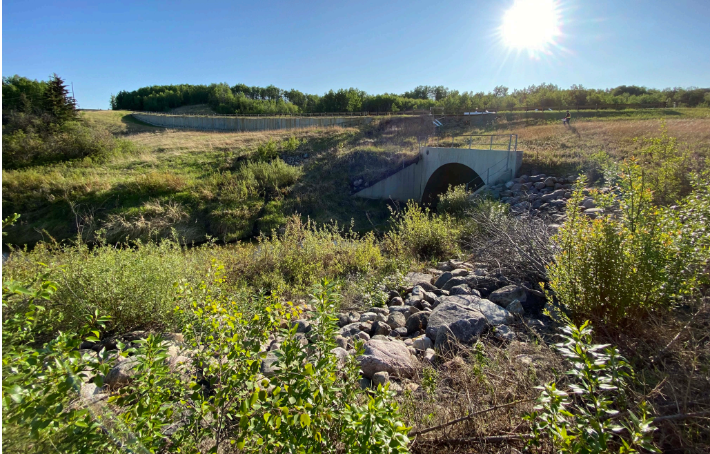
Photo 3 – Looking northeast at the slide that pushed debris against and around the arch culvert outlet headwall at Site 3. Note the cut trees growing again on the south side of the arch culvert.
