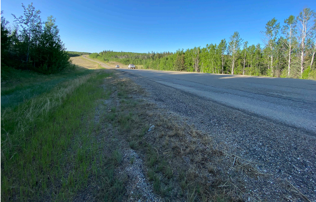
Photo 9 - Looking south along the highway at the subsidence in the NB driving lane and shoulder at Site 5.
