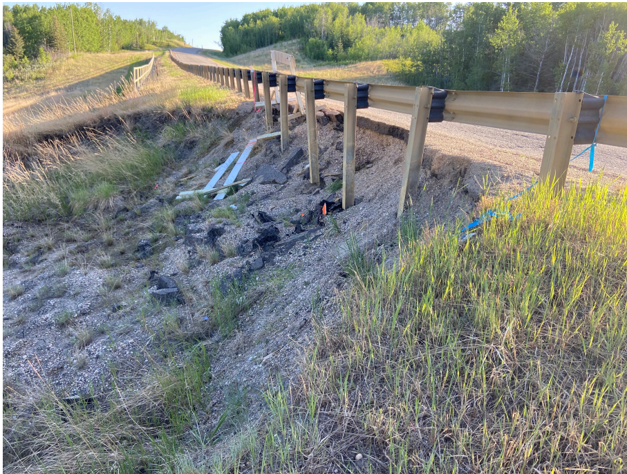
Photo 2 – Looking north at the slide scarp that has extended into the SB shoulder to within 0.25 m of the white line beyond the south end of the upper pile wall at Site 3.
