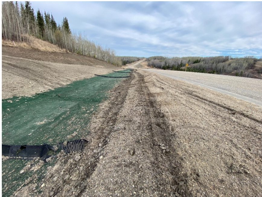
Photo 2 – Looking north along the west ditch of Site 2, at vehicle track ruts that caused damage to the ditch barriers.
