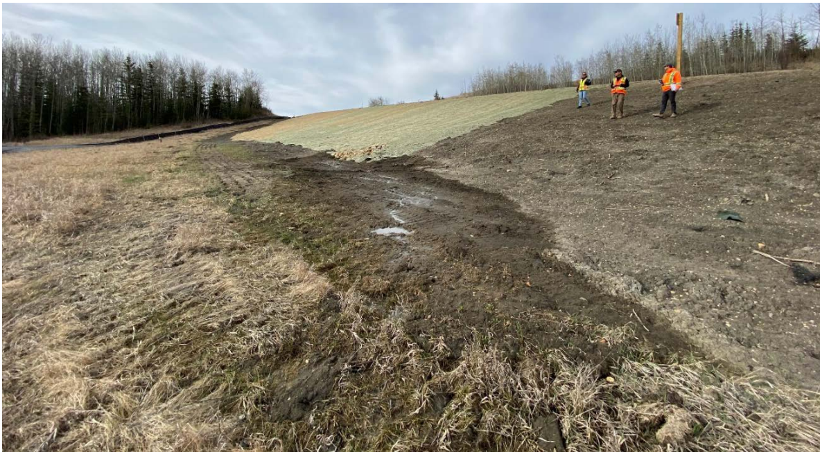
Photo 4 – Looking south along the east sideslope at steady seepage from the new subdrain outlet constructed beneath the new Lightweight Geofam fill at Site 2.
