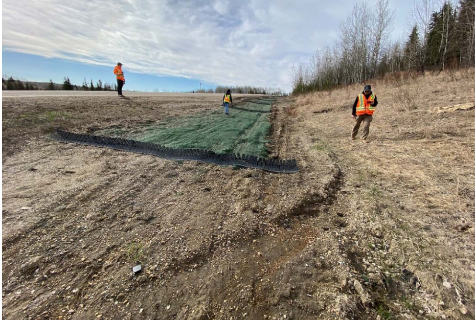
Photo 1 – Looking south along the west ditch at the east end of the TRM placement at Site 2.
