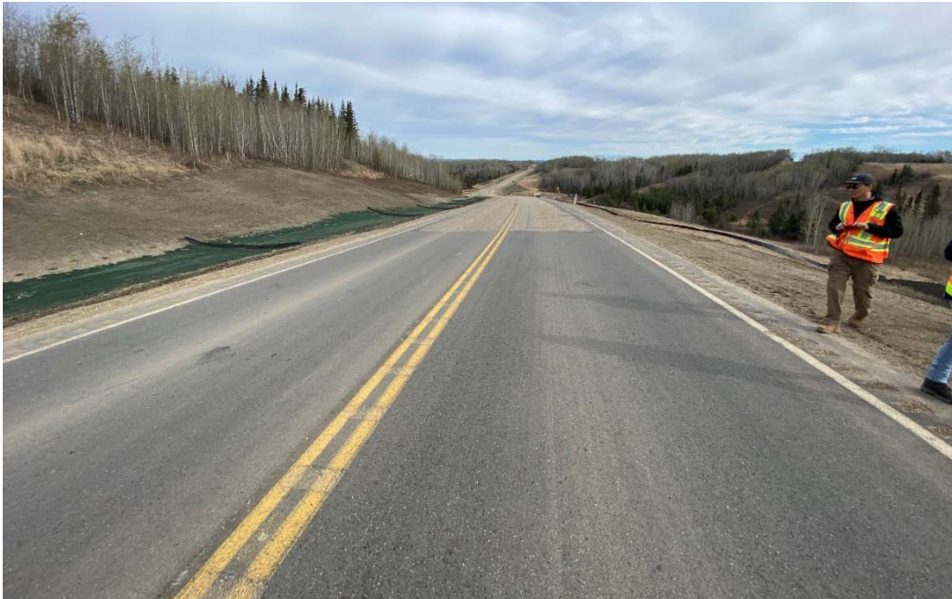
Photo 3 – Looking north along the freshly paved highway surface that was constructed over Lightweight Geofam fill at Site 2.
