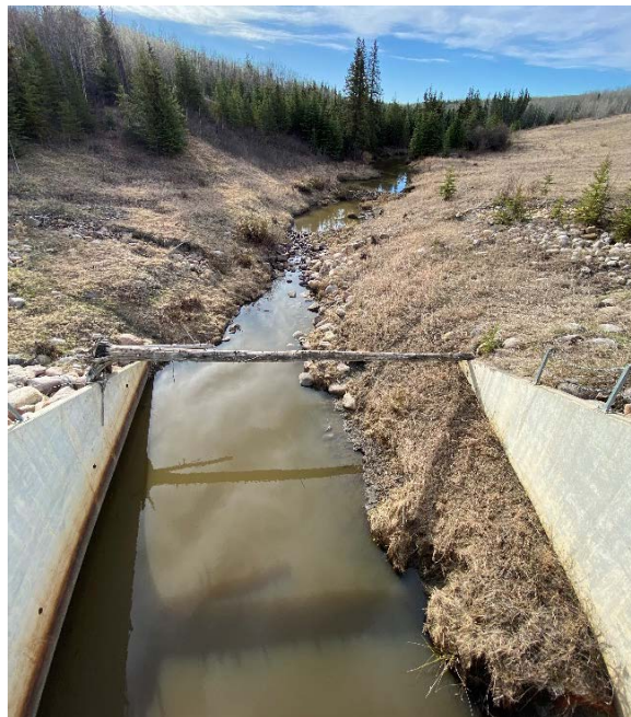
Photo 10 – Looking southeast along the Eureka River from the arch culvert inlet (Site 1).
