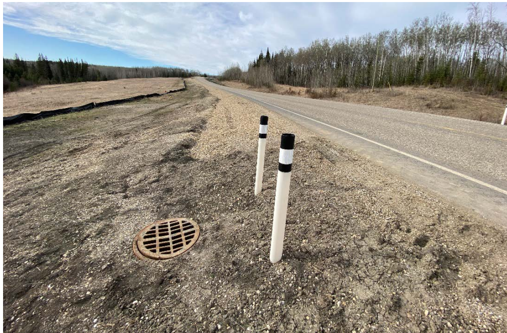
Photo 8 – Looking south from the north end of the Site 1 slide at the new surface water catch basin manhole that captures surface runoff from the new subdrain further south along the east edge of the highway, that drains into a smooth-wall steel pipe outletting further east. This replaced the previously existing AC curb/Manhole/Half-Culvert system.
