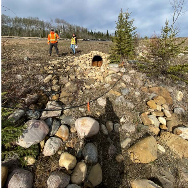
Photo 9 – Looking northwest at the new SWSP outlet (Site 1). Note the re-routed Telus cable at ground surface.
