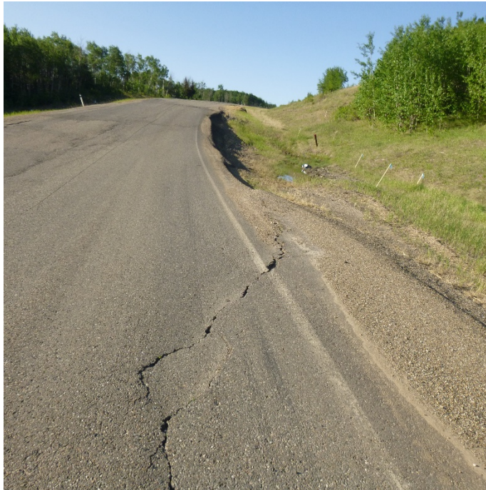
Photo 1 – Looking south at the slide scarp crossing the highway at Site 2, at the dip in the road that extends into the north ditch.
