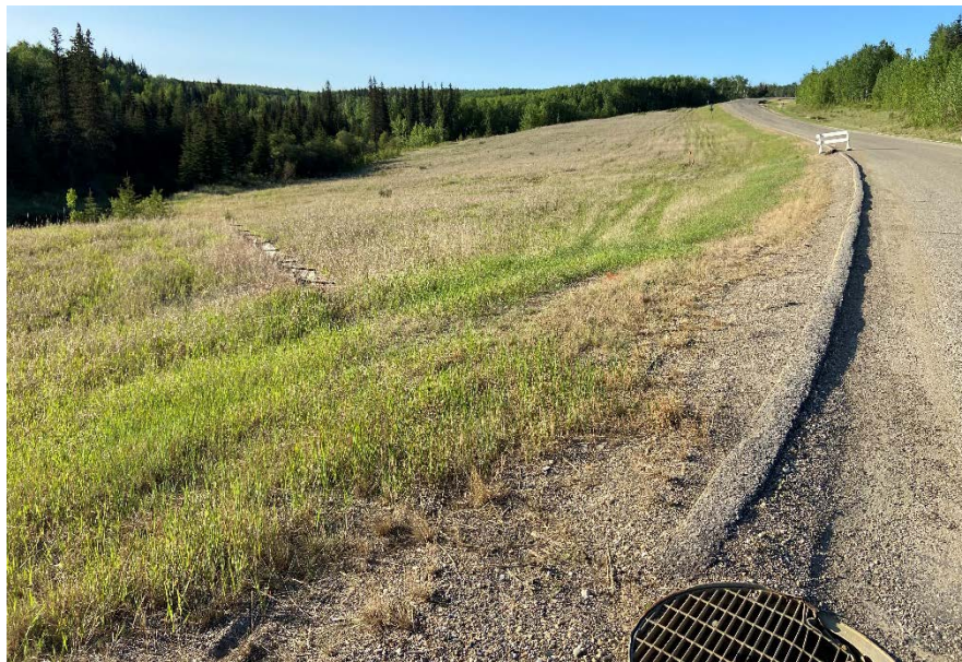
Photo 8 – Looking south from the north end of Site 1 slide. This surface water catch basin manhole on the edge of the highway draining to the half-culvert is to be replaced with a subdrain just off the east highway edge leading to a drop structure and into a smooth-wall steel pipe.
