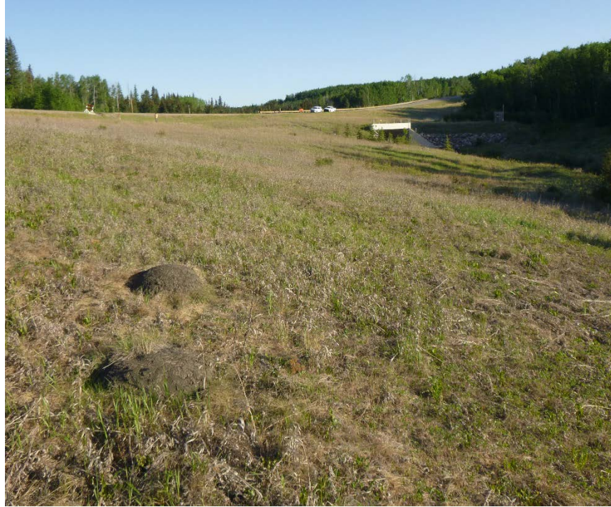
Photo 7 - Looking north across the Site 1 Slide from south of the river. Note the grassed over slide scarp parallel in the background to the highway.
