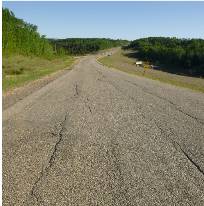
Photo 3 – Looking north along the fatigued highway pavement across slide Site 4.
