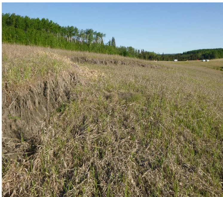
Photo 6 – Looking northwest along the fresh slide scarp/crack of Site 2, from just north of the most active portion of the slide.
