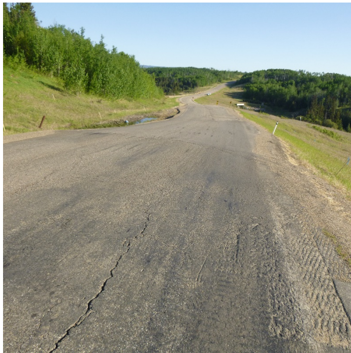
Photo 2 – Looking north from the Slide Site 2 at the milled/patched pavement. Note the fresh, well-defined reflective north end scarp crack extending across the road.
