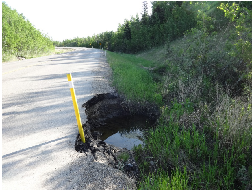
Photo 1. Looking northeast at where water has eroded the highway. Photo credit: Nicole Wilder.
