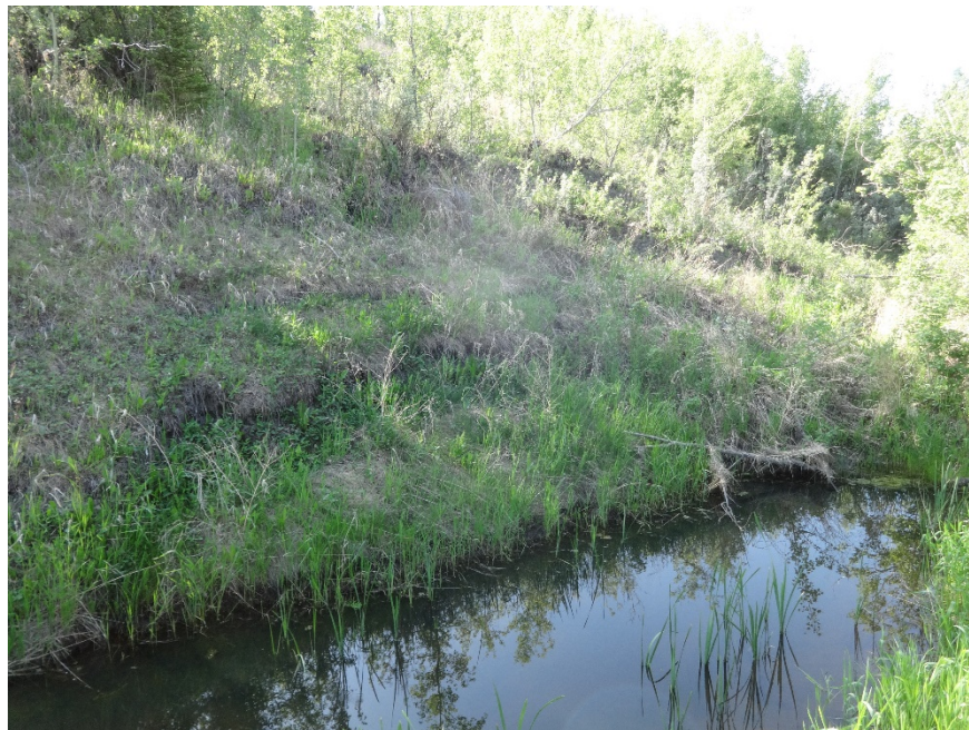
Photo 9. Looking southeast at scarps above ponded water near toe of the landslide. Photo credit: Nicole Wilder.
