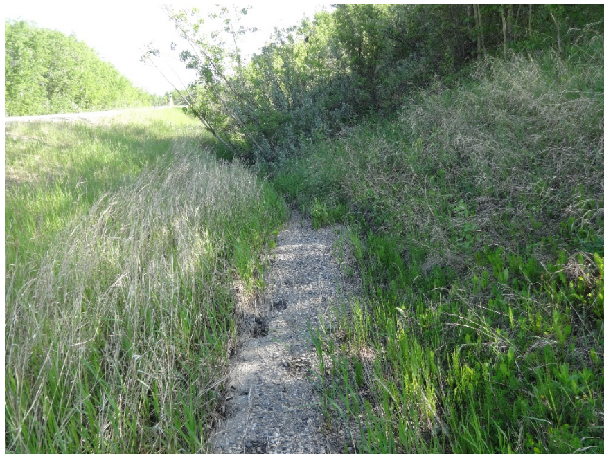
Photo 12. Looking north at where erosion continues south of main area. Photo credit: Nicole Wilder.
