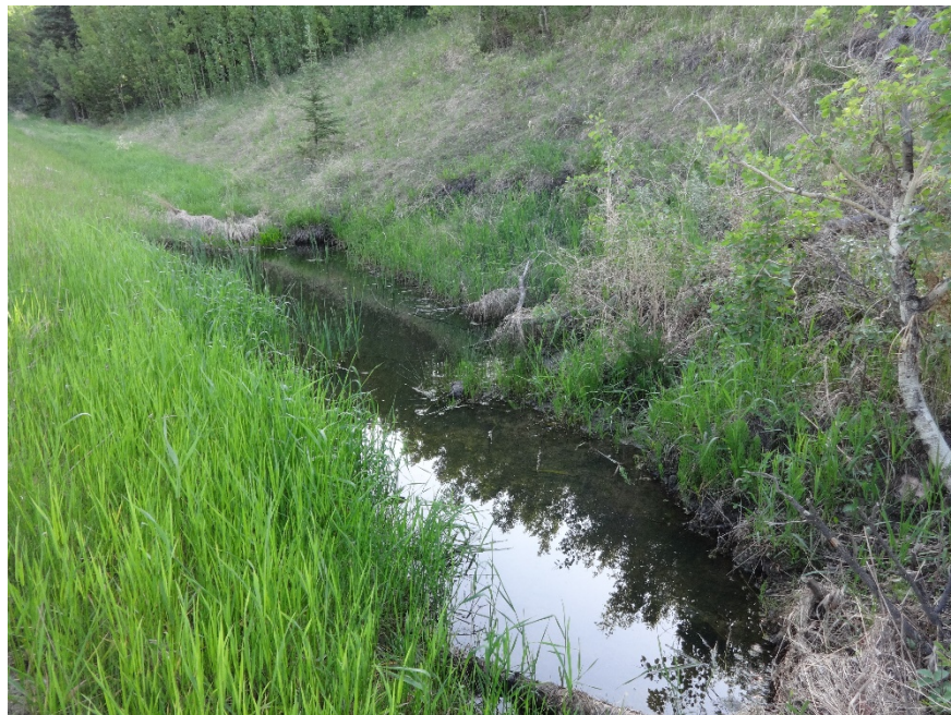
Photo 3. Looking northeast at where water has ponded north of where pavement was affected. Photo credit: Nicole Wilder.
