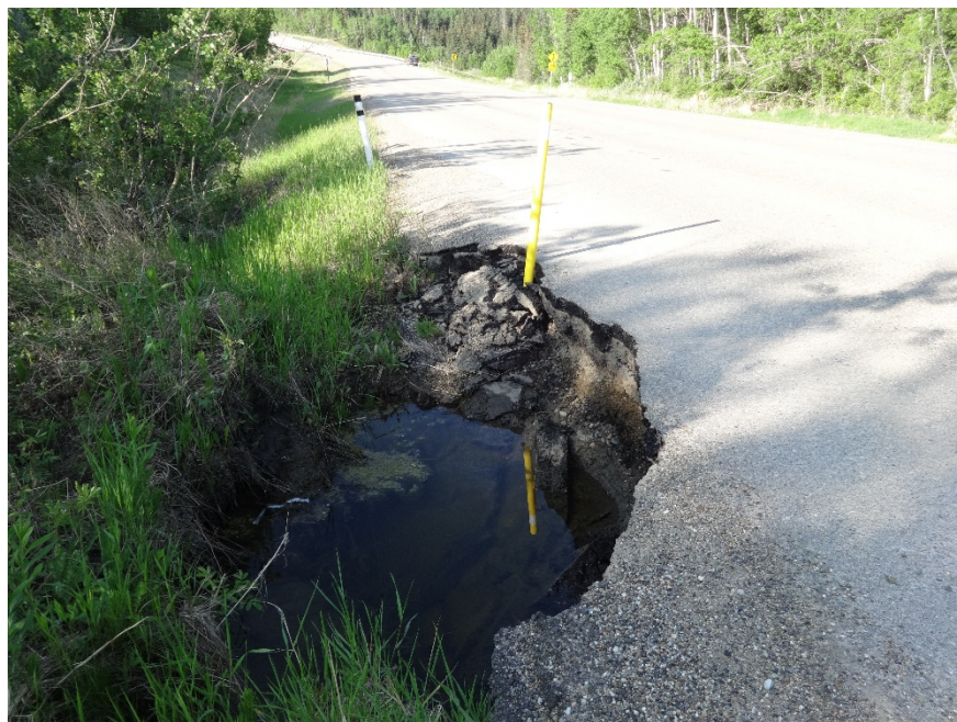
Photo 2. Looking southwest at where water has eroded the highway. Photo credit: Nicole Wilder.
