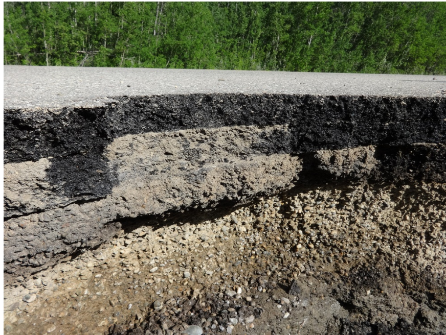
Photo 13. Looking west at where pavement has been eroded. Photo credit: Nicole Wilder.
