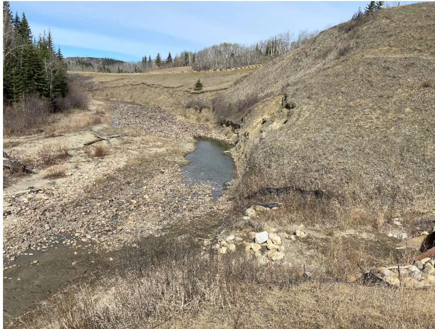
Photo 9. Looking west at river erosion and culvert outlet area of PH077-2. Photo Credit: Don Proudfoot.
