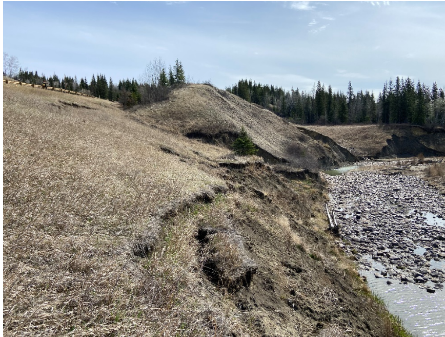
Photo 1. Looking east at Slide PH077-1 at the erosion along the north side of the Creek. Photo credit: Don Proudfoot.
