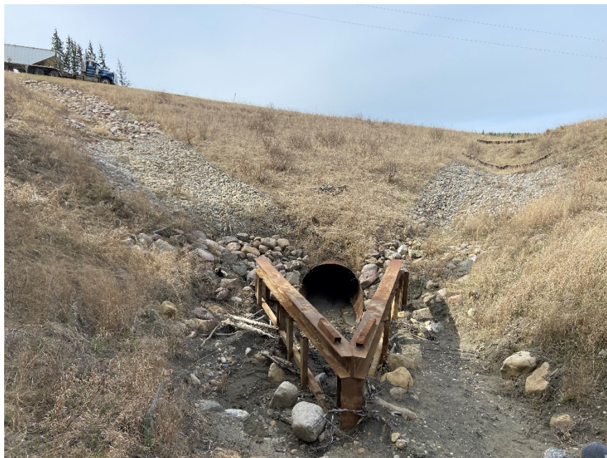
Photo 12. Looking south at the culvert inlet area at PH077-2, the trash rack appeared half full of debris. Photo Credit: Don Proudfoot.
