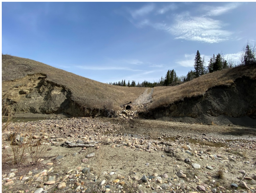
Photo 6. Looking north at culvert outlet and river bank erosion and sloughing on either side. Photo Credit: Don Proudfoot.
