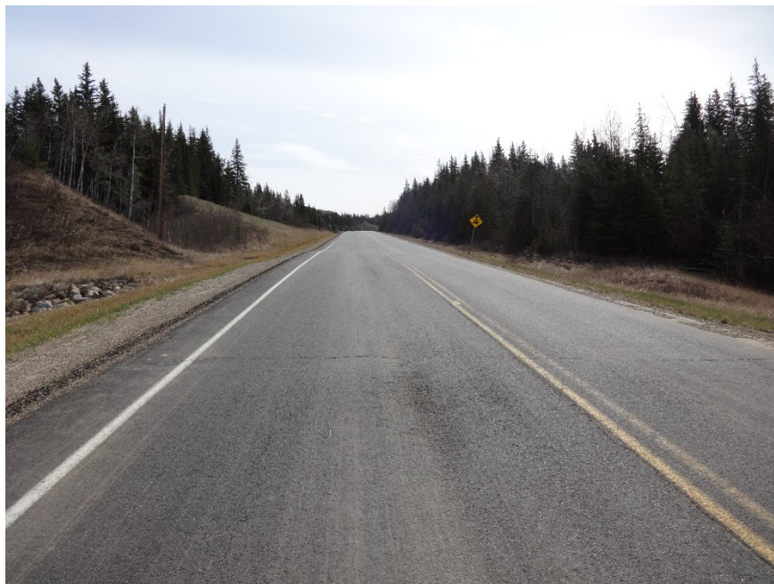
Photo 14. Looking east at the dip in the highway. Photo credit: Don Proudfoot.
