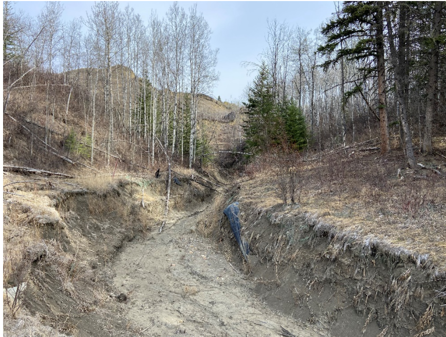
Photo 11. Looking north at eroded tributary creek channel leading into the culvert inlet north of the highway at PH077-2. Photo Credit: Don Proudfoot.
