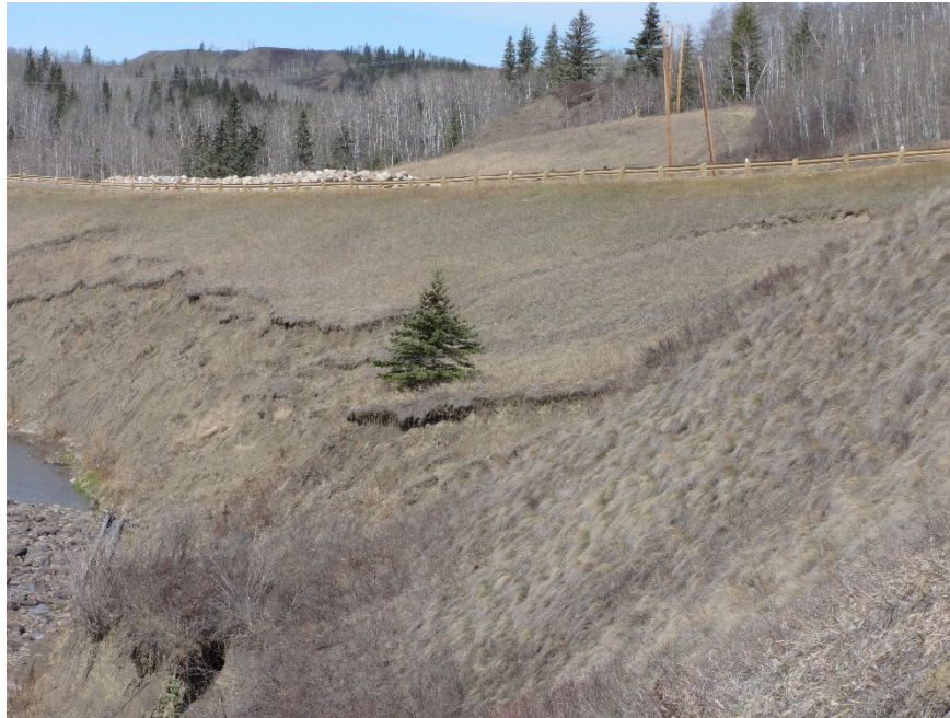
Photo 3. Looking west at the fresh toe slumping above the creek at PH077-1 in the south highway embankment. Photo credit: Nicole Wilder.
