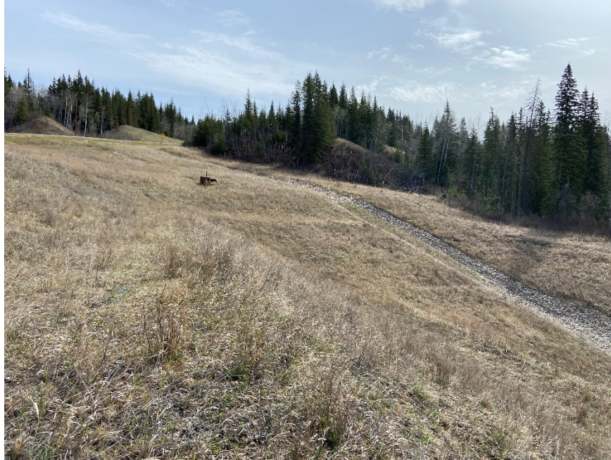
Photo 7. Looking east at riprap swale into the gabion mattress channel of PH077-2. Photo Credit: Don Proudfoot.
