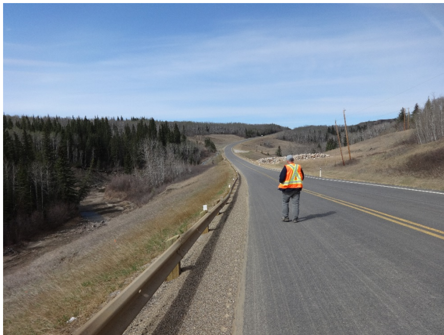
Photo 4. Looking west along the highway at where crack in the highway was (before overlay) above the Slide at PH077-1 The dip is still evident. Photo credit: Nicole Wilder.
