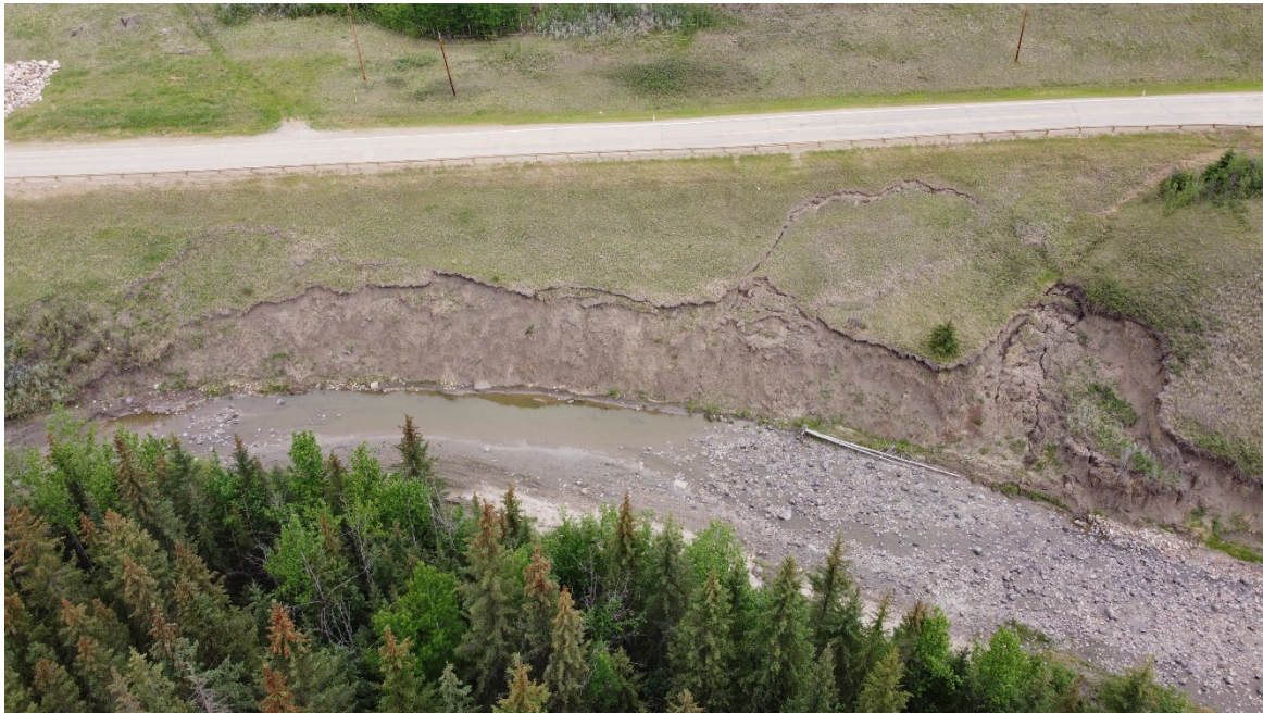
Photo 15. Looking north at slumping riverbank at PH077-1. Drone Photo Credit: Don Proudfoot.
