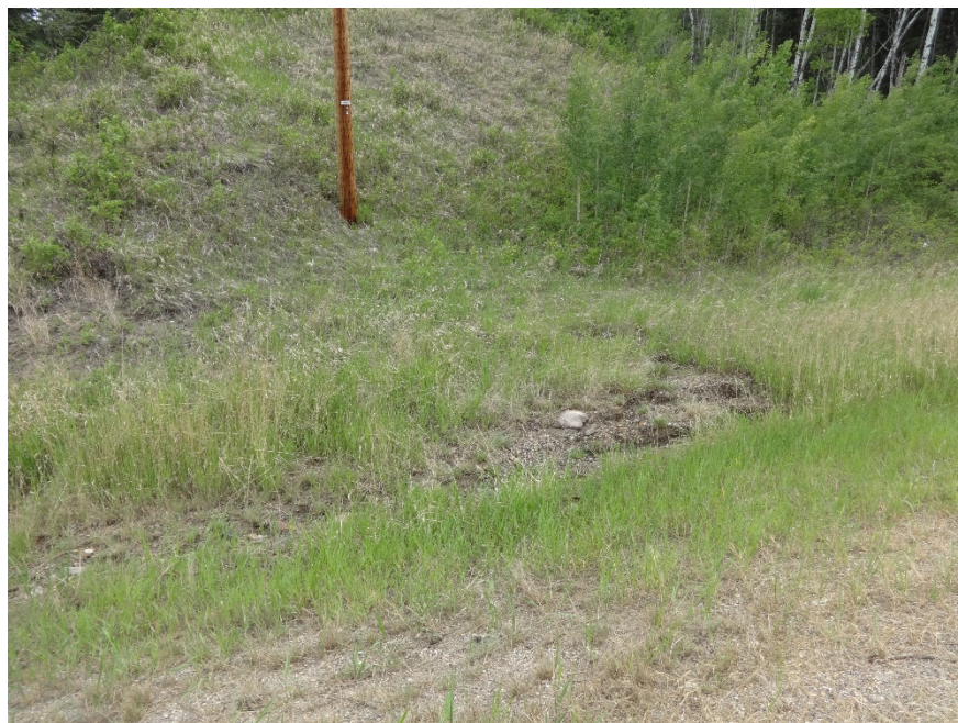
Photo 9. Looking north at new erosion noted upslope from the riprap. Photo Credit: Nicole Wilder.
