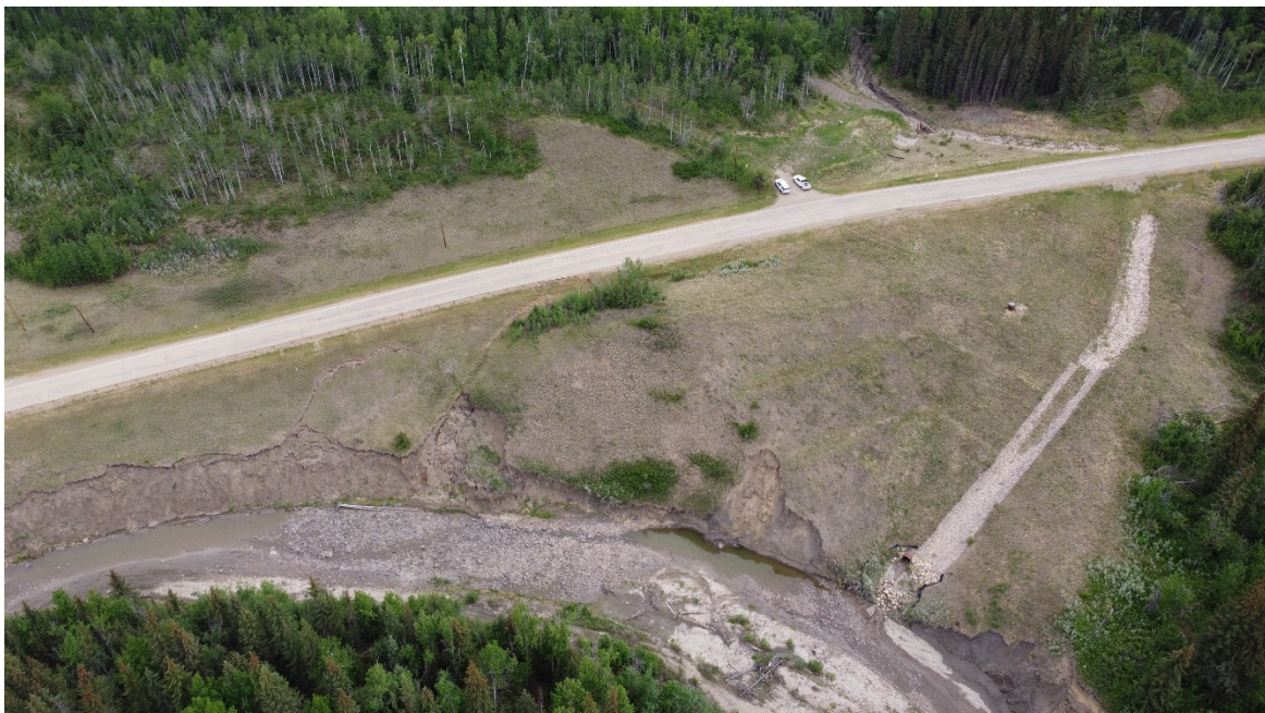
Photo 14. Looking north at Slumping riverbank at PH077-1/2. Drone Photo Credit: Don Proudfoot.
