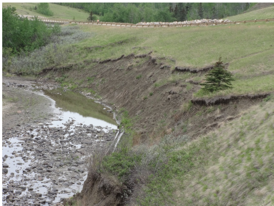
Photo 2. Looking west at the fresh toe slumping above the creek at PH077-1 in the south highway embankment. Photo credit: Nicole Wilder.
