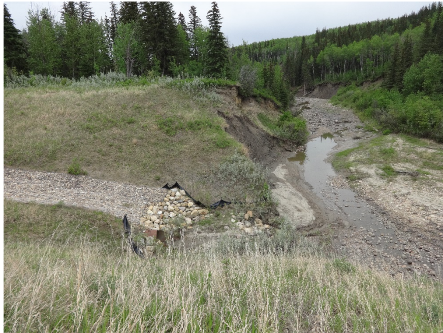
Photo 7. Looking east at the southeast ditch drainage channel of PH077-2, Hines Creek. Photo Credit: Nicole Wilder.
