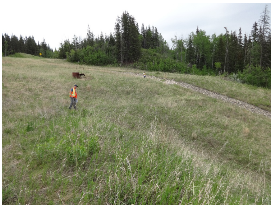
Photo 6. Looking east at riprap swale into the gabion mattress channel of PH077-2. Photo Credit: Nicole Wilder.
