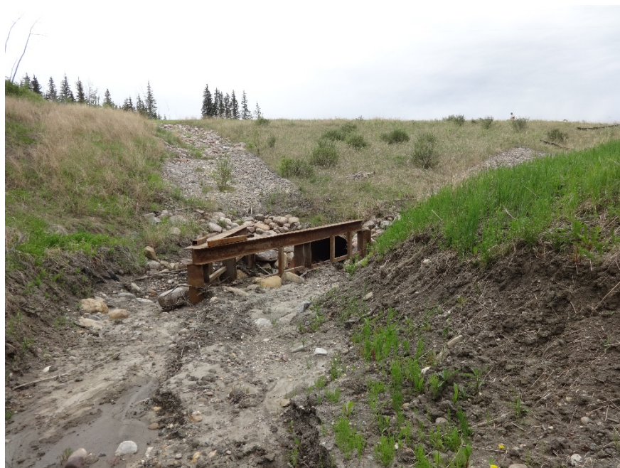
Photo 10. Looking south at the culvert inlet area at PH077-2, the trash rack appeared slightly less full of debris. Photo Credit: Nicole Wilder.
