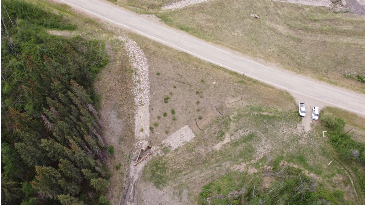
Photo 13. Looking southeast at north sideslope of highway at culvert inlet at PH077-2. Drone Photo Credit: Don Proudfoot.
