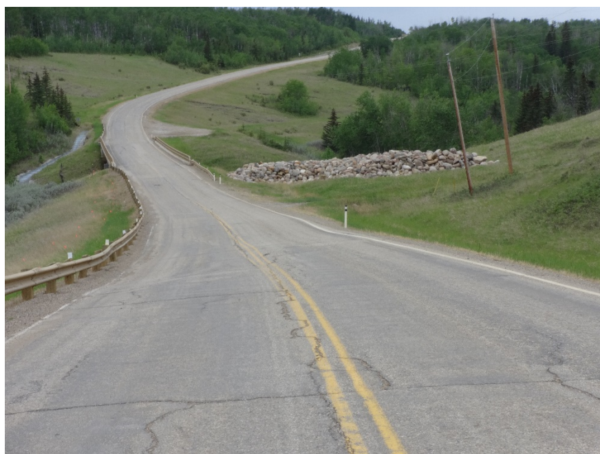
Photo 4. Looking west along the highway at the crack/dip in the highway above the Slide at PH077-1. Photo credit: Nicole Wilder.
