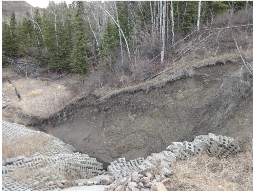
Photo 9. Looking north at the slumping and infill occurring into the channel upstream of the 1524 SWSP culvert entrance. Photo Credit: Nicole Wilder.
