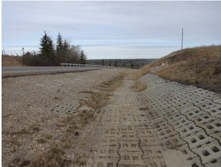
Photo 15. Looking west at east end of ACB mat lining. Photo Credit: Nicole Wilder.
