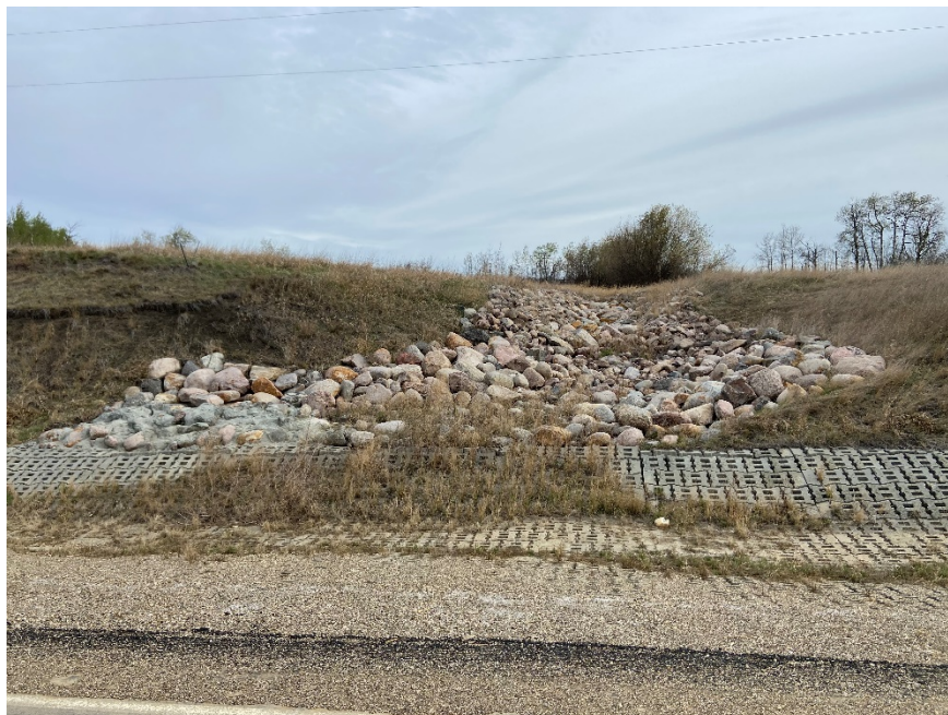
Photo 14. Looking north at where riprap was previously placed, appears to be in good condition but a scarp has extended to the west of it. Photo Credit: Don Proudfoot.
