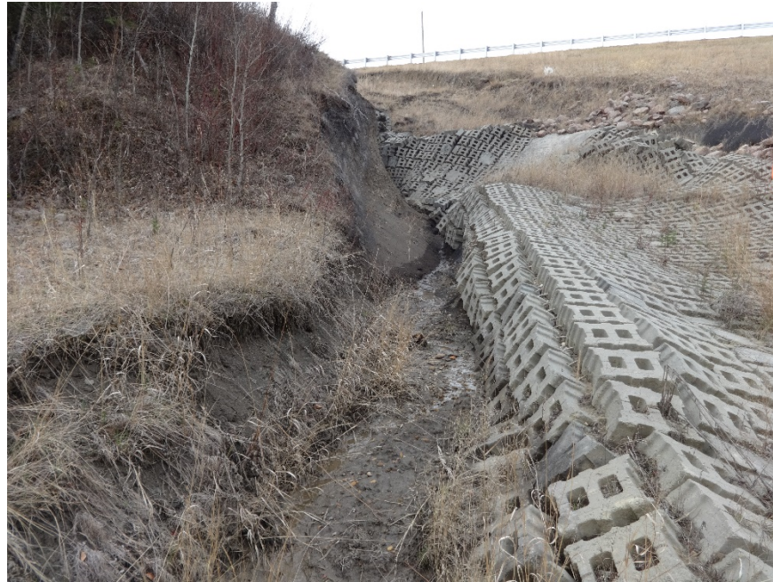
Photo 5. Looking southeast along the east edge of the eroded ACB mats. Here the mats have slid down into the deeply eroded channel and water flows along here. Photo Credit: Nicole Wilder.
