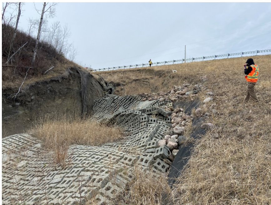
Photo 4. Looking southeast at the severe erosion through the ACB mats. Note the enlarged erosion and slide developing south of the mats. Photo credit: Nicole Wilder.
