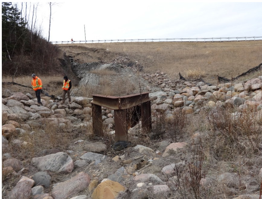
Photo 8. Looking southwest at the culvert inlet, trash rack and eroded ACB mat area leading to it. Photo Credit: Nicole Wilder.
