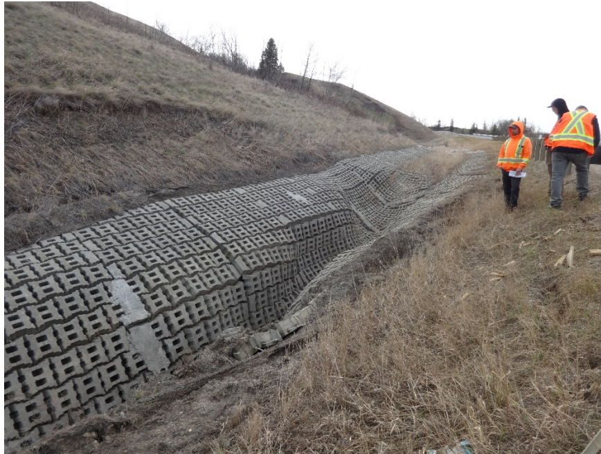
Photo 1. Looking east along the beginning of the eroded ACB mat area north of the highway. Photo credit: Nicole Wilder.
