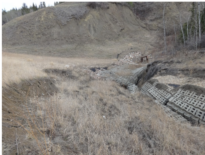
Photo 6. Looking north along the southwest side of the damaged and eroded ACB mats. Photo Credit: Nicole Wilder.
