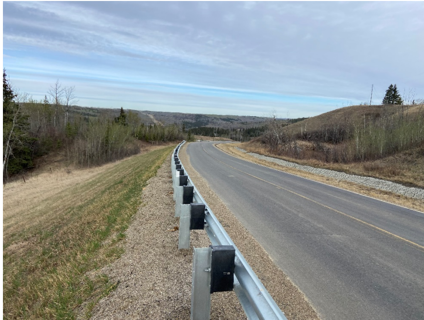
Photo 13. Looking northwest towards sag pond and dip in highway. Photo Credit: Nicole Wilder.
