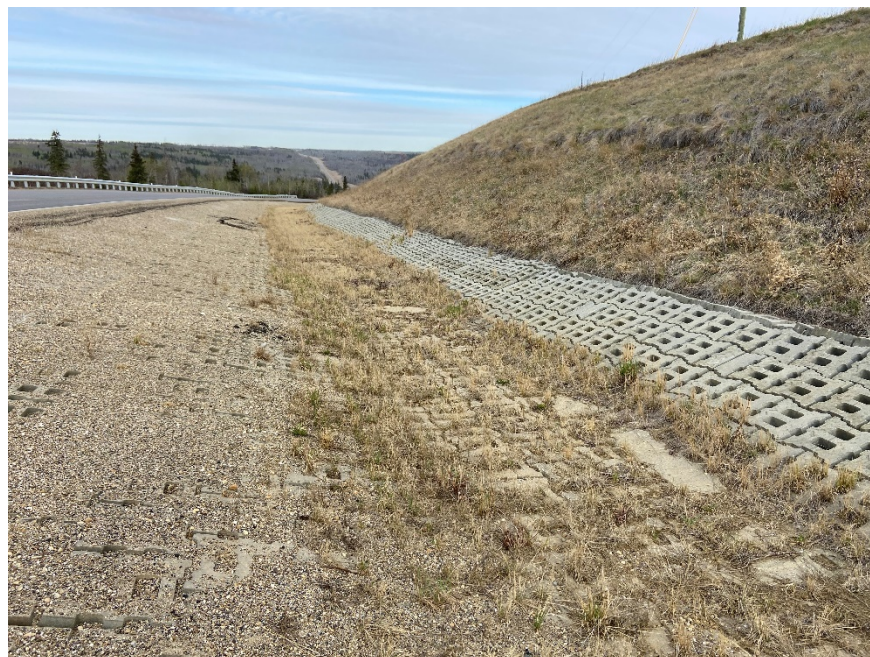
Photo 12. Looking northwest at the ACB Matting performing well and previously had some willows growing out of them which were cut. Photo Credit: Nicole Wilder.
