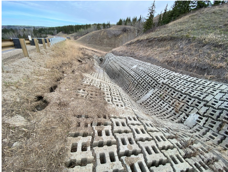
Photo 3. Looking northwest along the severely damaged ACB mat area and enlarged slide scarp area. Photo credit: Don Proudfoot.
