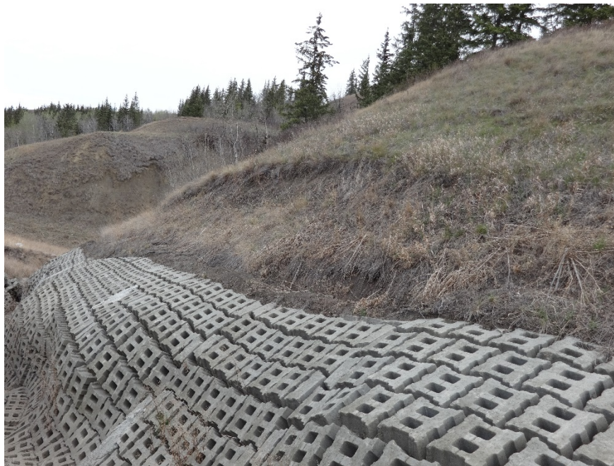
Photo 2. Looking north along the edge of the eroded ACB mat area. Note the scarp extension along the north edge of the mats. Photo credit: Nicole Wilder.
