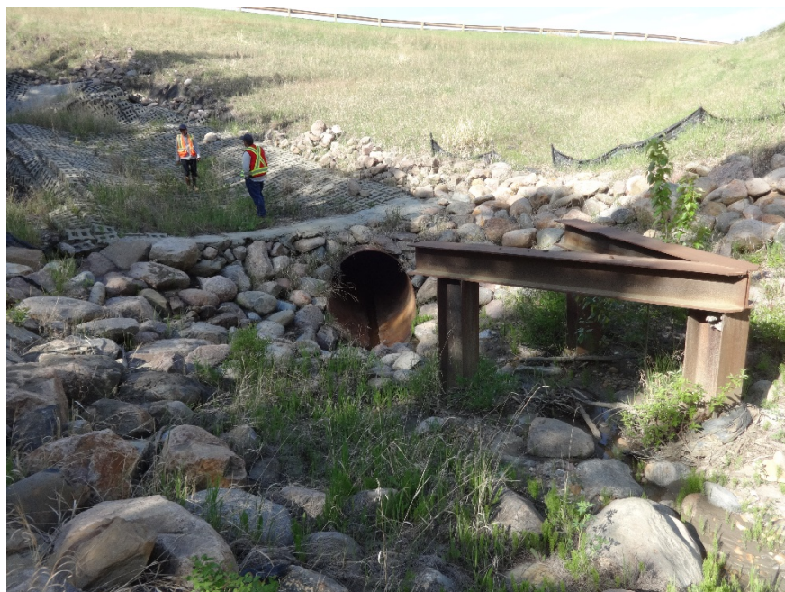
Photo 8. Looking southwest at the culvert inlet, trash rack and eroded ACB mat area leading to it. Photo Credit: Nicole Wilder.
