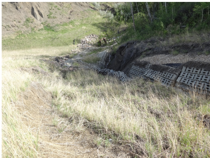
Photo 6. Looking north along the southwest side of the damaged and eroded ACB mats. Photo Credit: Nicole Wilder.
