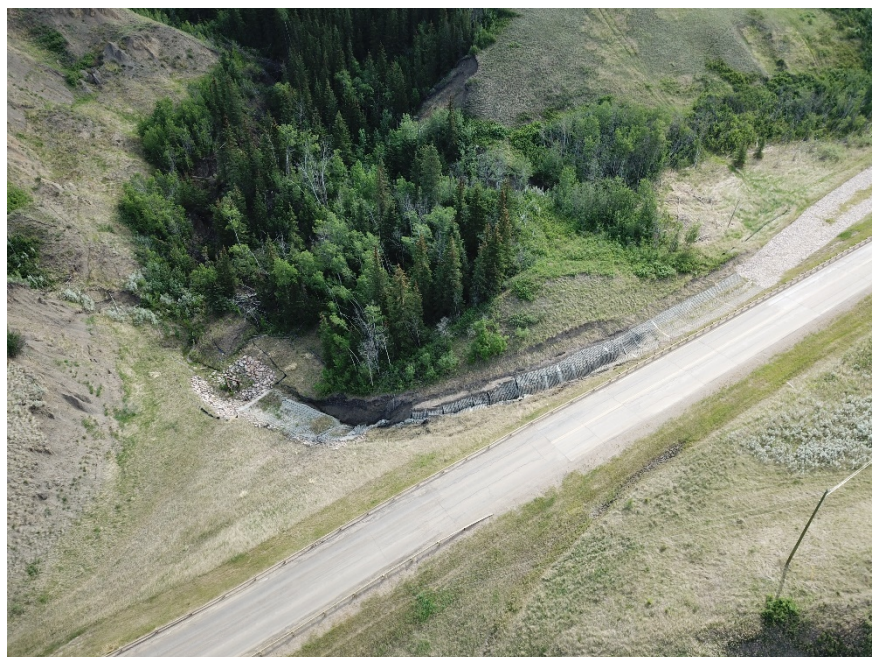
Photo 16. Looking northeast down at eroded ACB blocks and channel along them. Photo Credit: Drone-Nicole Wilder.
