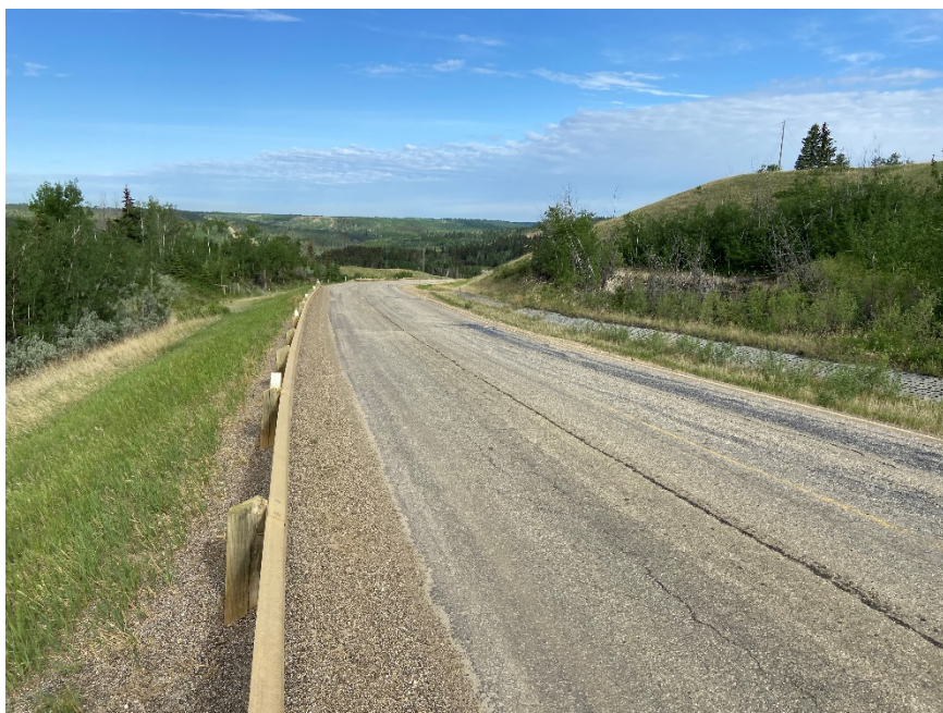
Photo 14. Looking northwest at cracks in asphalt and dip in highway. Photo Credit: Nicole Wilder.
