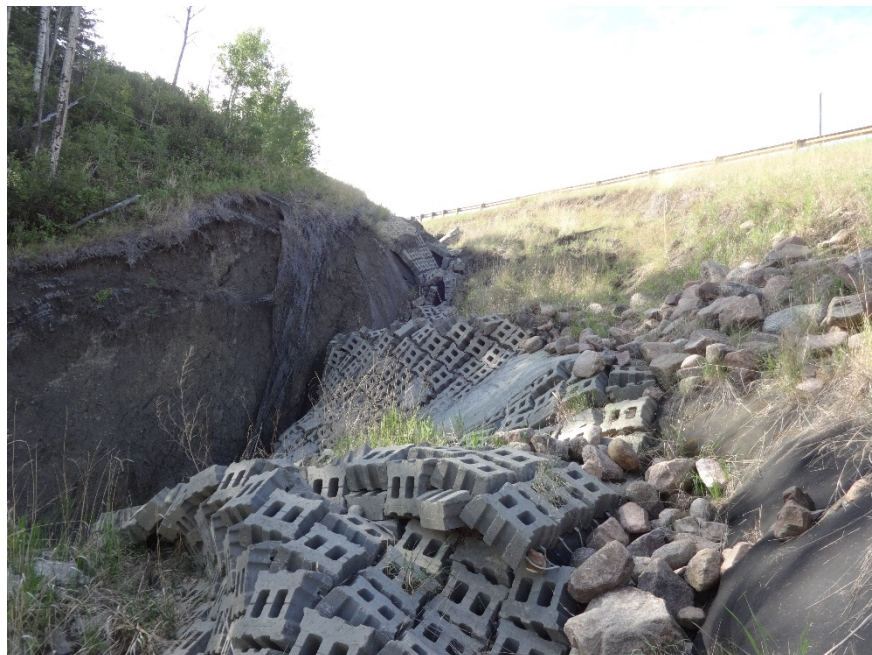
Photo 4. Looking southeast at the severe erosion through the ACB mats. Note the enlarged erosion and slide developing south of the mats. Photo credit: Nicole Wilder.
