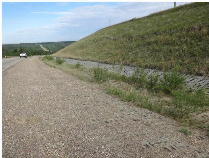
Photo 15. Looking northwest at the ACB Matting performing well but had some willows growing out of them. Photo Credit: Nicole Wilder.
