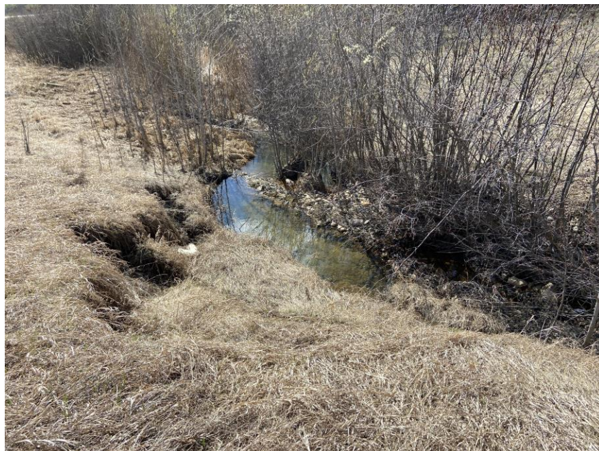
Photo 16 - Looking west at the erosion in the north ditch channel at the completely eroded gabion liner between the 760 SWSP and 1200 CSP outlets.
