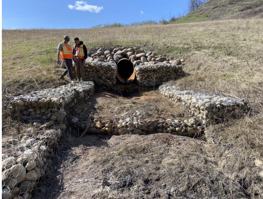
Photo 7 – Looking north at the 900 SWSP outlet and gabion outlet structure. There was significant ice inside this pipe this year.
