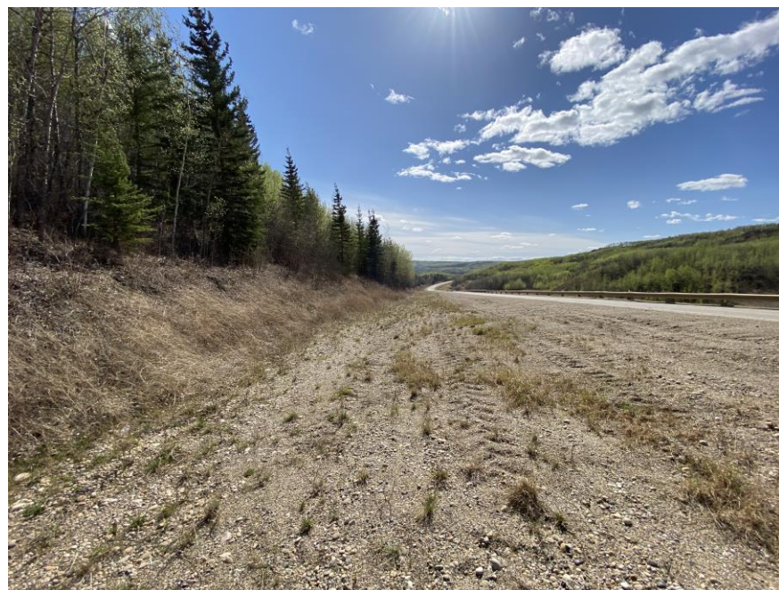
Photo 4 – Looking west along the south ditch channel and hwy embankment that was lined with 6-80 gravel.
