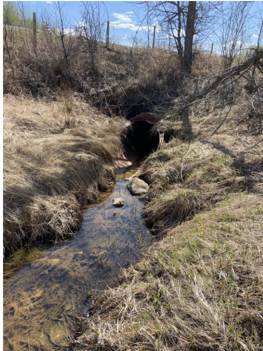
Photo 11 - Looking southwest at the 1040 SWSP inlet, at the west end of the north ditch channel.
