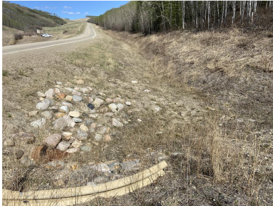
Photo 1 – Looking east along the south ditch at the ditch block and inlet of the 810 CSP on the south side of the hwy embankment.
