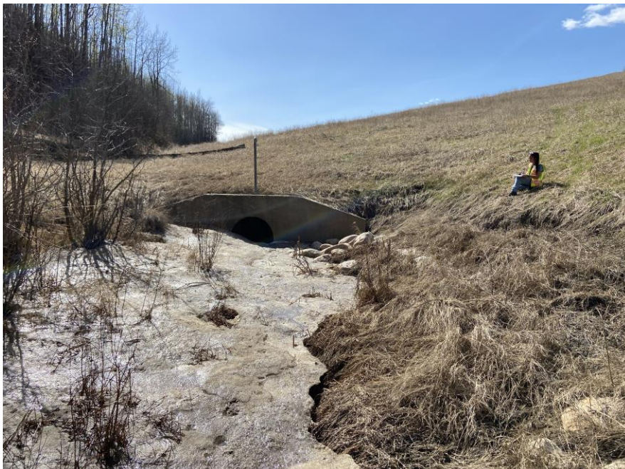
Photo 6 - Looking northwest at the 1200 CSP inlet headwall. Note the ice build-up in the channel in front of the culvert.
