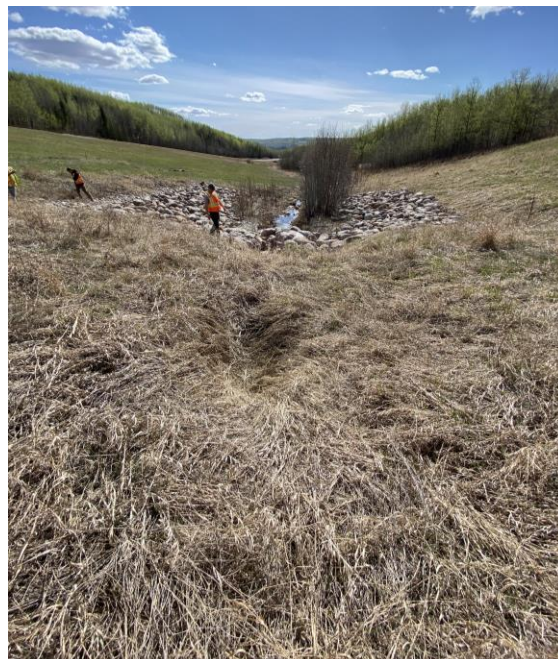
Photo 18 – Looking west at the 1200 culvert outlet area. Note the old subsidence behind the riprap.
