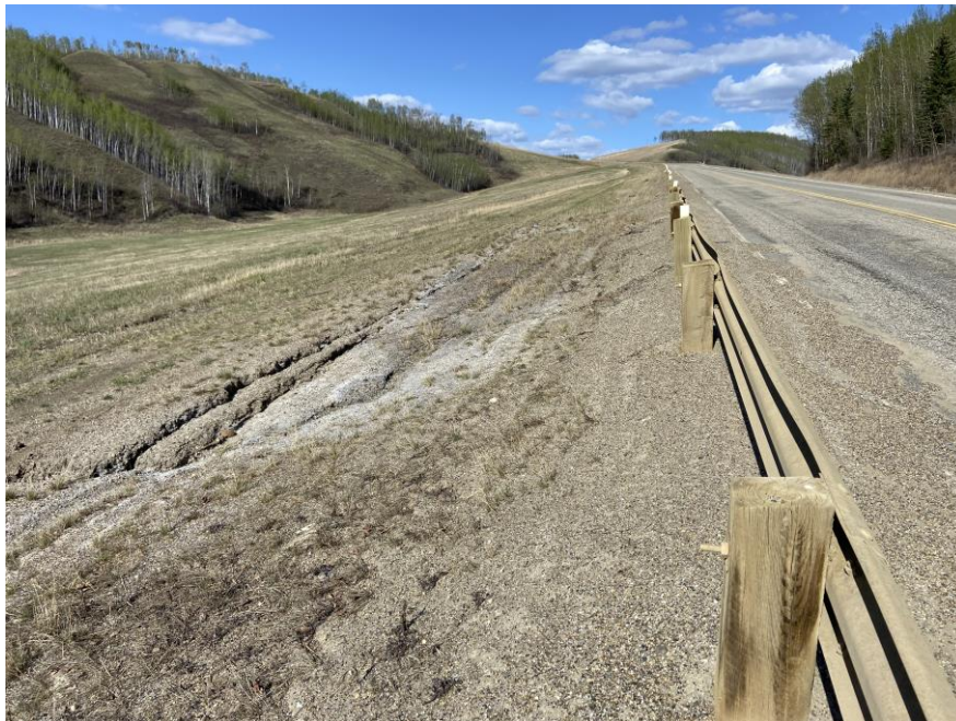
Photo 10 – Looking east at the rilling adjacent to the north guardrail (just west of the repaired rilling on the north embankment).
