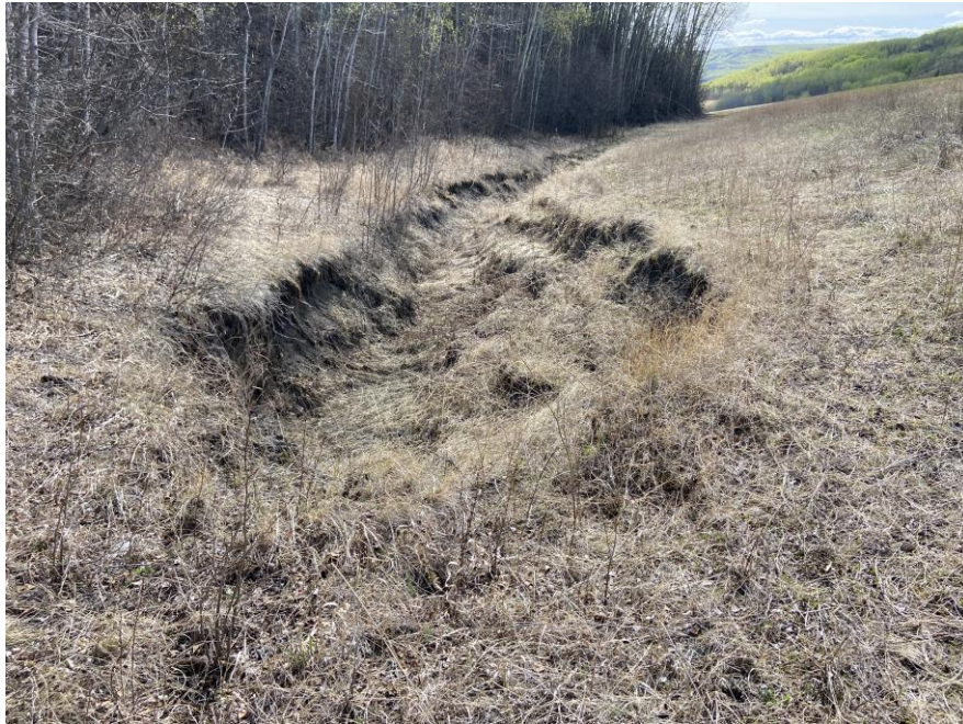
Photo 5 – Looking west at the erosion that formed in 2020 along the boundary of the south embankment fill and the bush line.
