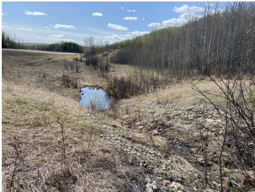
Photo 12 - Looking west (downstream) along the north ditch channel upstream of the 810 CSP outlet. Note the gabions are still intact here.
