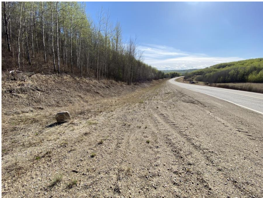
Photo 2 - Looking west along the unlined south highway ditch from the inlet of the 760 mm dia. SWSP.
