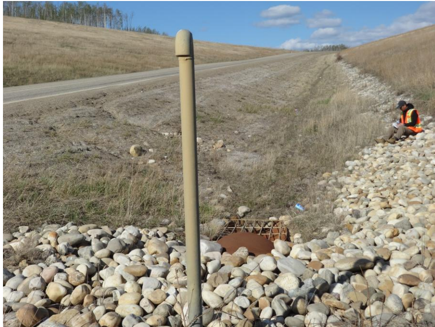
Photo 9 – Looking east along the south gabion-lined ditch from the north 900 mm SWSP entrance.
