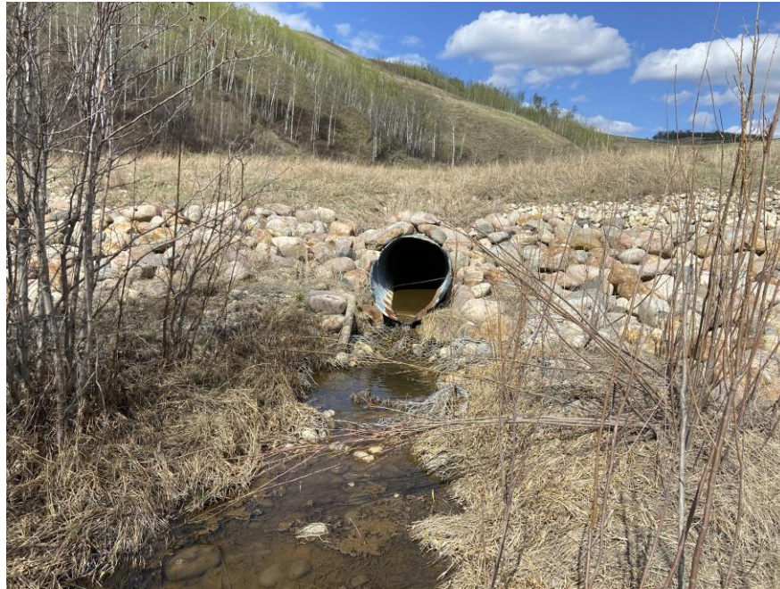
Photo 17 - Looking east at the 1200 CSP outlet area in the north channel. Note the damaged gabions.
