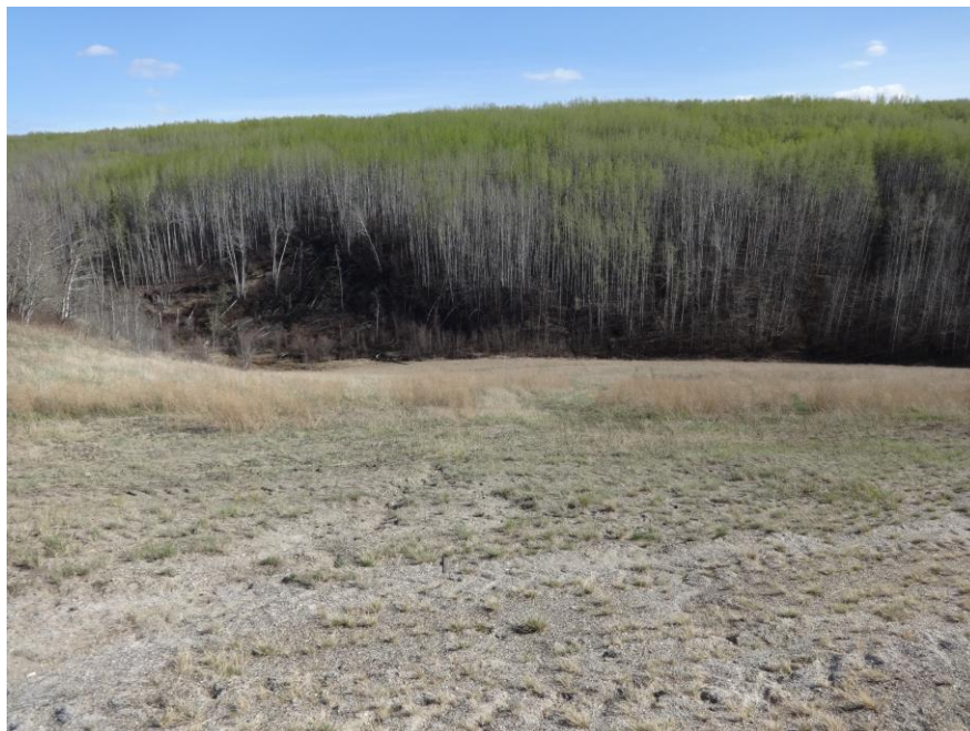
Photo 8 – Looking south at the valley slope slumping above the 1200 culvert inlet and gabion outlet area, caused by rapid drawdown of built-up floodwater.
