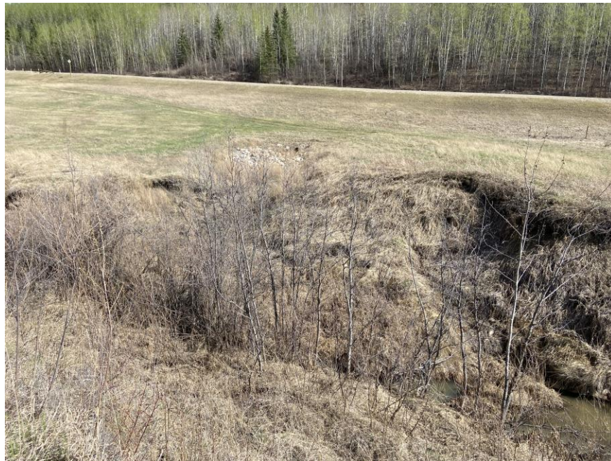
Photo 14 - Looking southeast at the 760 mm SWSP outlet. Note the fresh erosion and associated slumping inside the channel.
