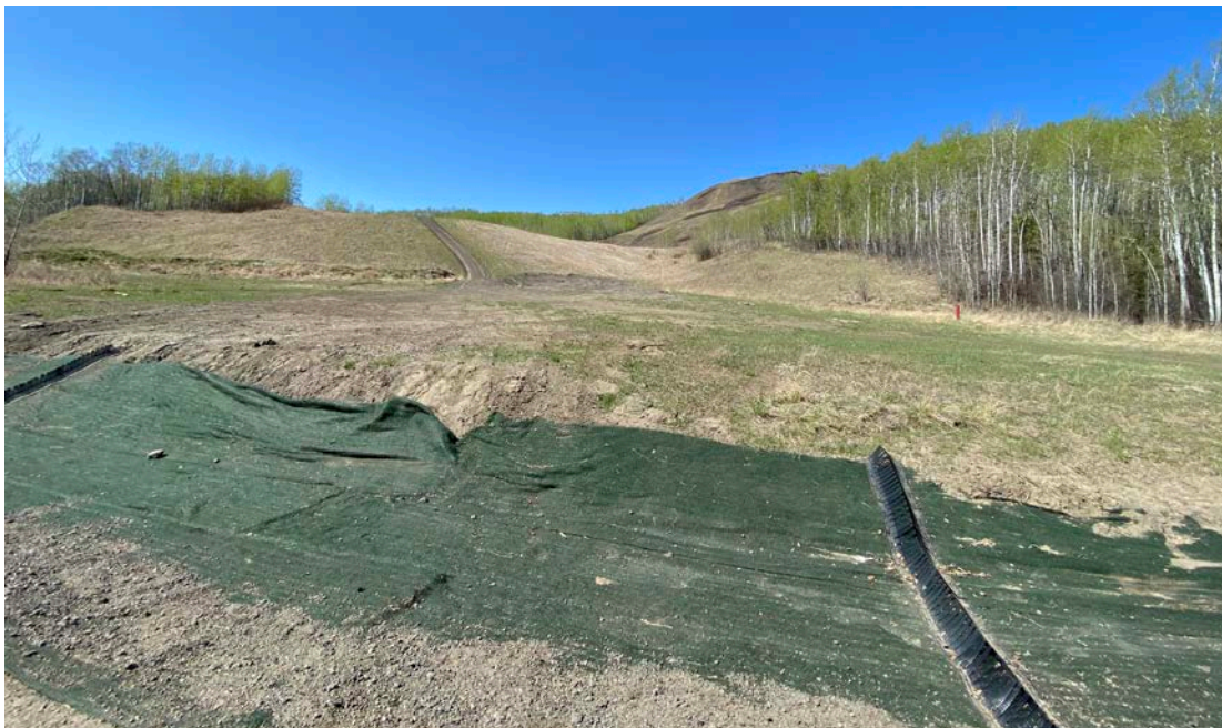
Photo 8 - Looking north across the repaired highway ditch from the former alligator cracked highway area at the east end of the site.
