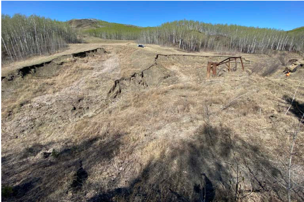
Photo 13 – Looking north across the eroded tributary channel towards the highway, at the eroded piping area (LHS), twin pipe inlets and trash rack (Center), and eroded gabion weir (RHS).
