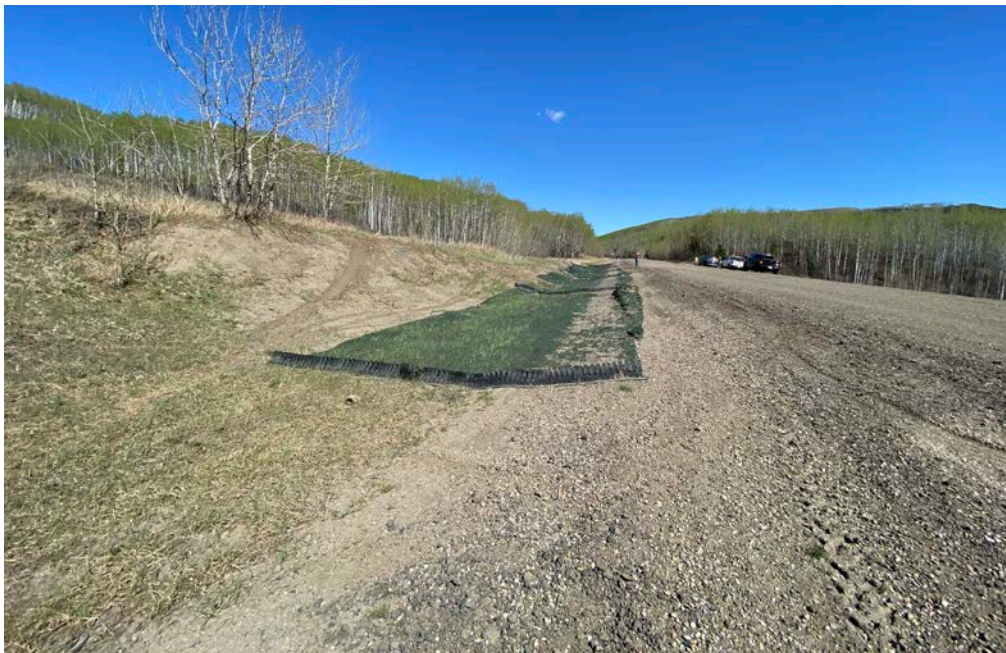
Photo 6 – Looking east along the north ditch that was re-graded and lined with TRM, across the area where the east slide crack was affecting the highway.
