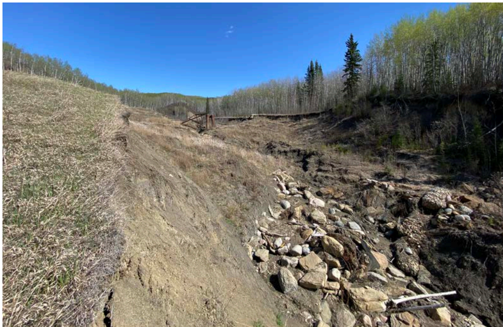
Photo 16 – Looking east along the eroded channel from the site center.
