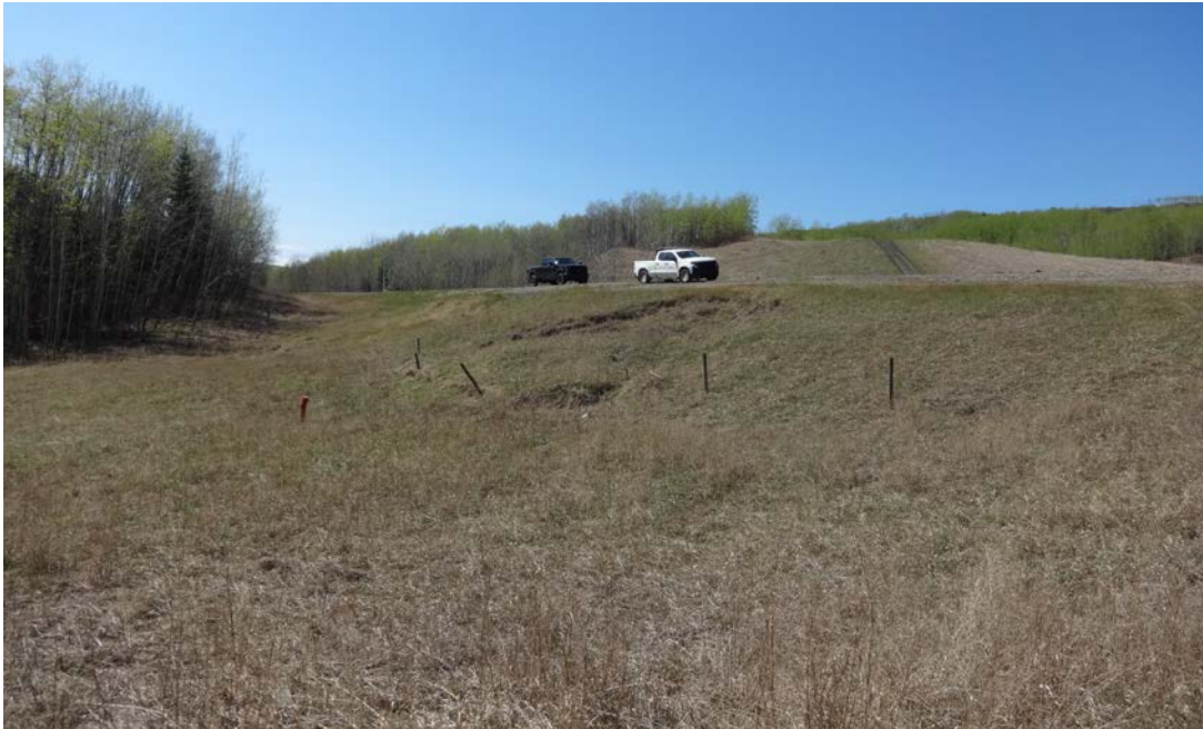
Photo 9 – Looking northwest at the slump in the south highway embankment sideslope.
