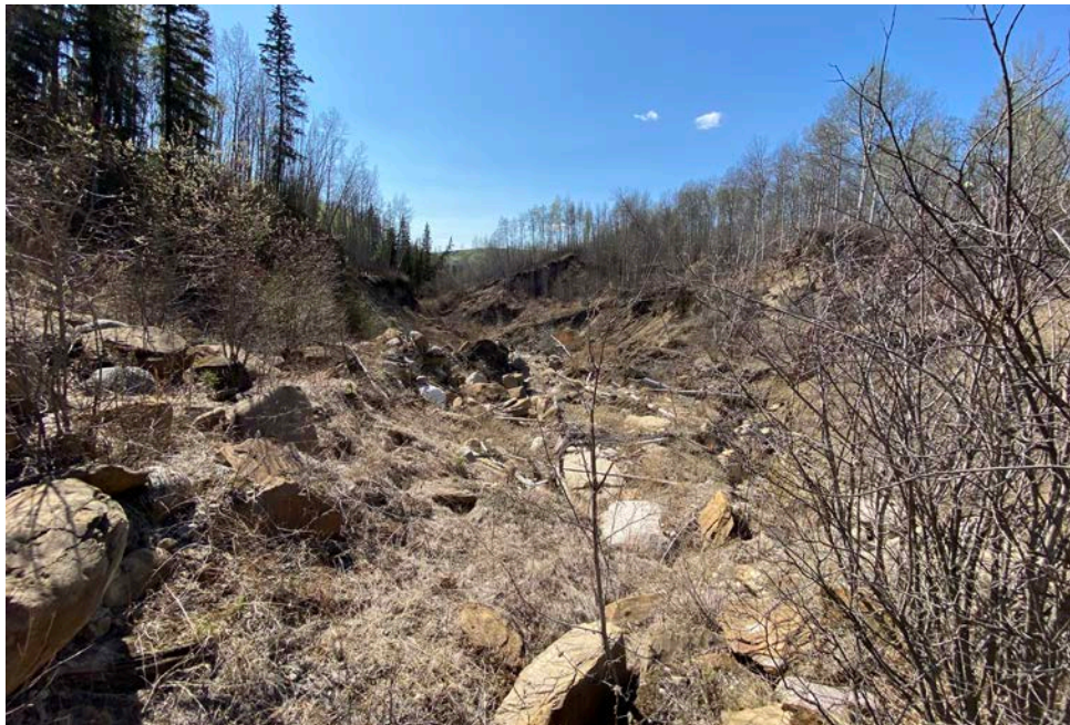
Photo 14 – Looking west along the eroded channel from west of the point where the two tributary branches merge into one.
