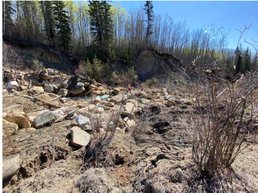
Photo 15 – Looking west along the eroded creek channel at the twin pipe outlets.
