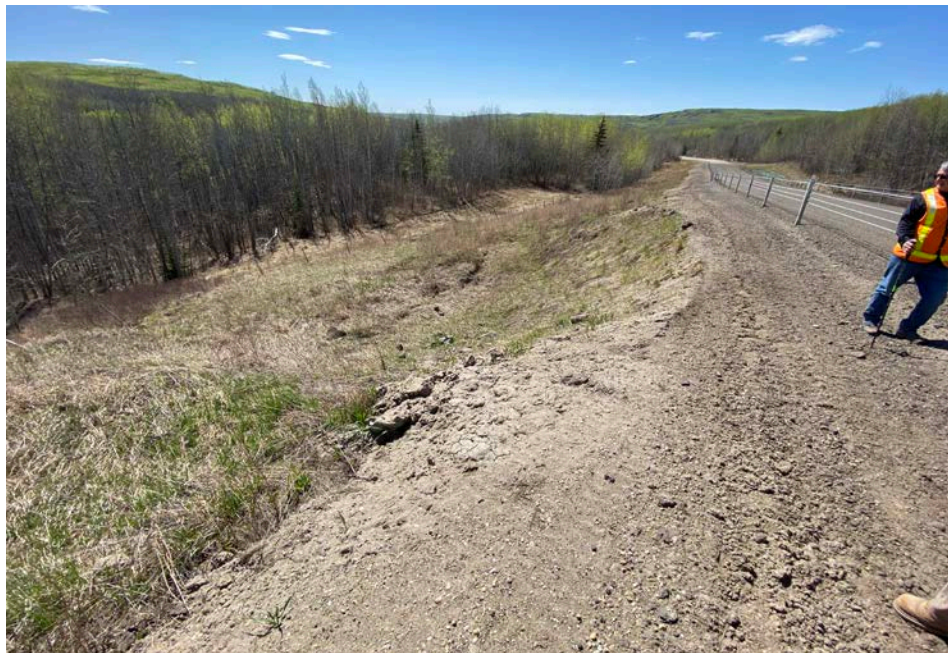
Photo 4 – Looking west at Embankment Slump B on the south side of the hwy.
