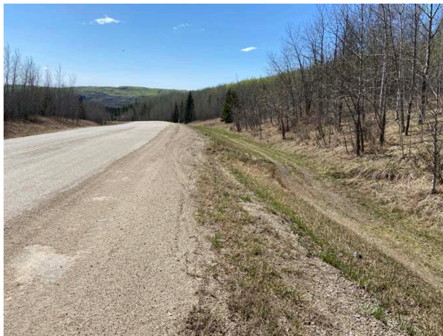
Photo 2 – Looking west at the same slide crack and scarp that extends into the north ditch.
