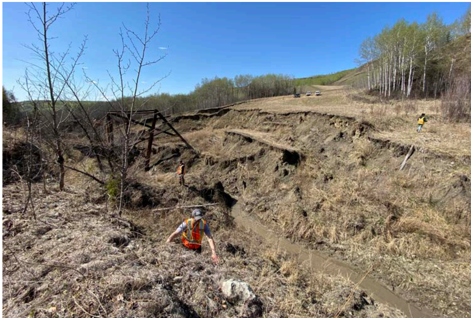
Photo 12 – Looking northwest across the eroded tributary channel and trash rack. Note a fresh slide block has moved about half-way down the north channel slope face.
