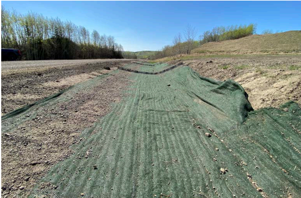
Photo 7 – Looking west along the north highway ditch at the former sagged area that had ponded water. Water was drained, the former north approach was removed and the ditch was graded and lined with TRM as part of the 2023 road surface gravel conversion project.
