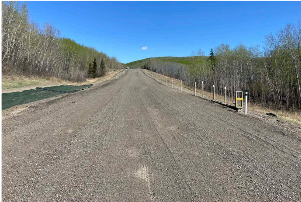
Photo 3 – Looking east at the location where a landslide crack and large dip used to be visible in the road surface before the road surfacing was converted to gravel in 2023. The ditch that had been distorted by landslide movement was also regraded and the ditch lined with TRM.
