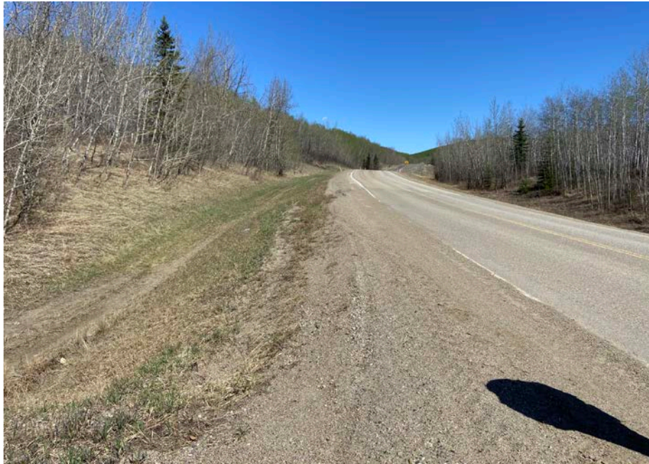
Photo 1 - Looking east at the milled/patched area over the two slide cracks first observed in 2013 that mark the west boundary of the slide on the highway. Note the two settled areas along the north edge of the highway embankment.
