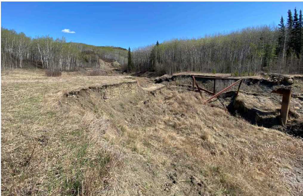
Photo 10 – Looking southeast across the eroded channel at the twin pipe riser inlets and eroded trash rack.
