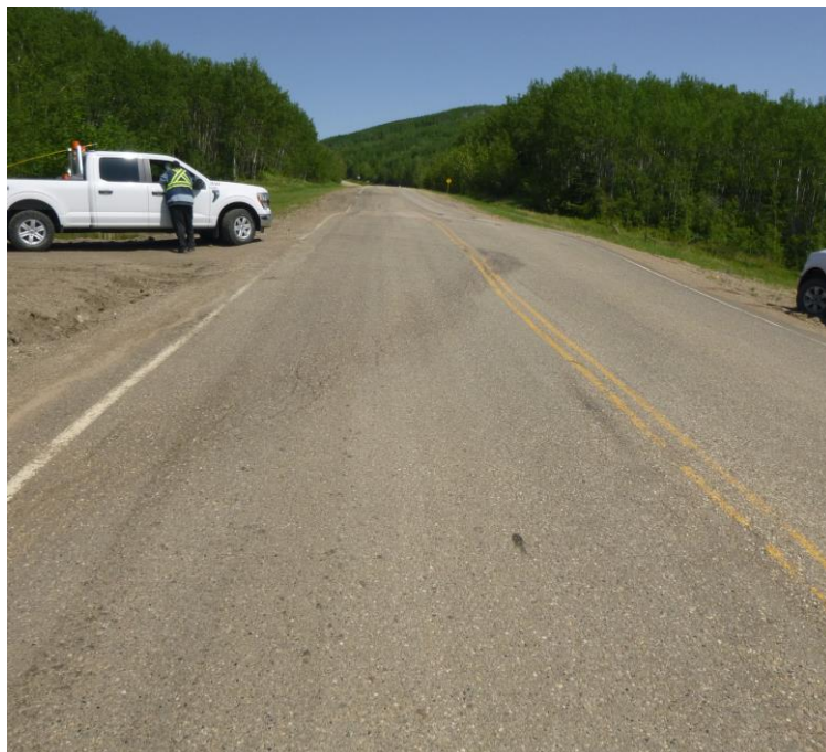
Photo 6 – Looking east at the west milled/patched area over the east slide crack.
