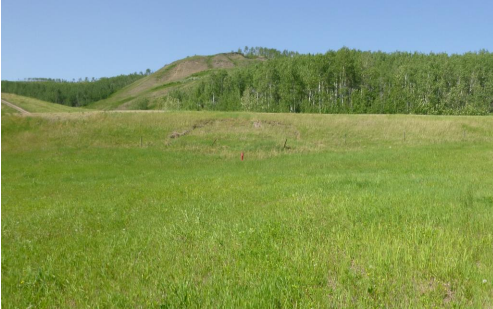
Photo 9 – Looking north at the slump in the south hwy embankment, from the top of the piping area.
