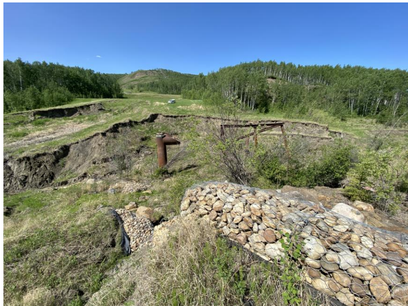
Photo 12 - Looking north across the eroded tributary channel towards the highway, at the eroded piping area (LHS), twin pipe inlets and trash rack (Center), and eroded gabion weir (Foreground).
