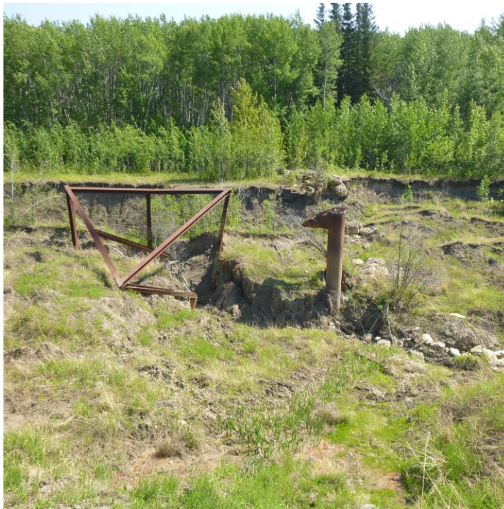
Photo 10 – Looking south across the eroded channel at the twin pipe riser inlets and eroded trash rack.
