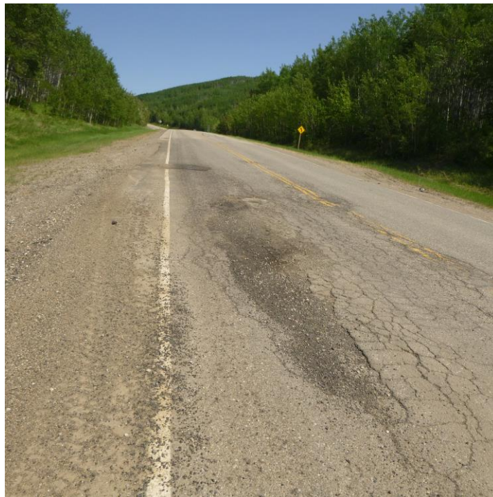
Photo 8 - Looking east along the highway at the alligator cracked hwy area at the east end of the site.
