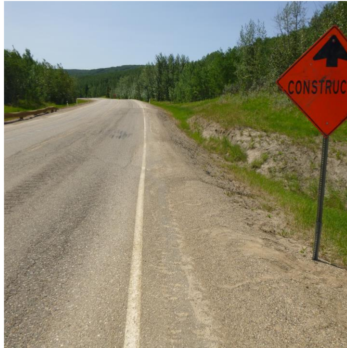
Photo 3 – Looking west from near the west end of the guardrails along the slide scarp that extends along the north highway ditch.
