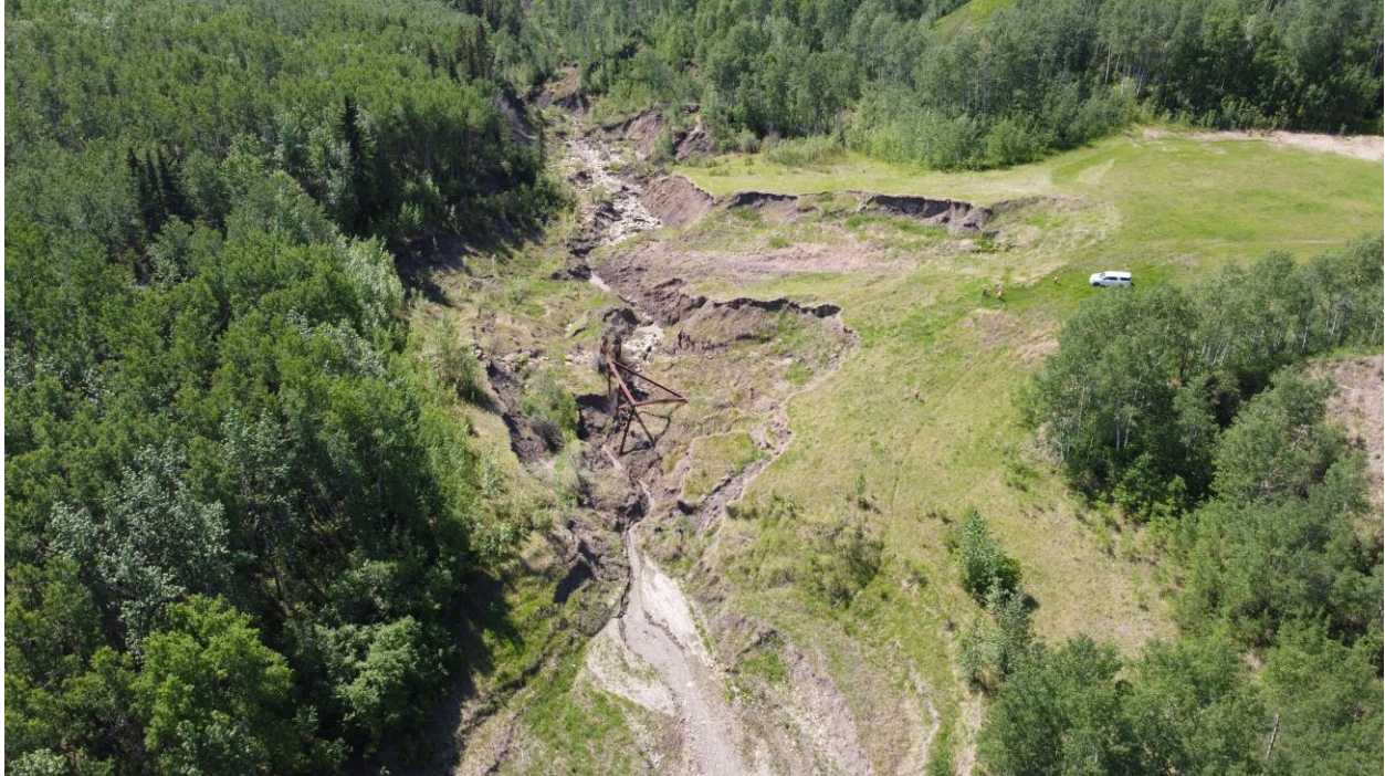
Drone Photo 15 – Looking west along the eroded creek channel at the twin pipe inlet risers, and the eroded trash rack.
