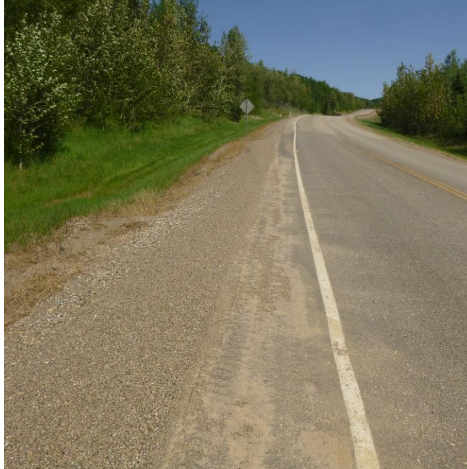
Photo 1 - Looking east along the highway at the milled/patched area over the two cracks first observed in 2013 that mark the west boundary of the slide on the highway. Note the two settled areas along the north edge of the hwy embankment.
