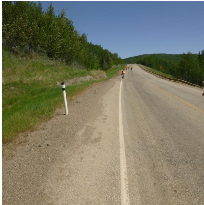
Photo 2 – Looking east along the highway and scarp in the north ditch, and large dip that extends across the highway at this location, near the west end of the site.
