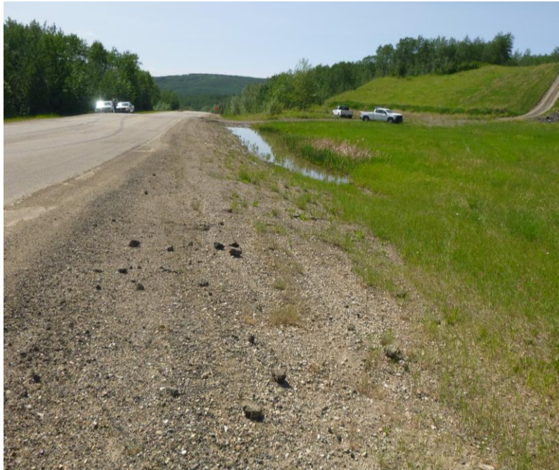
Photo 7 – Looking west along the north highway ditch at the sagged area with ponded water and north approach in the background.
