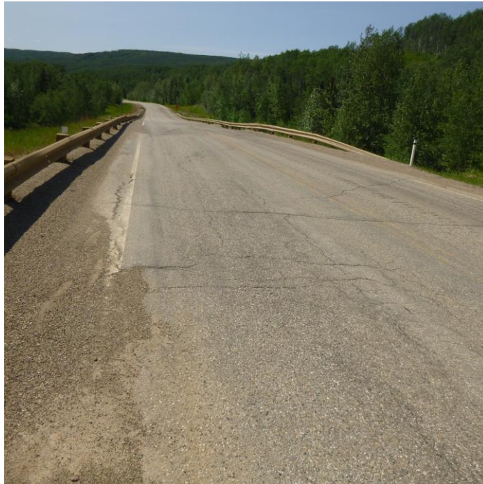
Photo 5 – Looking west along the distorted highway at previous slide cracks east of the northeast guardrail end.
