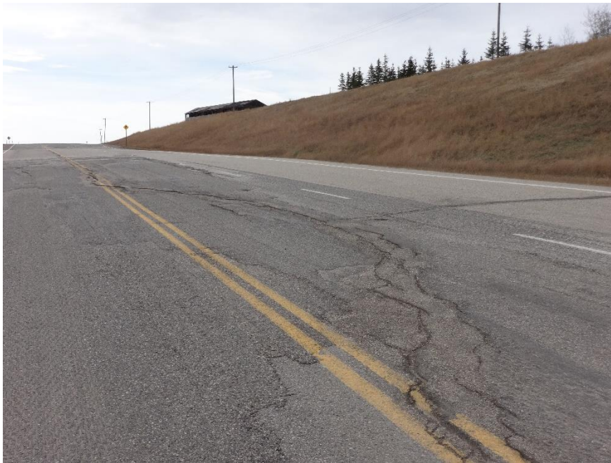
Photo 8. Looking northwest from the middle of Hwy 49:06 from the south end of the 2021 ACP patch. Photo Credit: Nicole Wilder.
