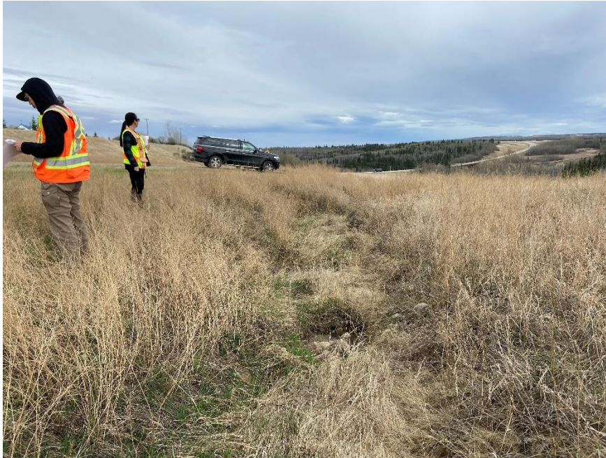
Photo 1. Looking southeast at erosion gully that had formed in the south ditch which had pooling water in it in 2022 but the scour holes were mainly dry with slight moisture in 2024. Photo credit: Don Proudfoot.
