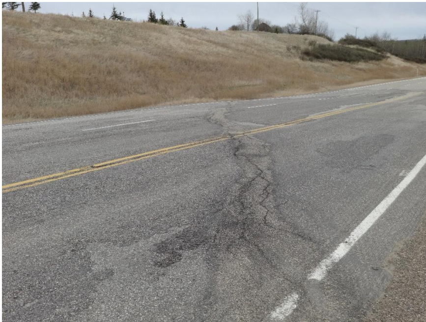
Photo 12. Looking southeast at the northwest end of the site at scarp crack open on the SBL shoulder. Photo Credit: Nicole Wilder.
