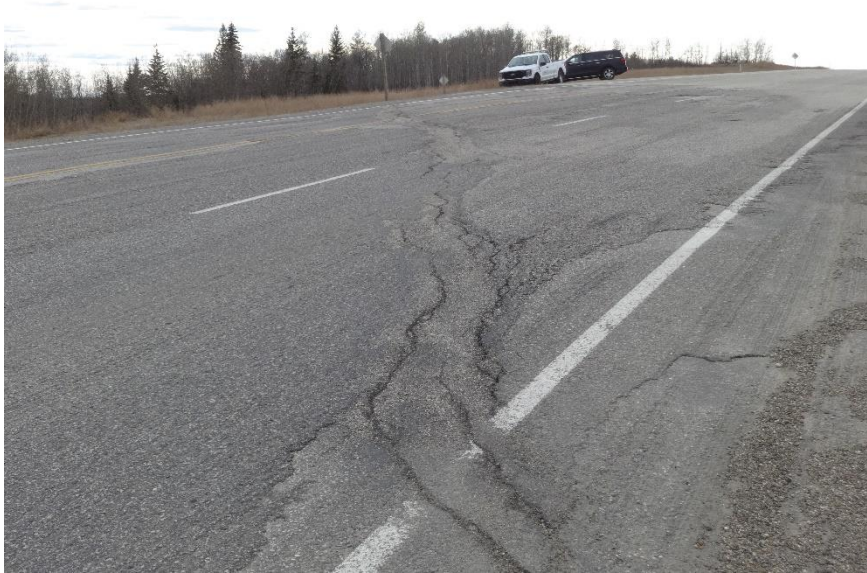
Photo 13. Looking southwest at the northwest end of the site at the scarp crack. Photo Credit: Don Proudfoot.
