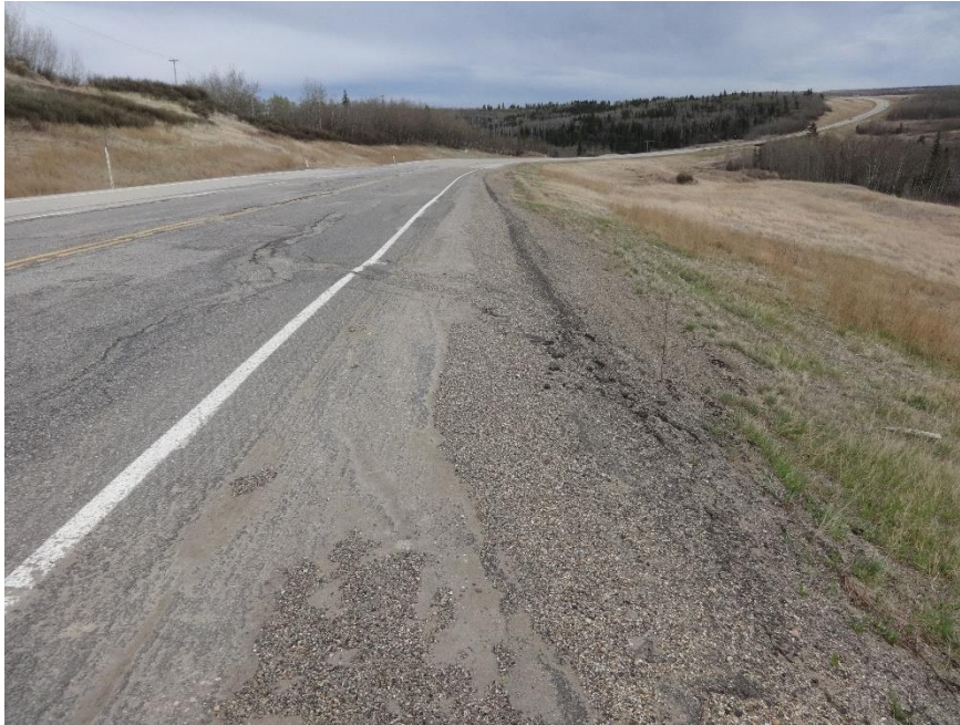
Photo 7. Looking east from the shoulder of the EBL of Hwy 49:06 at the dip in the 2021 ACP patch. Photo Credit: Nicole Wilder.
