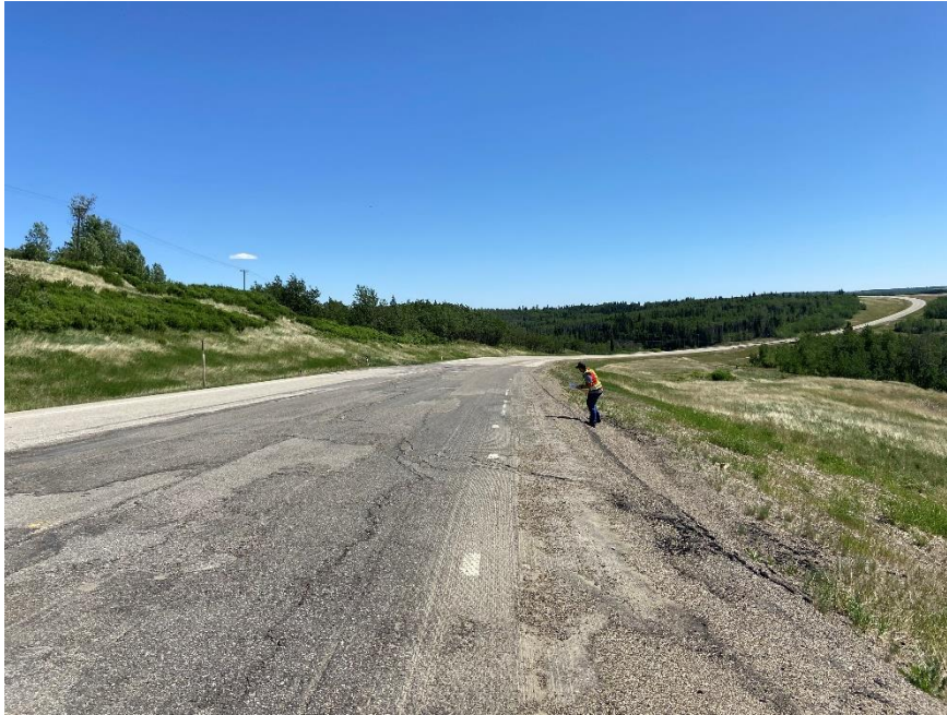
Photo 7. Looking east from the shoulder of the EBL of Hwy 49:06 at the dip in the 2021 ACP patch. Photo Credit: Don Proudfoot.
