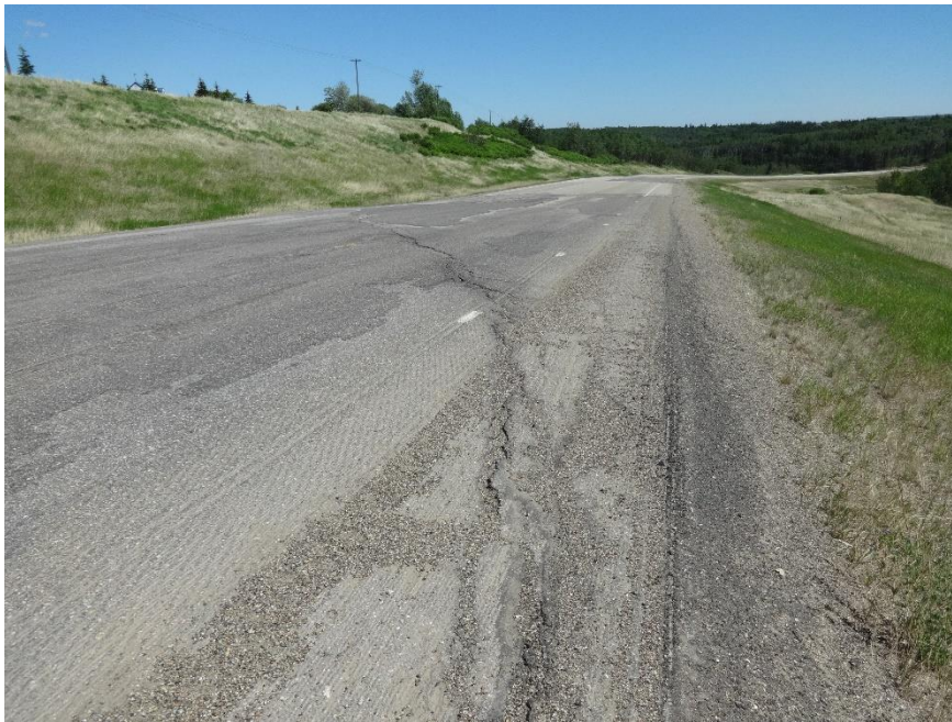
Photo 12. Looking southeast at the northwest end of the site at scarp crack open on the SBL shoulder. Photo Credit: Nicole Wilder.
