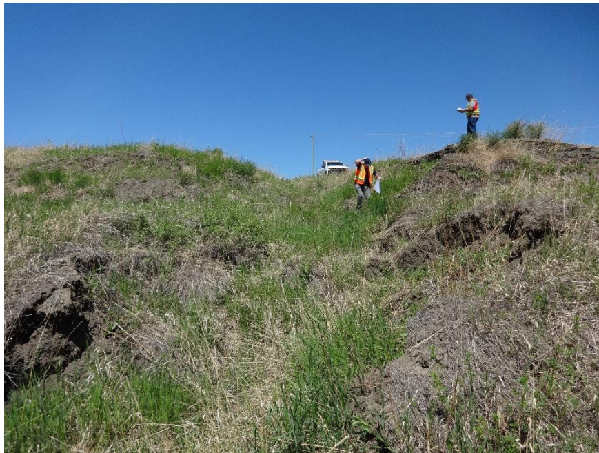
Photo 2. Looking north from edge of erosion gully. Note the ditch along south side of highway tails off and has been the contributor to this erosion. Photo credit: Nicole Wilder.
