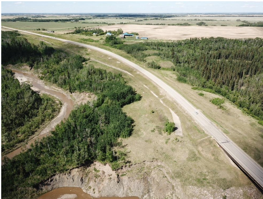
Photo 16. Looking northwest at river and river bank slumping. Photo Credit: Drone- Nicole Wilder. |
