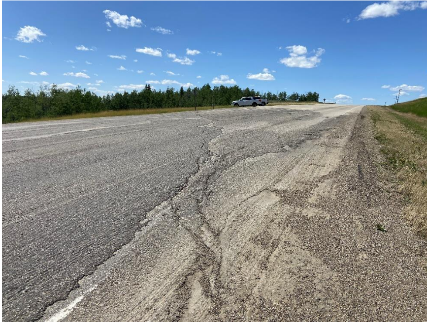
Photo 13. Looking southwest at the northwest end of the site at the scarp crack. Photo Credit: Don Proudfoot.
