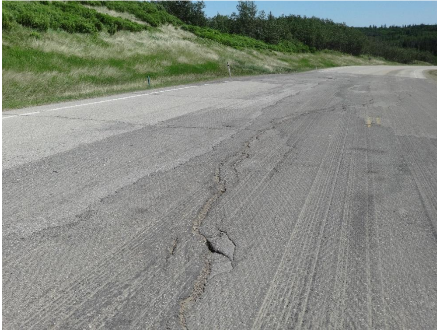
Photo 9. Looking east from near the middle of the 2021 ACP patch where crack continues into WBL. Photo Credit: Nicole Wilder.
