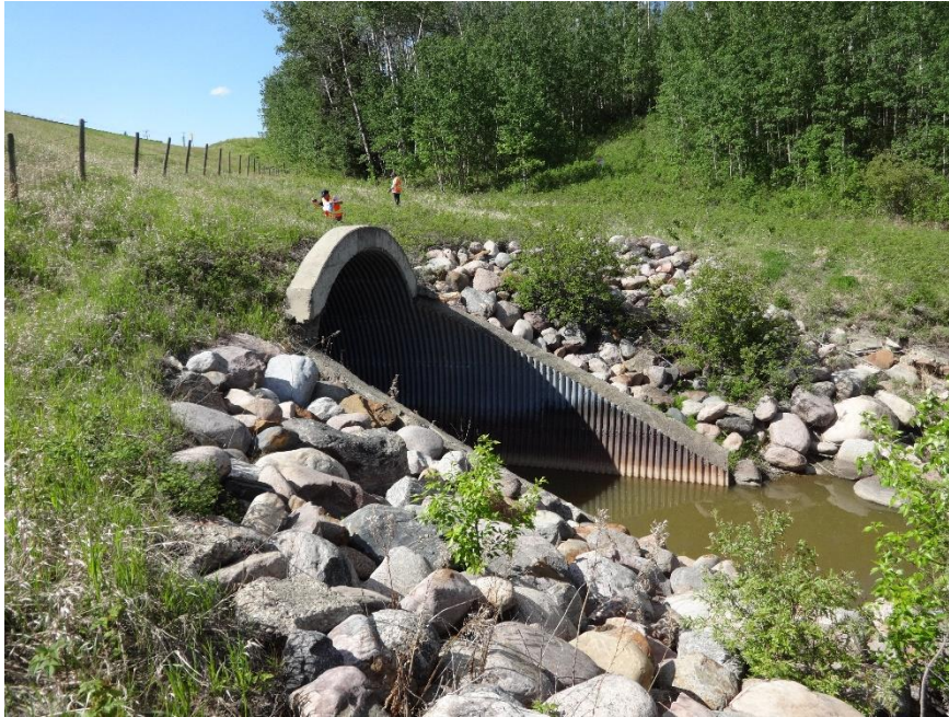
Photo 9. Looking northwest towards the 6.1 m diameter SPCSP centerline culvert outlet. Photo Credit: Nicole Wilder.
