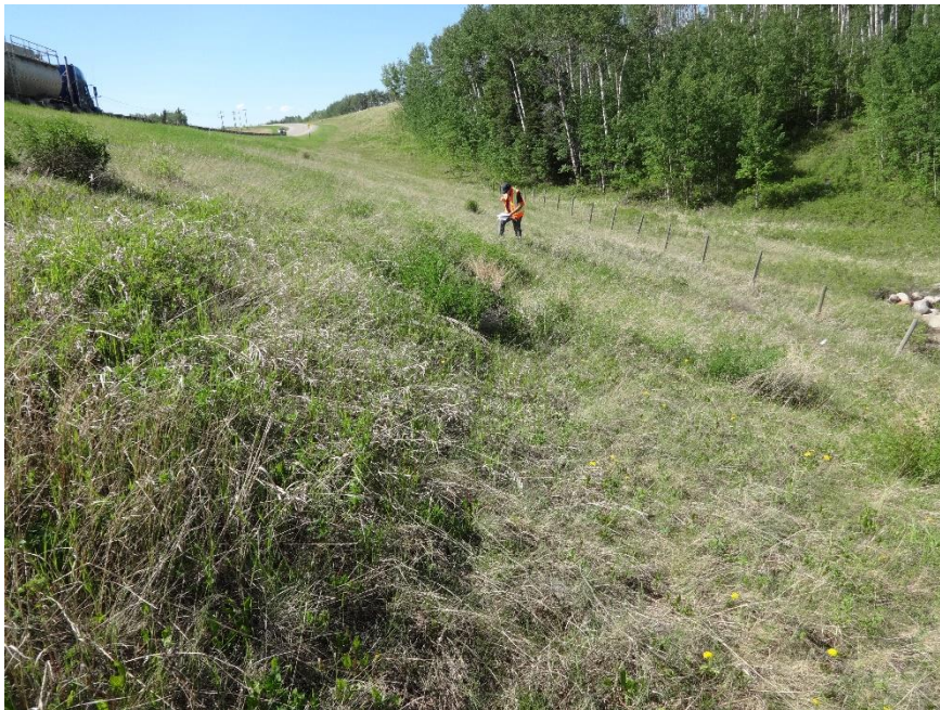
Photo 10. Looking northwest at a scarp crack in the highway sideslope. Photo Credit: Nicole Wilder.
