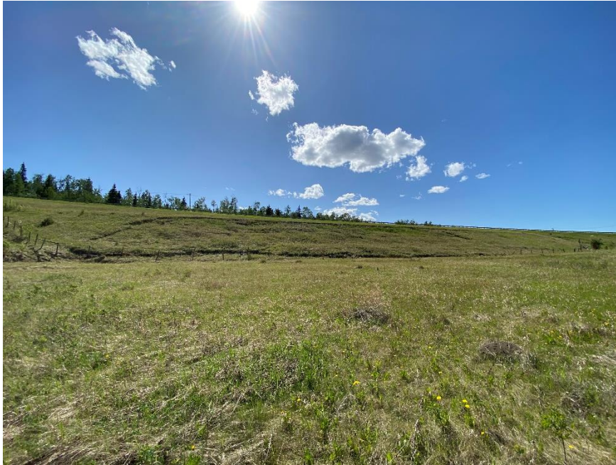
Photo 3. Looking southwest towards the landslide in the toe berm. Photo credit: Don Proudfoot.
