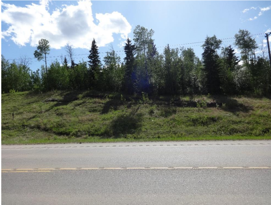
Photo 1. Looking southwest at backslope failure on other side of highway. Photo credit: Nicole Wilder.
