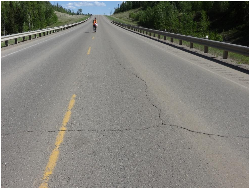
Photo 2. Looking southeast from the southeast bound lane at cracking in pavement. Photo credit: Nicole Wilder.
