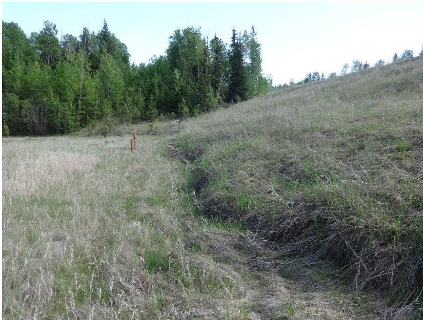
Photo 6. Looking at the toe bulge and bent over posts. Photo Credit: Nicole Wilder.
