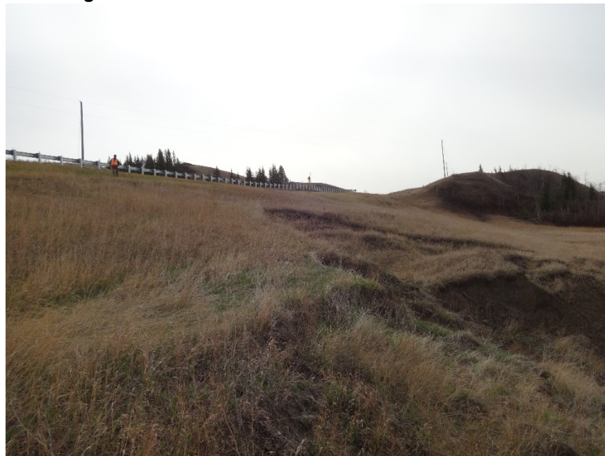
Photo 8. Looking southeast up at the backscarp and flank of the landslide. Photo Credit: Don Proudfoot.
