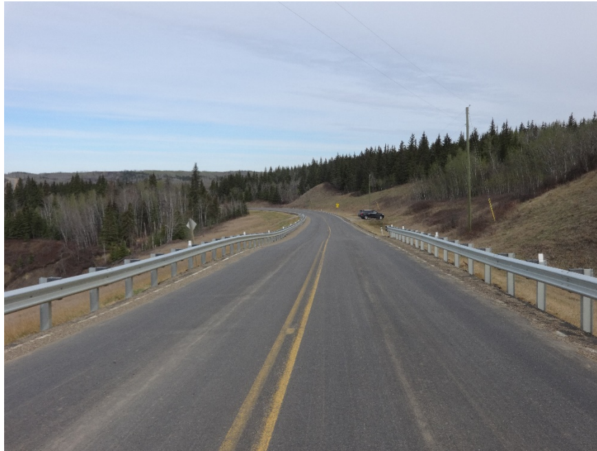
Photo 1. Looking west along the highway at where the highway was overlaid, note the dip in the guardrail. Photo credit: Don Proudfoot.
