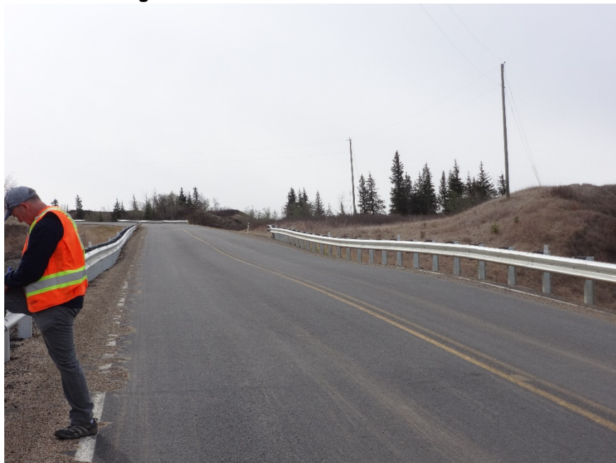
Photo 2. View of where the slide scarp crack was located looking east along the highway from near the west end of the north guardrail. Photo credit: Nicole Wilder.
