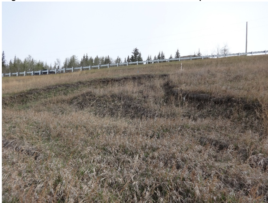
Photo 6. Looking north at slumping above the old culvert alignment on the south highway embankment. Photo Credit: Don Proudfoot.
