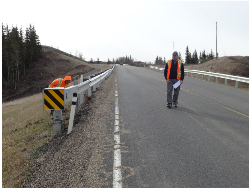
Photo 3. Looking east along the highway at the west end of where the scarp crack was located but was overlayed. Photo credit: Nicole Wilder.
