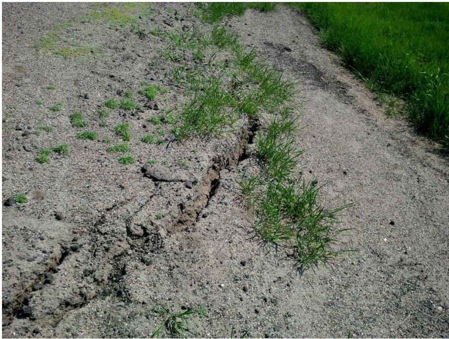
Photo 4. Looking northeast at cracks from backscarp extending through the highway embankment shoulder. Cracks at the shoulder are open to about 60 mm in width.
