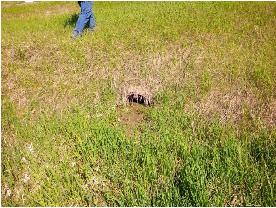
Photo 9. Looking north at the outlet of the existing centerline culvert. The outlet is partially obstructed. No significant change since May 12, 2015.
