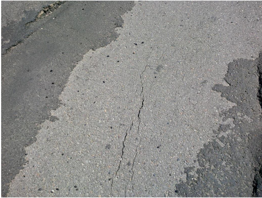
Photo 3. Hairline tension cracks have appeared within the asphalt pavement within the graben.
