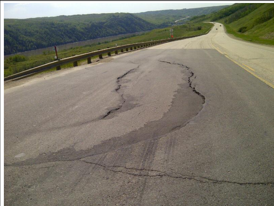
Photo 2. Looking SW from the NBL. The drop of the graben is at about 80 mm with cracks open to about 60 mm in width.
