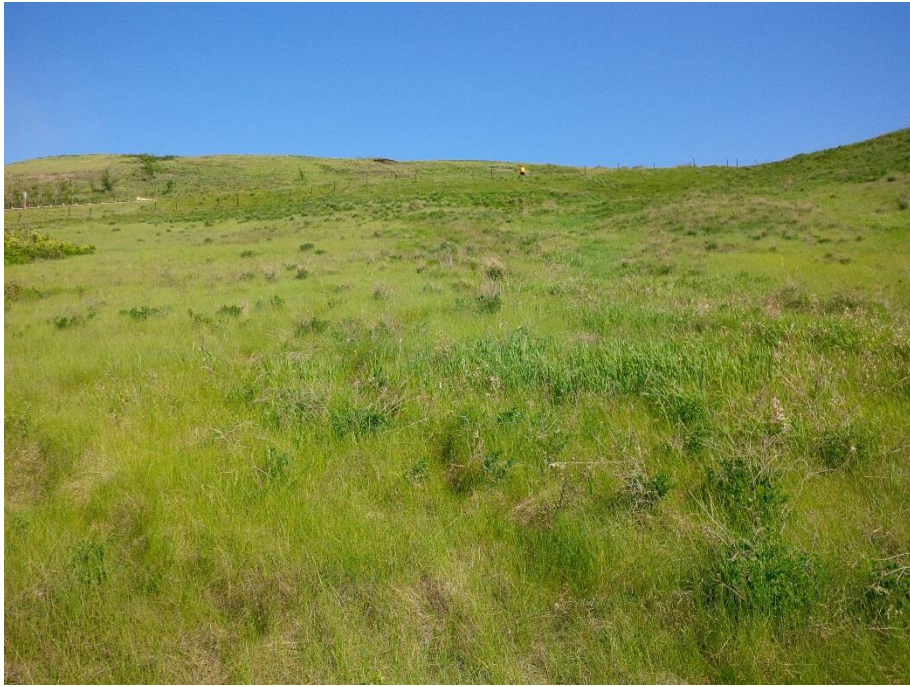
Photo 5. Looking north at the highway sideslope. Two lobe-shaped features were noted below highway with greener vegetation growing along the lower perimeter. This is likely a sign of water seepage. Ripples with tension cracks are visible in the surface at the base of the lobes and clay is exposed though the grass. No significant change since May 12, 2015.
