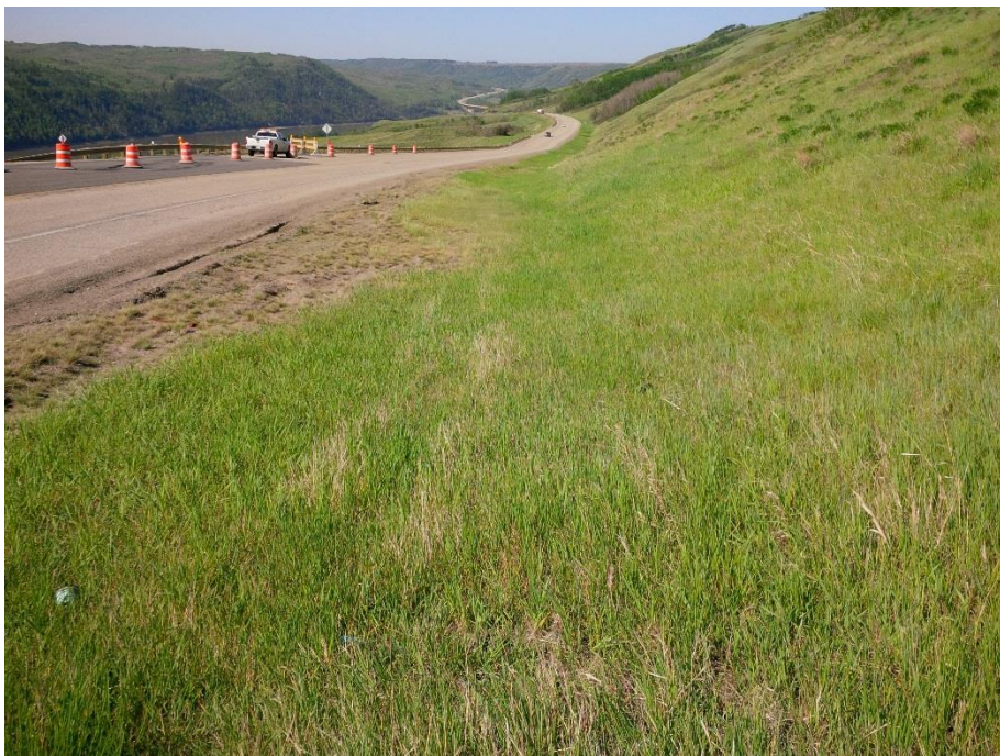
Photo 8. Looking southwest along the SBL lane ditch. Sediment is accumulated along the shoulder downslope of the ditch block at the culvert inlet. Highway embankment material is rilled, moist and soft.
