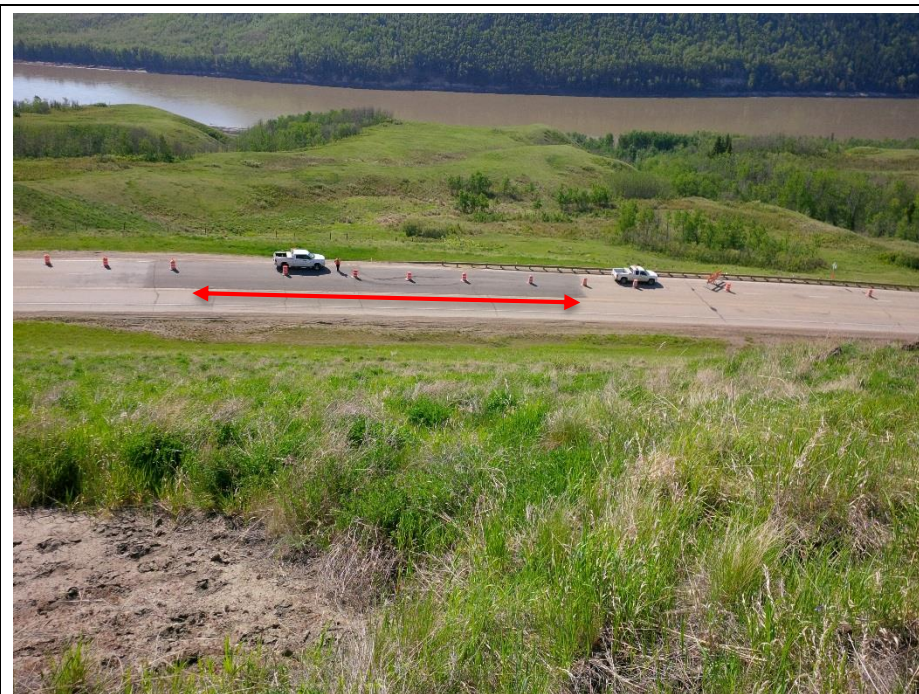
Photo 1. Looking south across the highway from the SBL backslope. Cracks in the pavement surface and along the edge of the guardrail are visible along a 28 m length. TRANS has closed the outer NBL lane due to the drop in the graben.
