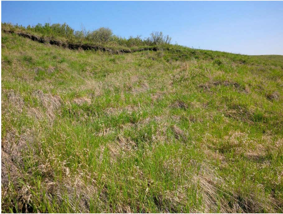
Photo 11. Looking north at large backscarps forming at the crest of the valley slope.
