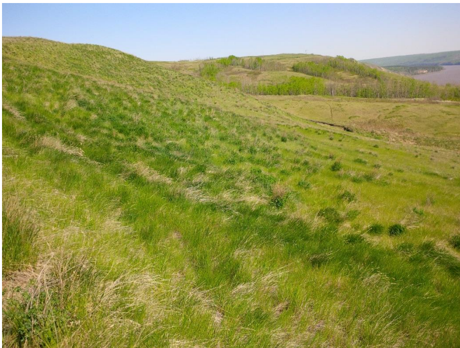
Photo 6. Looking east across the toe bulge feature along the NBL sideslope. Tension cracks with exposed clay are predominant in the lower half of the bulge.
