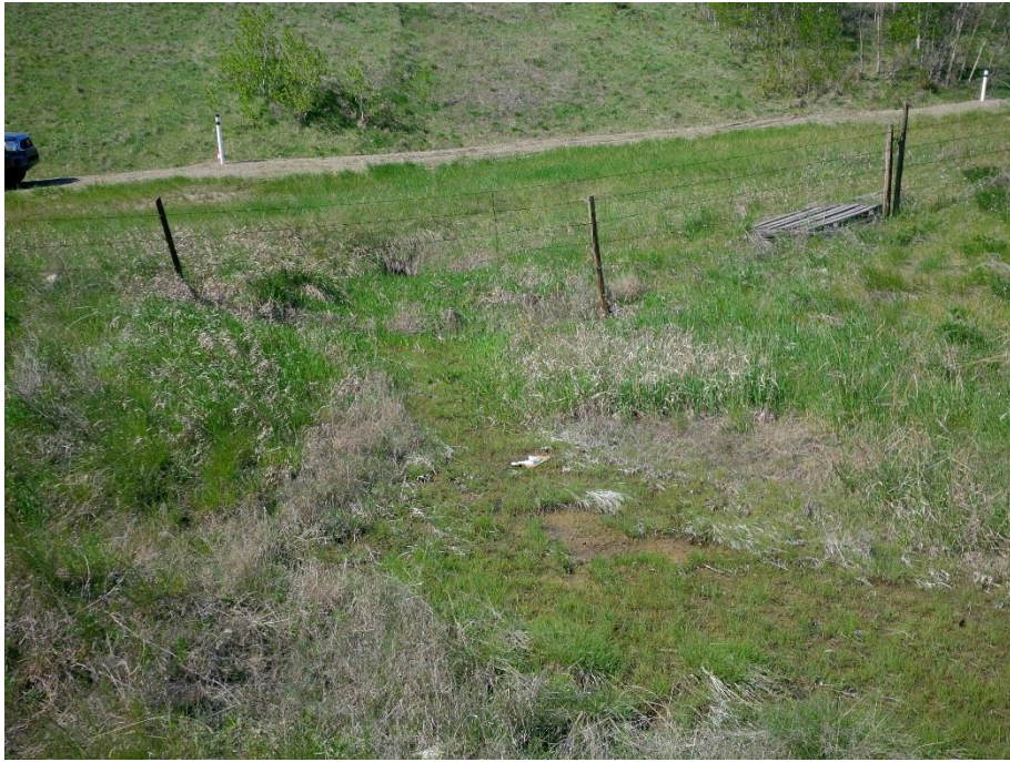
Photo 9. Looking north at the outlet of the existing centerline culvert. The outlet is partially obstructed.
