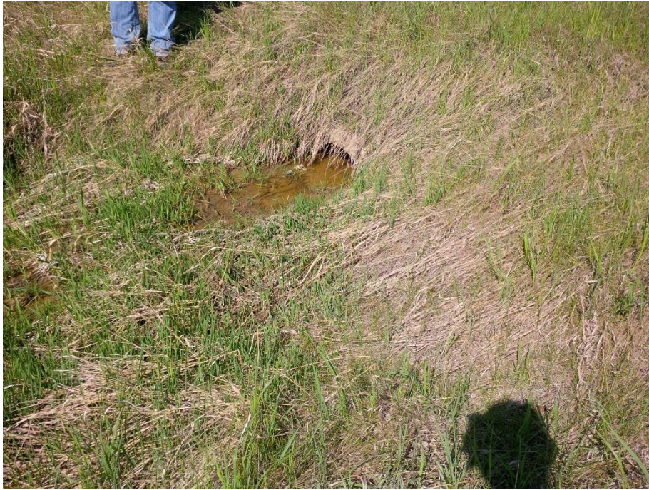
Photo 7. Looking east at the inlet to the centerline culvert. The inlet is over half filled with sediment.
