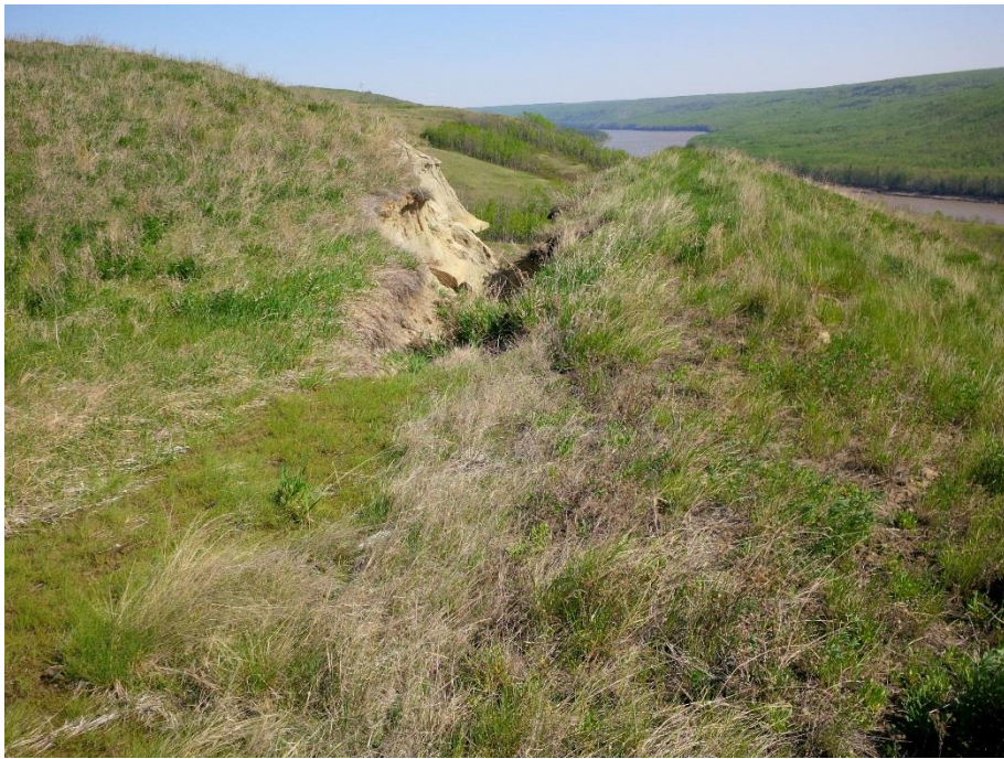
Photo 10. There is ongoing erosion in the gully downstream, with steep gully sidewalls in the bedrock. The backscarp of the gully has not retrogressed since 2014.
