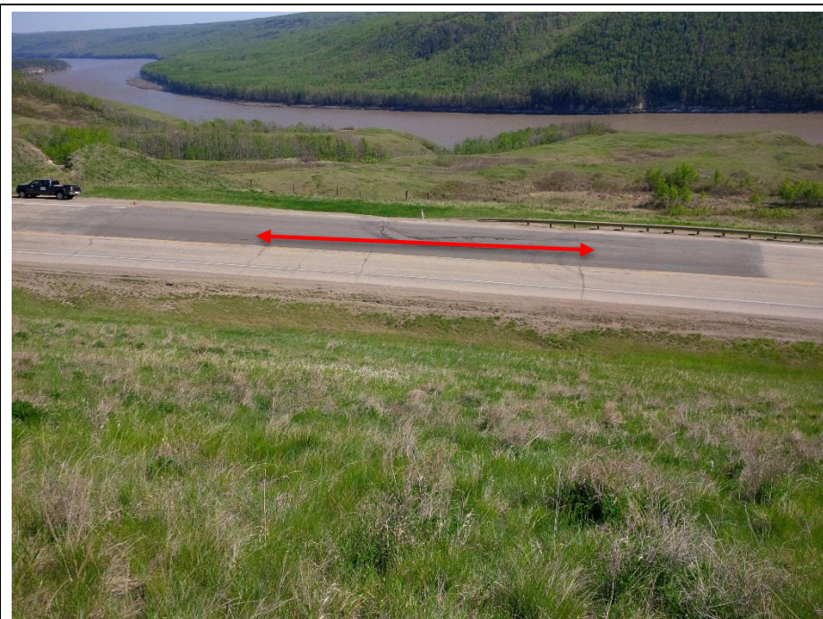
Photo 1. Looking south across the highway from the SBL backslope. Cracks in the pavement surface and along the edge of the guardrail are visible along a 28 m length.
