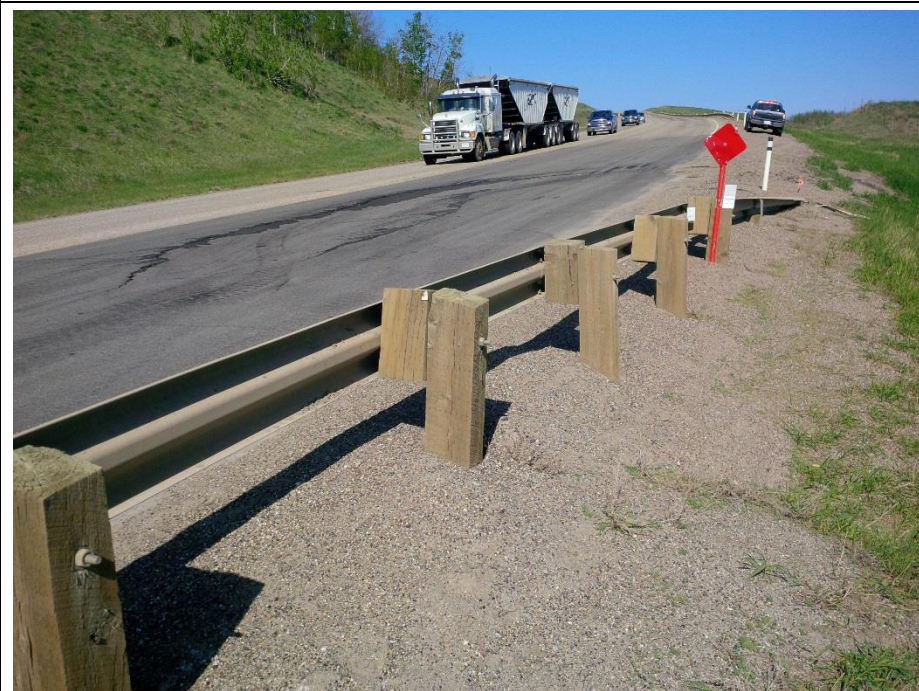
Photo 2. Looking NE from the NBL guardrail. The drop of the graben within the landslide is at about 50 mm with cracks open to about 50 mm in width.
