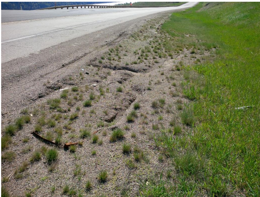
Photo 8. Looking southwest along the SBL lane ditch. Sediment is accumulated along the shoulder downslope of the ditch block at the culvert inlet. Highway embankment material is rilled, moist and soft.
