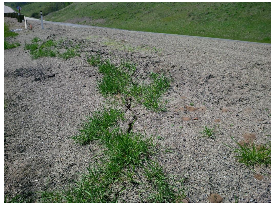
Photo 4. Looking west from the NBL shoulder. Cracking in the embankment shoulder extends 10 m to the east of the dip in the asphalt. Cracks in embankment shoulder extend about 8 m northeast past the edge of the paved shoulder in the sideslope with offset drops up to 150 mm and are open to about 75 mm.
