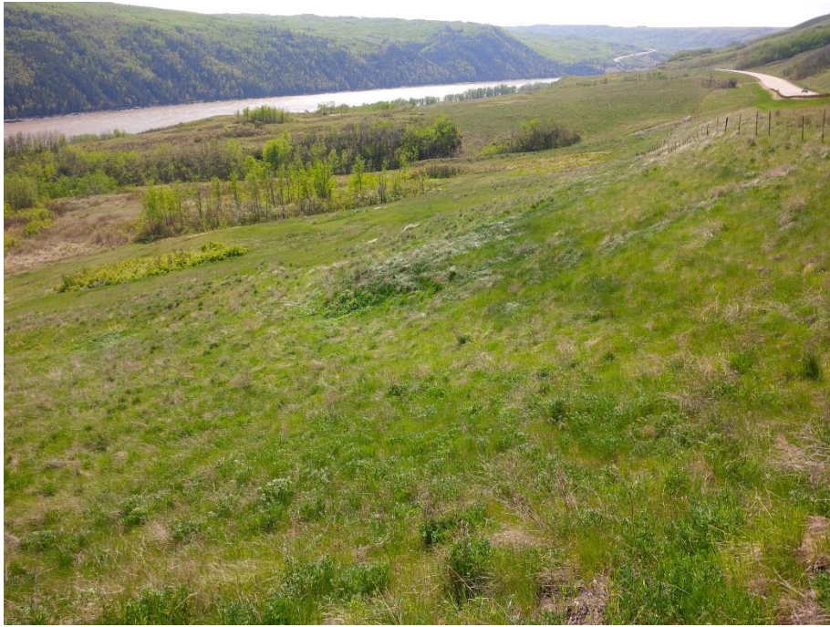
Photo 5. Looking south-westwards at the highway sideslope. Two lobe-shaped features were noted below highway with greener vegetation growing along the lower perimeter. This is likely a sign of water seepage. Ripples with tension cracks are visible in the surface at the base of the lobes and clay is exposed though the grass.
