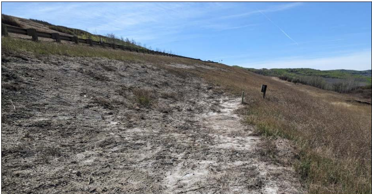
Photo 10: Looking south near Sta. 1+560 at rough area (drill access bench) with some seepage and tension cracks
