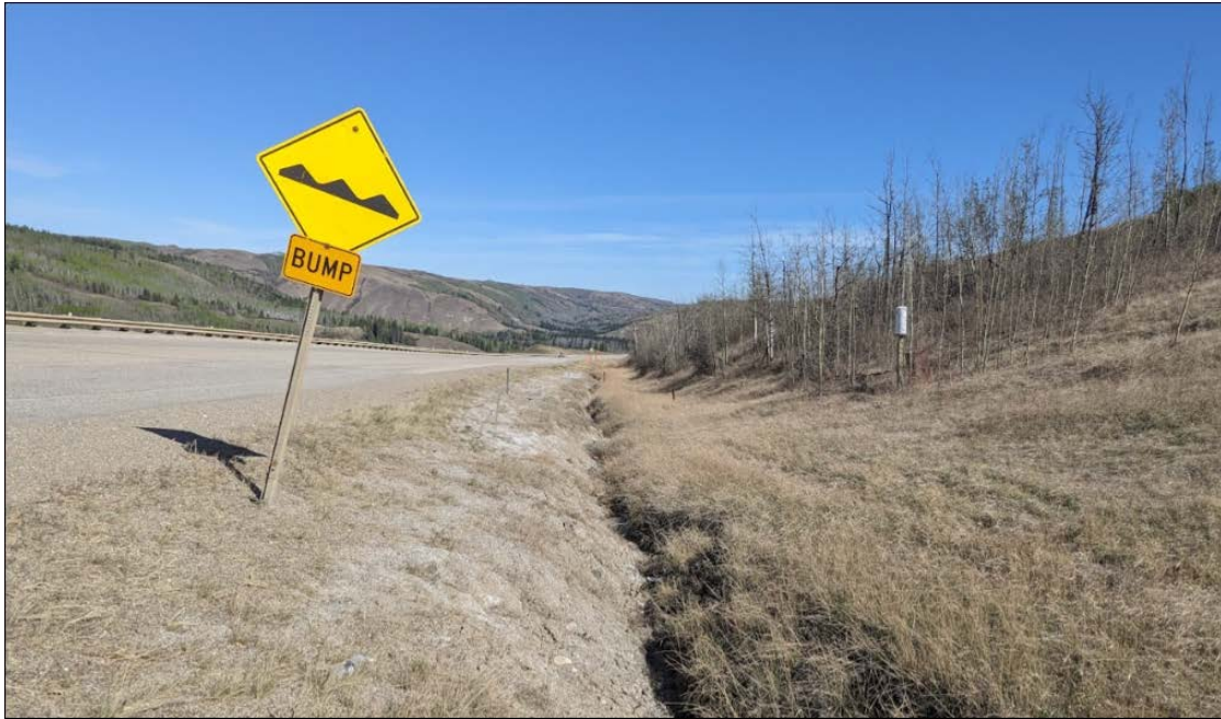
Photo 5: Looking north from Sta. 1+800 at the erosion gully developed on the ditch up to 1.7 m wide and 0.7 m deep.
