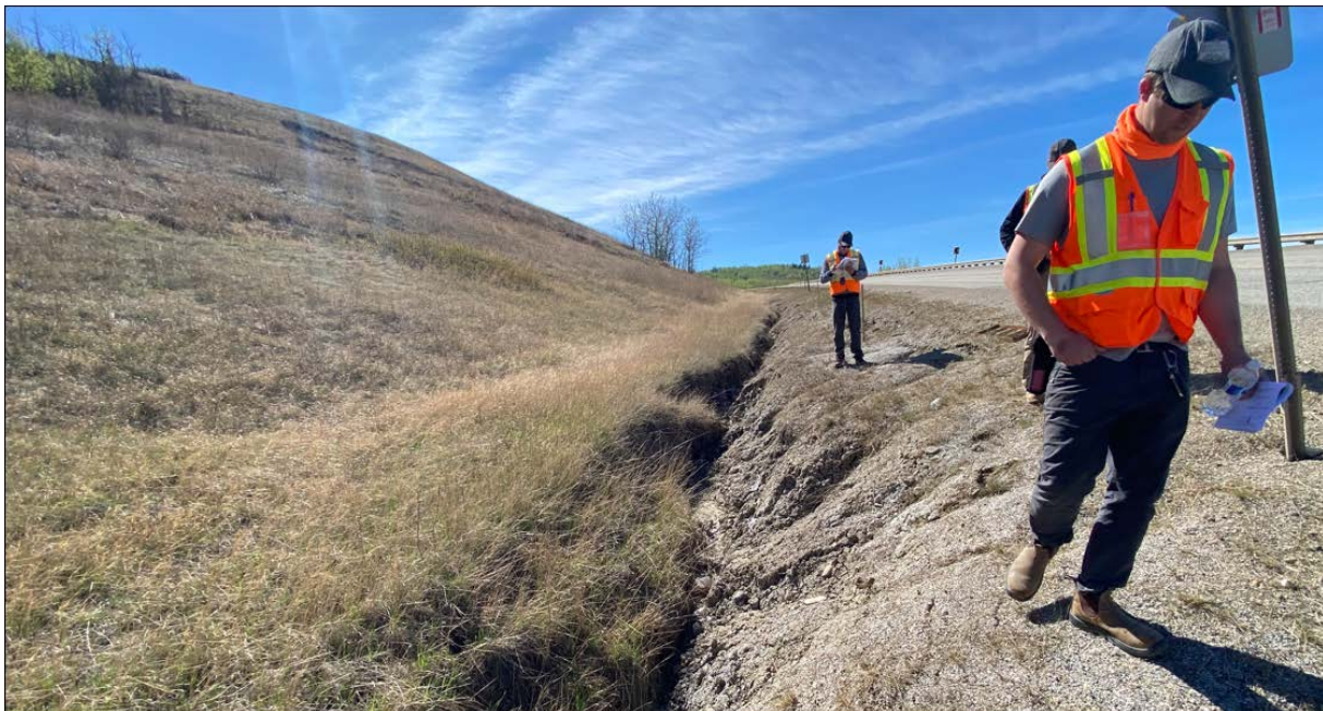
Photo 6: Looking south across the dip in the highway at the south end of the 1+800 slide.
