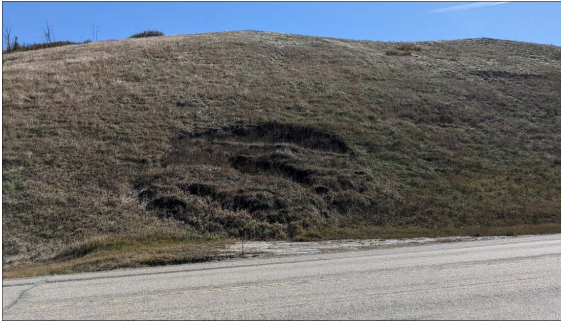
Photo 3: Looking east at backslope skin failure at Sta. 1+950
