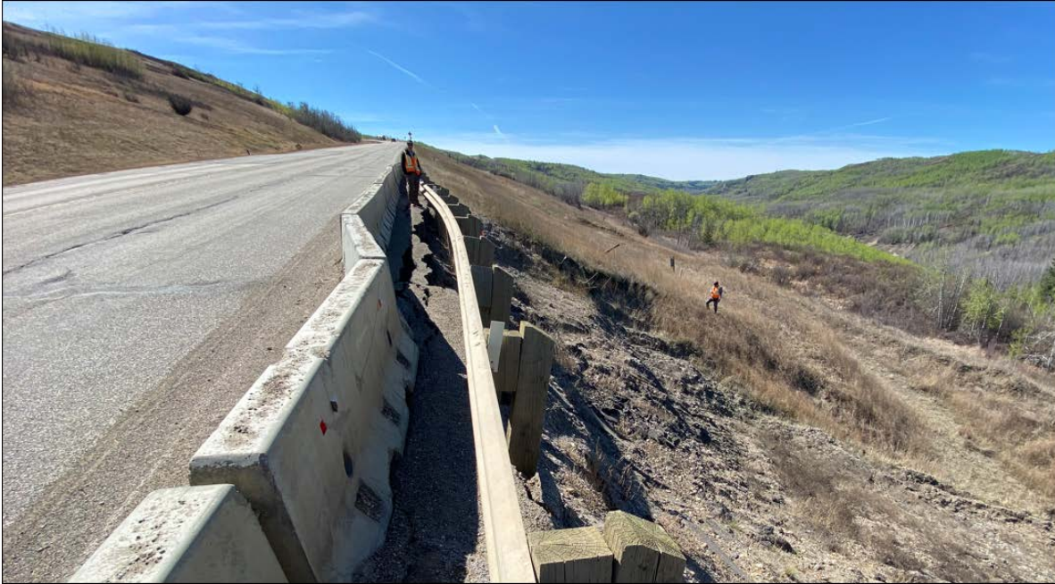
Photo 13: Looking south from Sta. 1+390 at the backscarp of the 1+400 slide which is impacting the highway shoulder. Slide cracks are wider and closer to the driving lane
