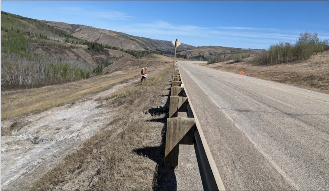
Photo 9: Looking north near Sta. 1+550 at fresh erosion rills and gullies developed on the highway side slope. Erosion became worse in 2023
