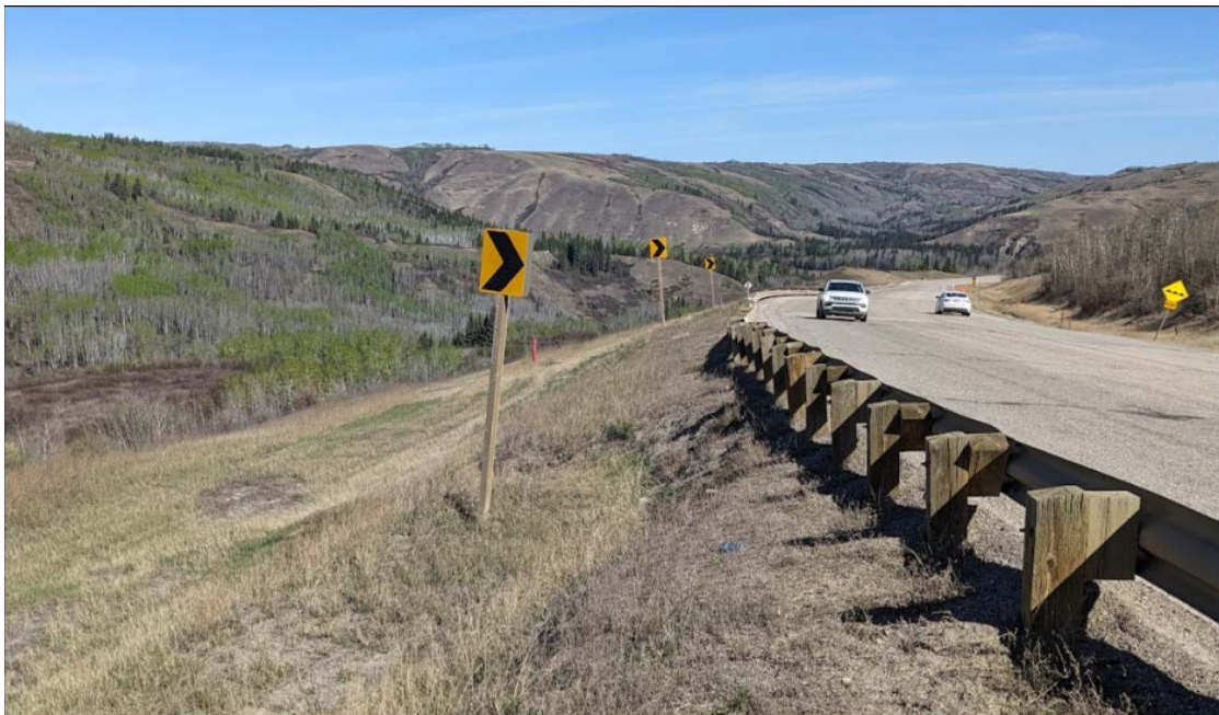
Photo 4: Looking north from Sta. 1+890 at the slump in the sideslope of the SBL. More movement since 2023. The scarp is 1.5 m high and 0.8 m from the guardrail.
