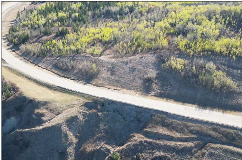
Photo 18: Oblique Drone Photo looking at overall site showing slide at Station 1+400
