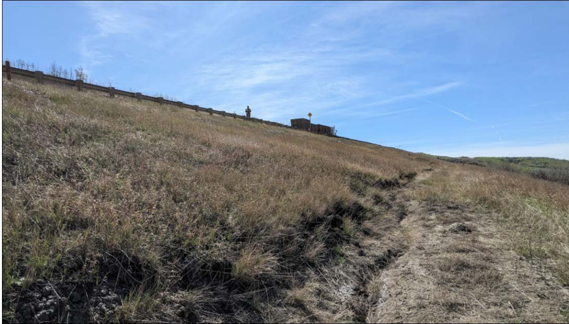
Photo 15: Looking south at slumping occurring from Sta. 1+450 to 1+550. Photo showing a drop of about 0.3 m
