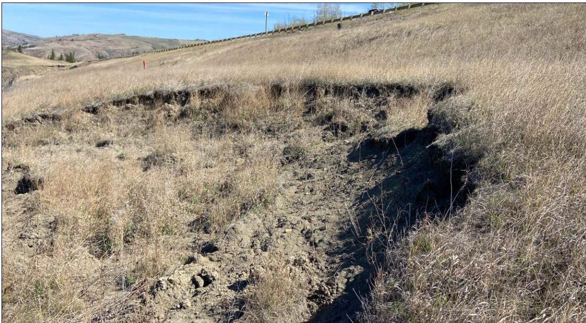
Photo 8: Looking north near Sta. 1+670 at slumping occurring on the highway side slope approximately 20 m from the edge of pavement. More movement noted since 2022
