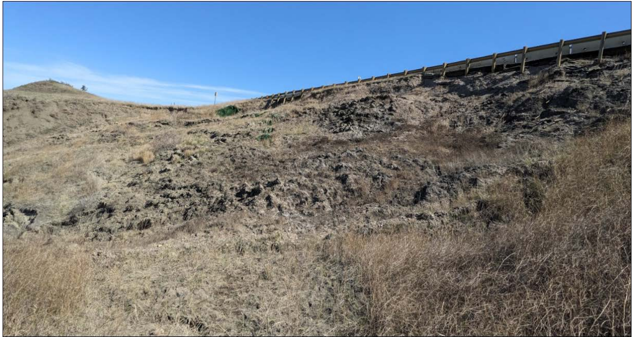
Photo 11: Looking east at failed soil matting and nails which were installed in August 2010 at Sta. 1+450 slide. Backscarp (5 m to 7.5 m high) continues retrogressing and impacting the highway.
