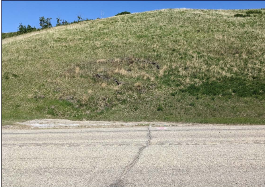
Photo 3: Looking east at backslope skin failure at Sta. 1+900 (Less movement since 2022).
