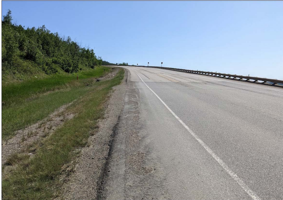
Photo 7: Looking from the shoulder of the SBL at Sta. 1+670 across the dip in the highway at the north end of the 1+800 slide.
