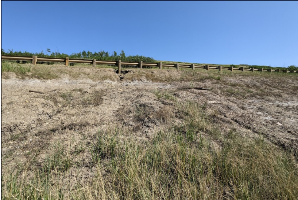
Photo 9: Looking east near Sta. 1+550 at fresh erosion rills and gullies developed on the highway side slope. Erosion became worse in 2023
