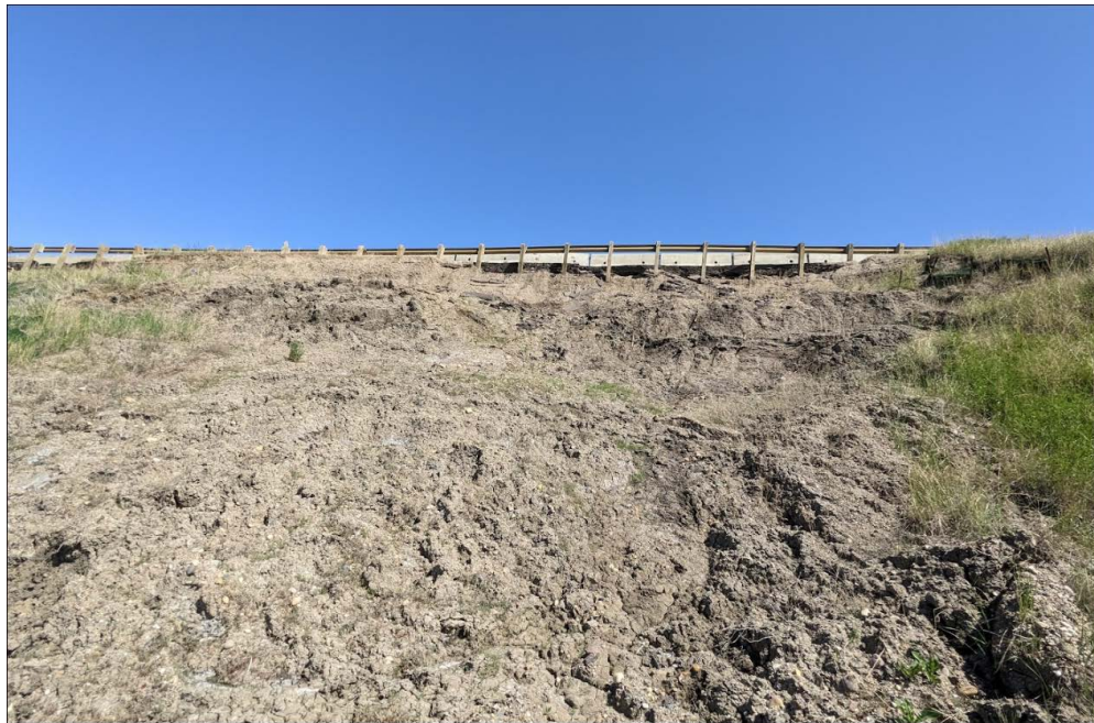
Photo 11: Looking east at failed soil matting and nails which were installed in August 2010 at Sta. 1+450 slide.
