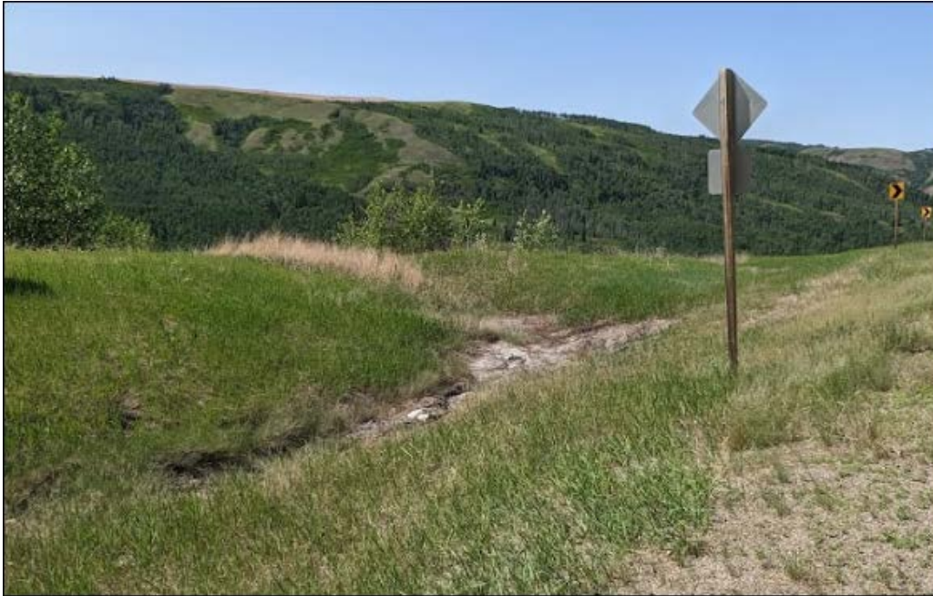
Photo 1: Looking northwest from Sta. 2+000 at erosion gully in SBL ditch south of ditch block
