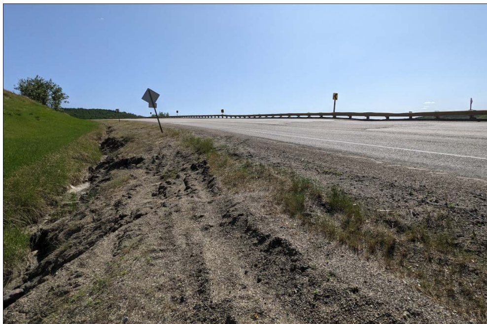
Photo 6: Looking south across the dip in the highway at the south end of the 1+800 slide.
