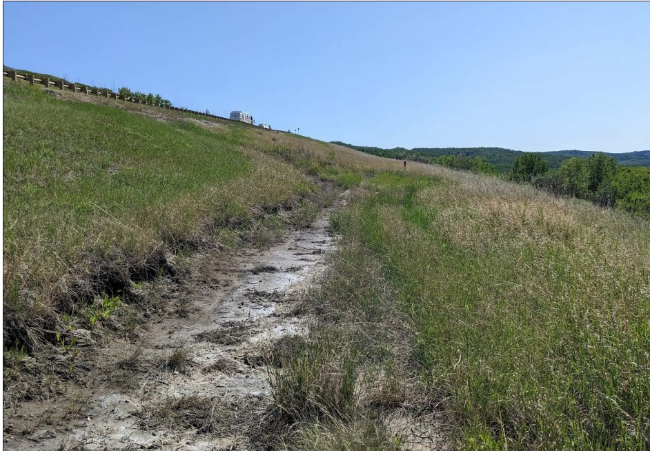
Photo 15: Looking south at the north end of slumping occurring from Sta. 1+450 to 1+550. Photo showing a drop of about 0.3 m
