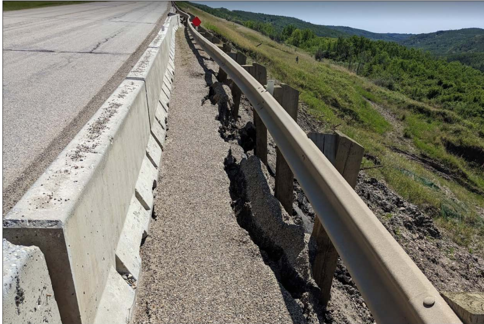
Photo 13: Looking south from Sta. 1+390 at the backscarp of the 1+400 slide which is impacting the highway shoulder. Slide cracks are wider and closer to the driving lane
