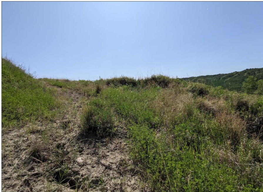
Photo 16: Looking south at the middle portion of slumping occurring from Sta. 1+450 to 1+550. Photo showing a drop of about 1 m.
