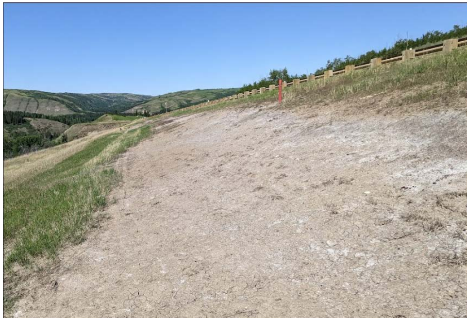
Photo 10: Looking north near Sta. 1+560 at rough area (drill access bench) with some seepage and tension cracks
