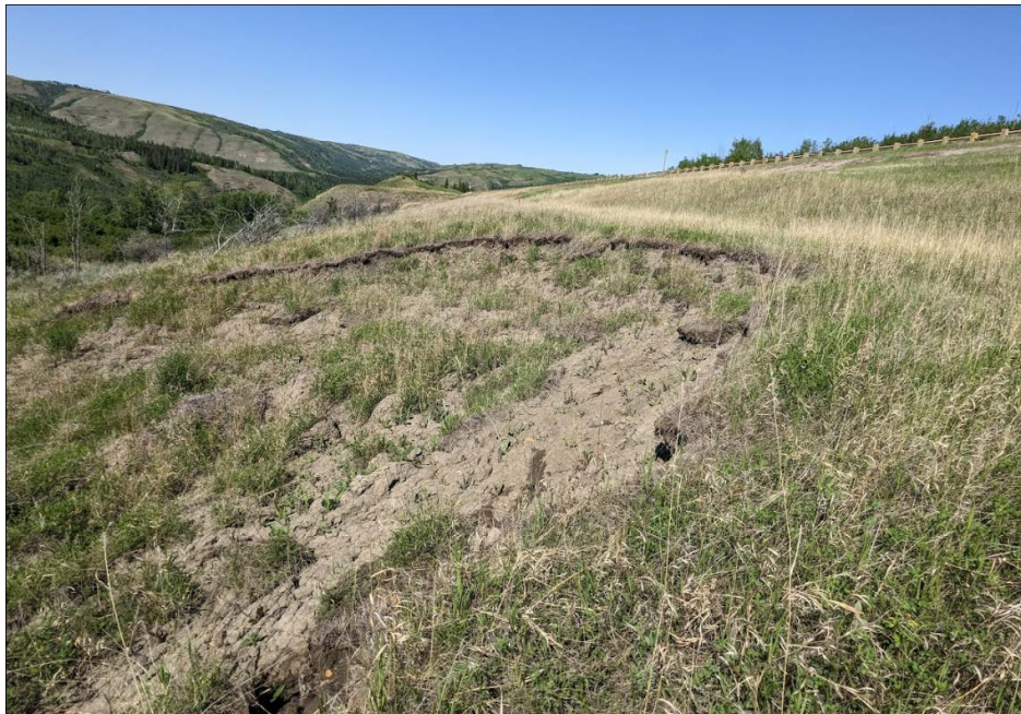
Photo 8: Looking north near Sta. 1+670 at slumping occurring on the highway side slope approximately 20 m from the edge of pavement. More movement noted since 2022
