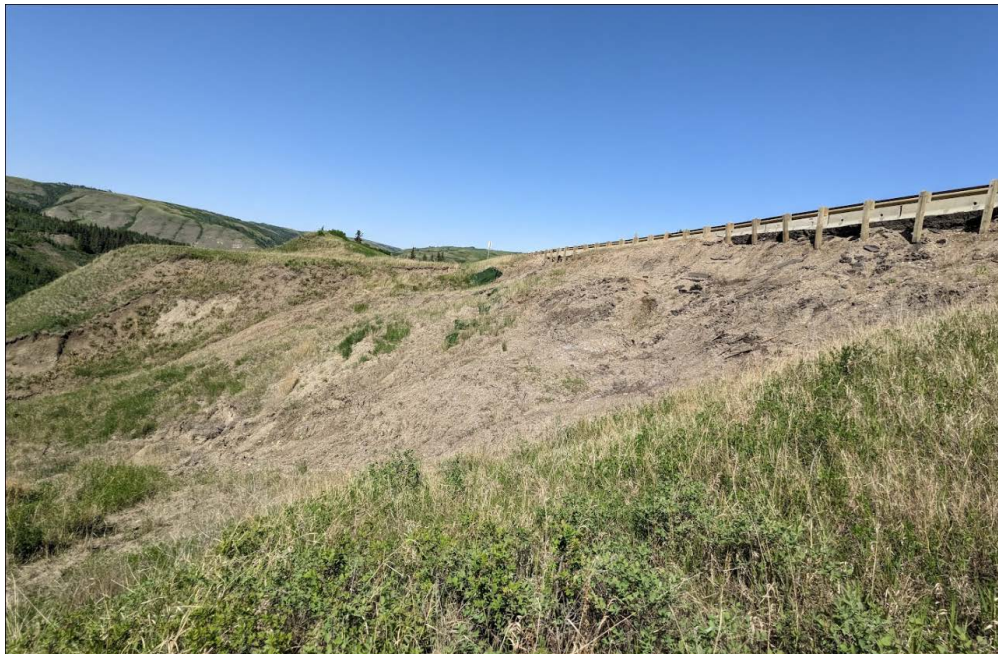
Photo 14: Looking north towards the 1+400 slide. The slide has further retrogressed towards the highway, is wider than in 2022 and there is a 5 m to 7.5 m drop below the guardrail.
