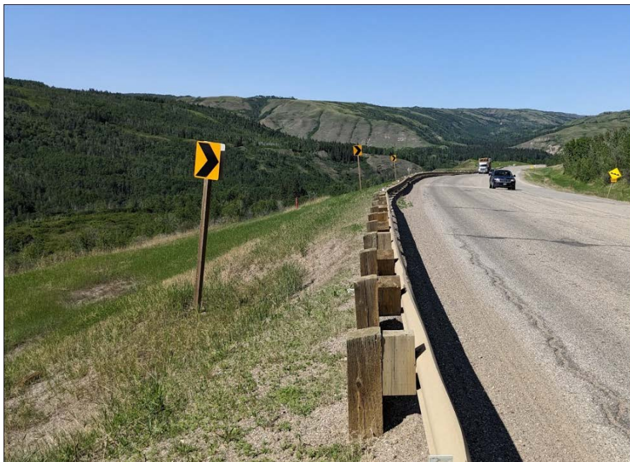
Photo 4: Looking north from Sta. 1+890 at the slump in the sideslope of the SBL. More movement since 2022. The scarp is 1.5 m high and 0.4 m from the guardrail.
