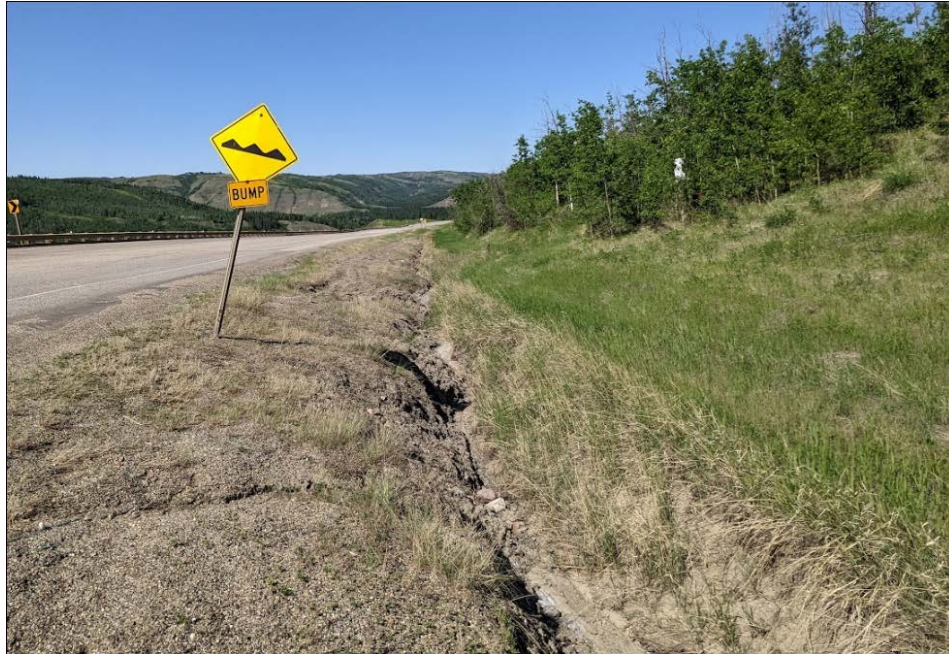
Photo 5: Looking north from Sta. 1+800 at the erosion gully developed on the ditch up to 5 m wide and 0.8 m deep. Erosion gully wider and deeper than noted at the 2022 inspection.
