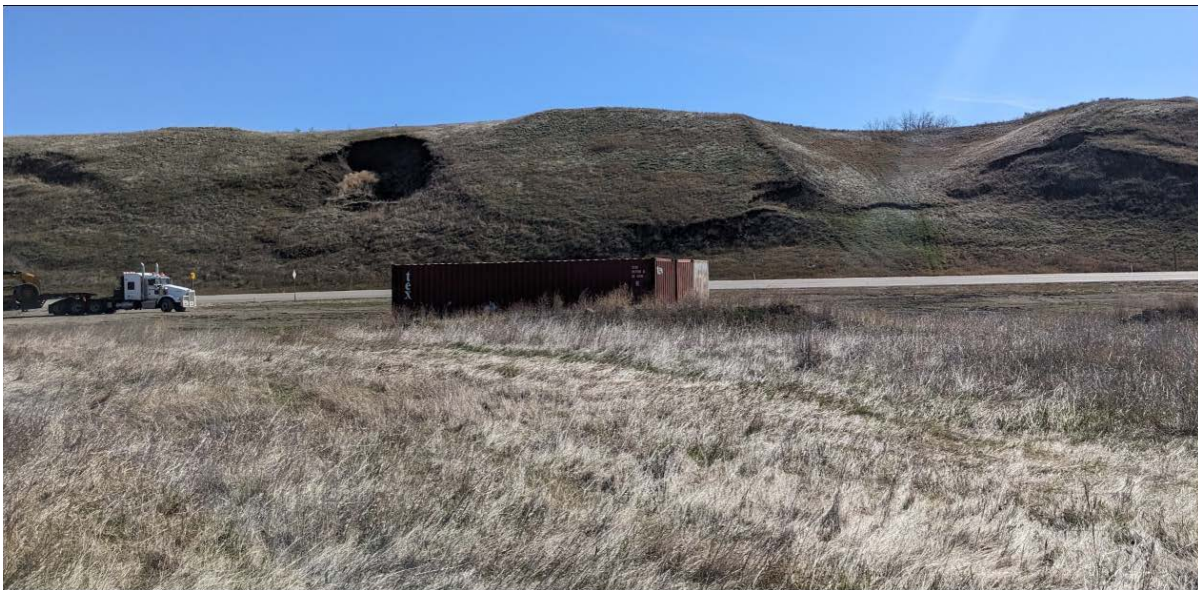
Photo 6. Looking east at backslope slumps showing ongoing creep movement
