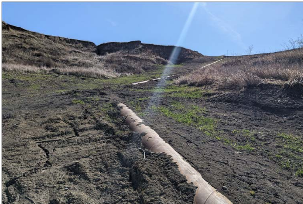
Photo 4. Minor Rills and some seepage noted in 2024
