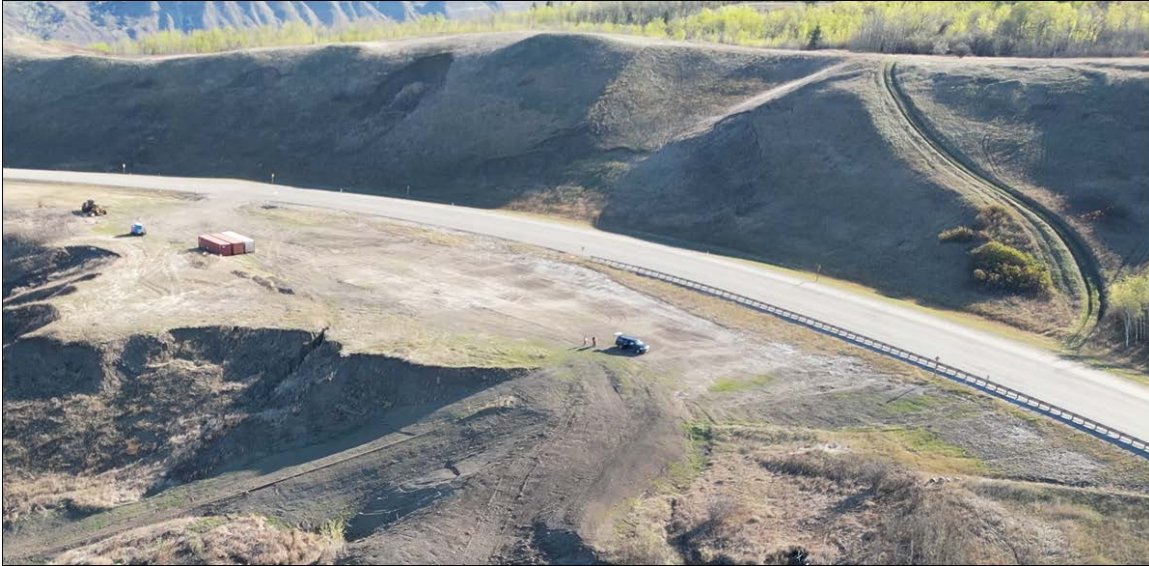
Photo D3. Oblique drone view of backslope slumps
