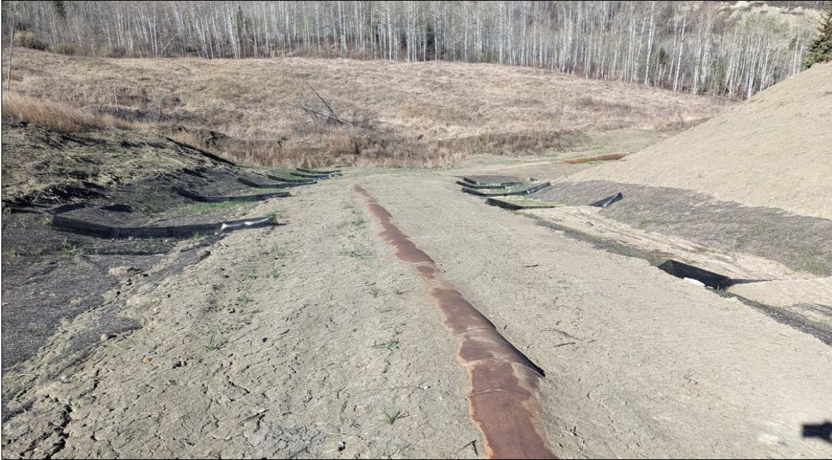
Photo 5. Looking downslope at SWSP middle bend where the ground surface shaped, seeded, and swales were lined with TRM and protected with geosynthetic ditch barriers.
