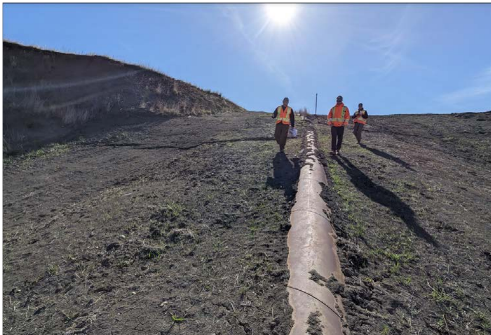
Photo 2. Looking upslope at Elephant Trunk Pipe where fill was placed in 2023 to support the underside of pipe and erosion gullies.
