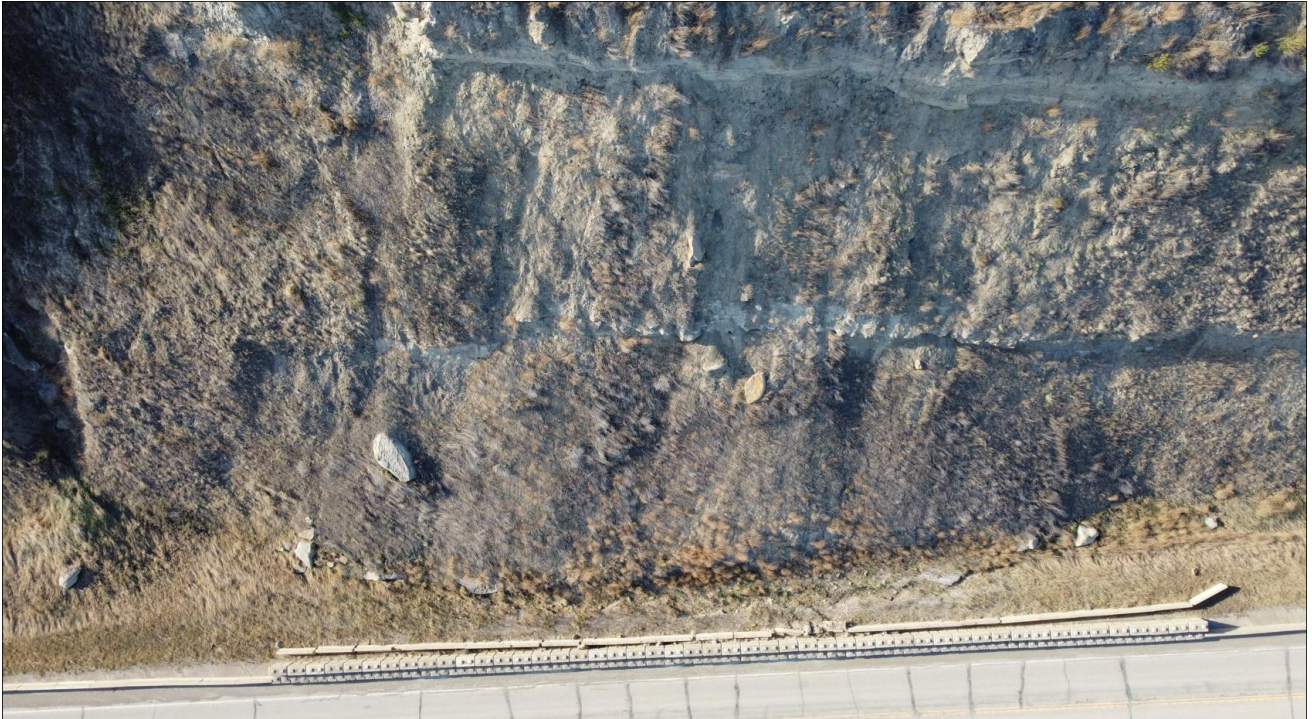
Aerial Photo 7: Few sandstone rock slabs accumulating behind the Concrete Jersey Barrier
