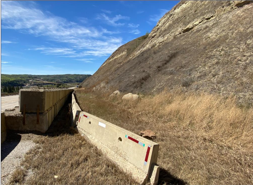
Photo 3: Looking west at accumulated debris in the ditch below the landslide.
