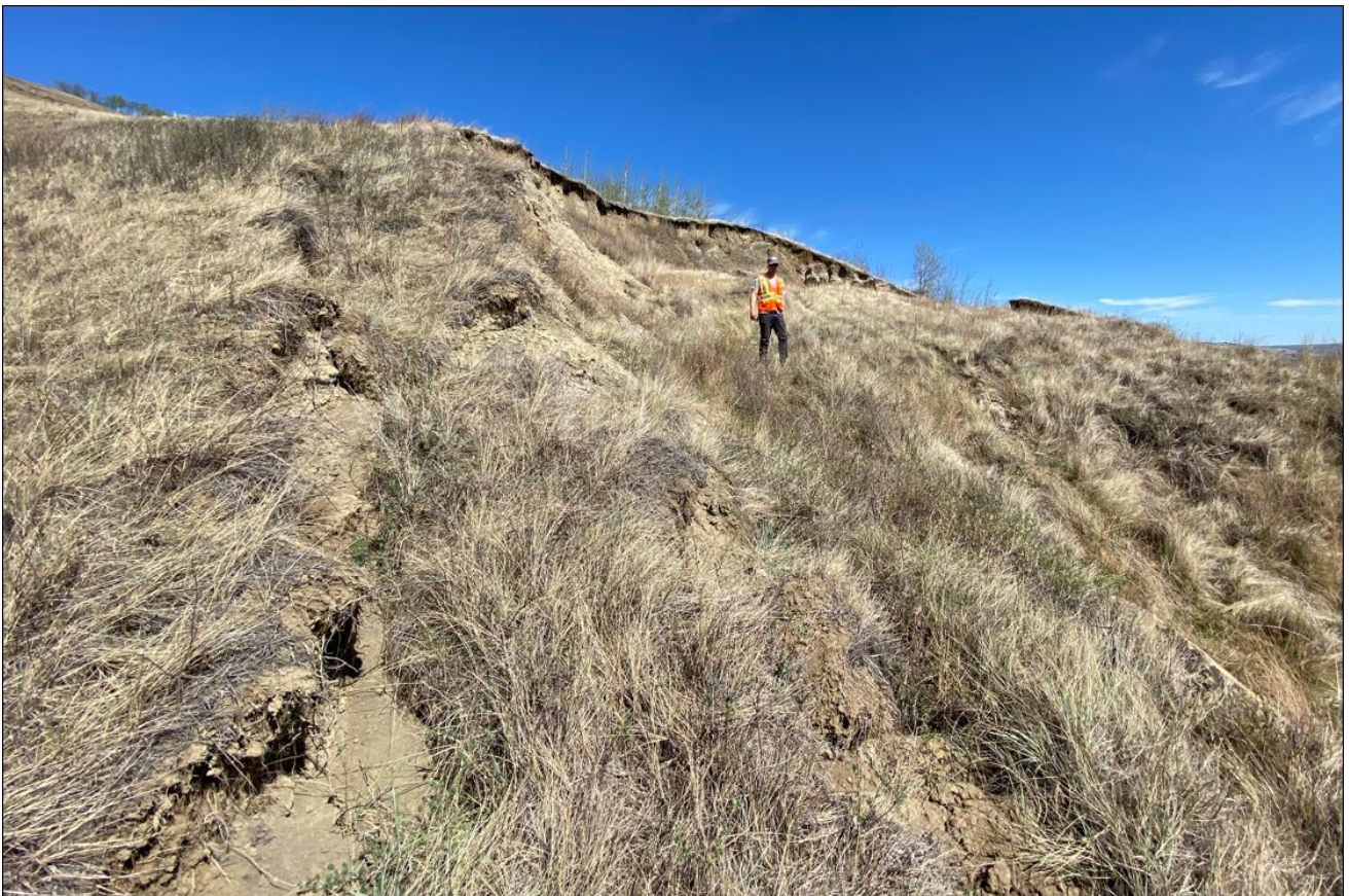
Photo 6: Landslide backscarp showing movements since 2023.
