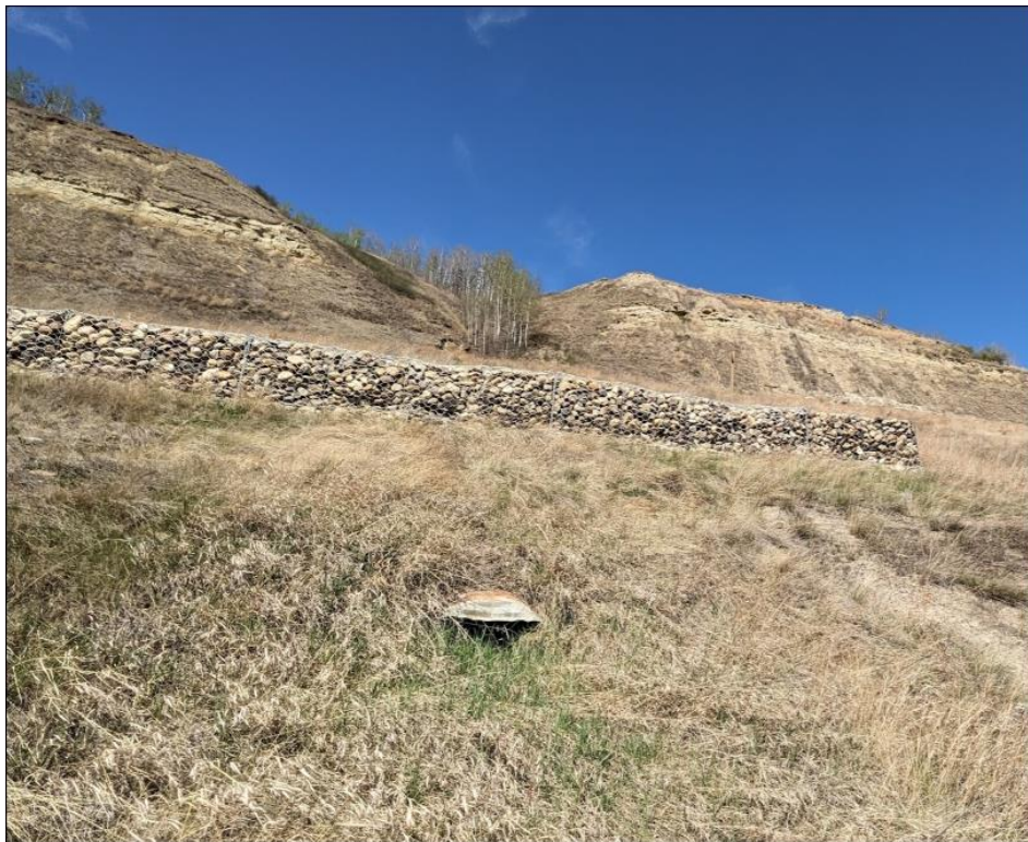
Photo 10: 600 mm CSP Culvert. Approximately 300 mm buried under sediment. Dry in 2024
