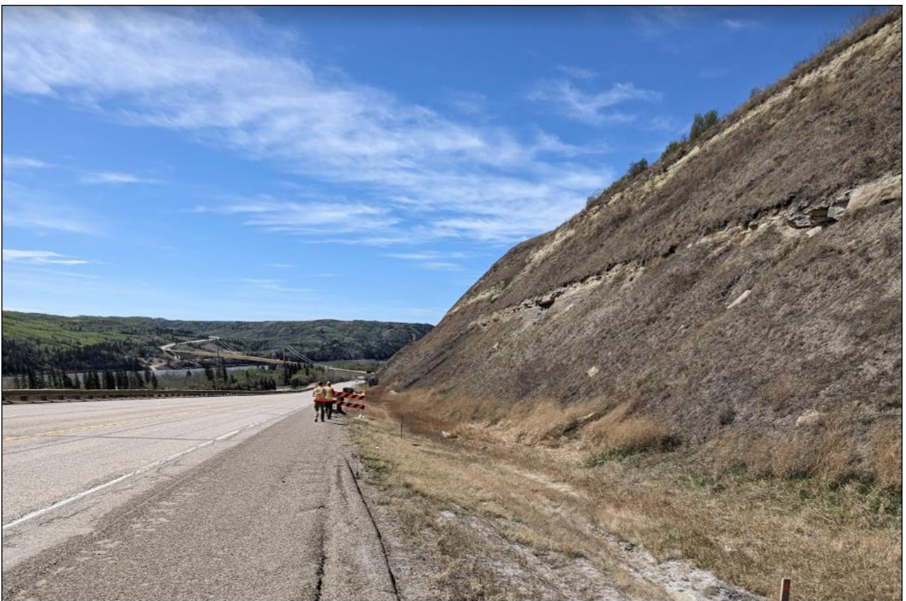
Photo 2: Looking west at the highway backslope and concrete barriers below the landslide
