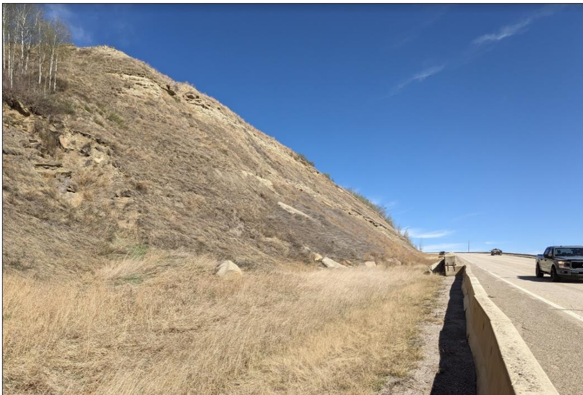
Photo 8: Looking east at steep rock backslope and a few sandstone blocks accumulating behind the Concrete Jersey Barrier
