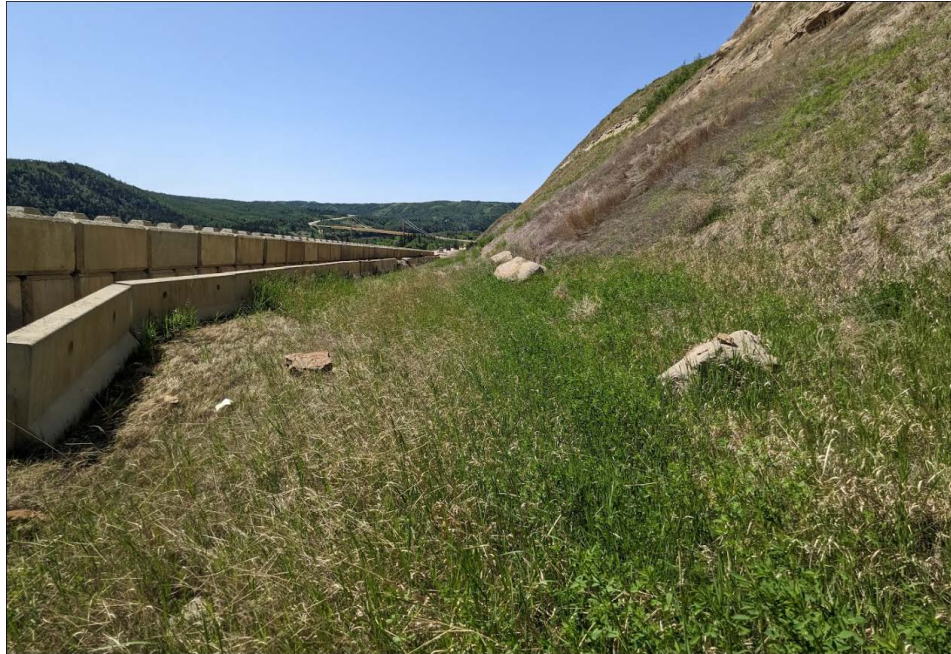
Photo 3: Looking west at accumulated debris in the ditch below the landslide.
