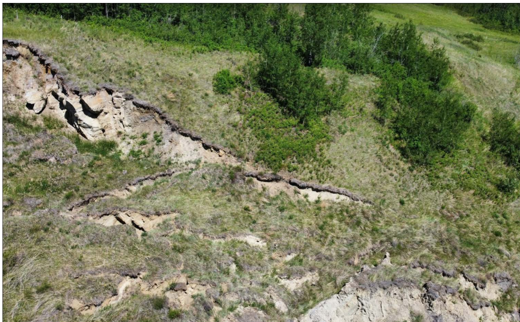
Aerial Photo 8: Looking east landslide backscarp eastern flank
