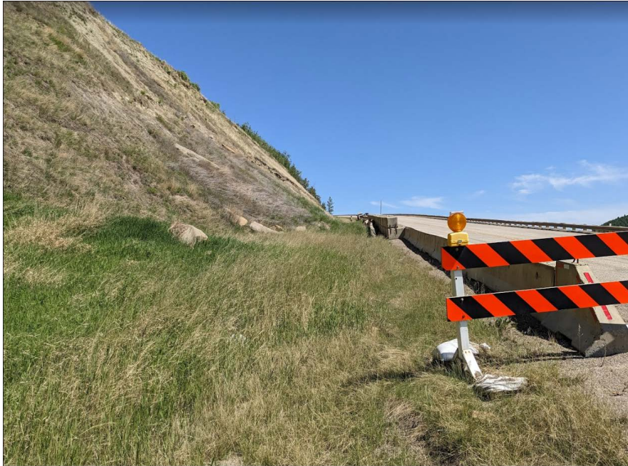
Photo 11: Looking east at steep rock backslope and a few sandstone blocks accumulating behind the Concrete Jersey Barrier |
