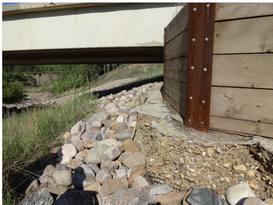
Photo 4. Looking east at the corner of the pile wall and settled riprap. Photo credit: Nicole Wilder.
