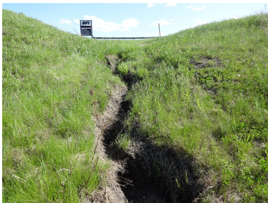
Photo 6. Looking south at erosion gully that has formed east of the south side of the bridge. Photo Credit: Nicole Wilder.
