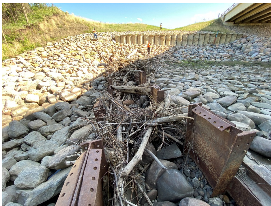
Photo 10. Looking south at debris that has accumulated in the pile weirs. Photo Credit: Don Proudfoot.
