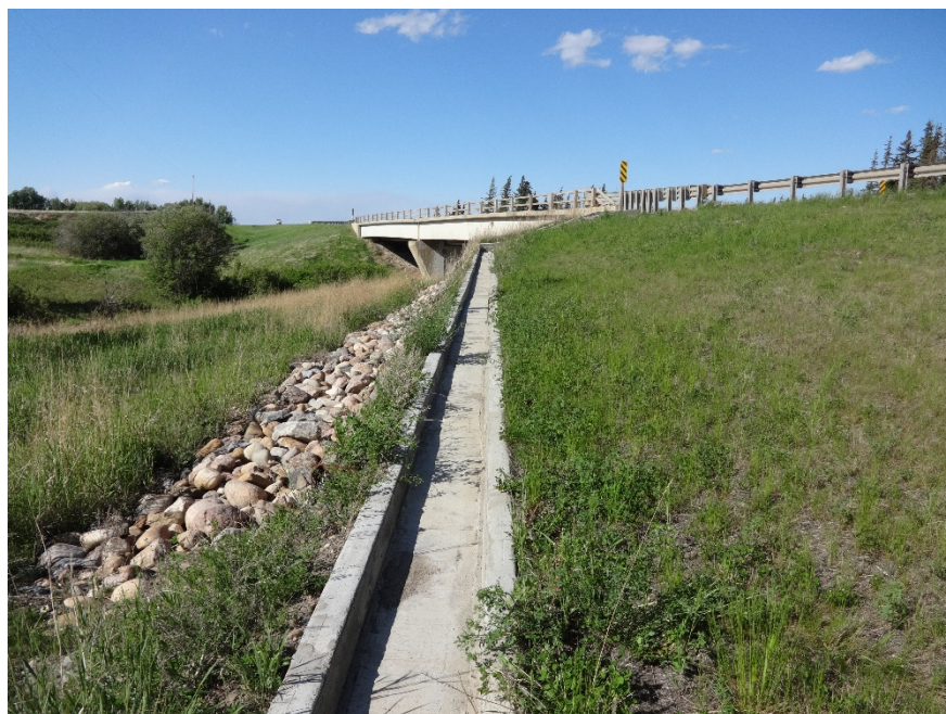
Photo 2. Looking northeast at the concrete drain trough above the west pile wall. Photo credit: Nicole Wilder.
