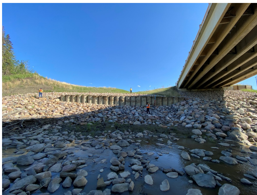
Photo 8. Looking south towards the east pile wall and riprap. Photo Credit: Don Proudfoot.
