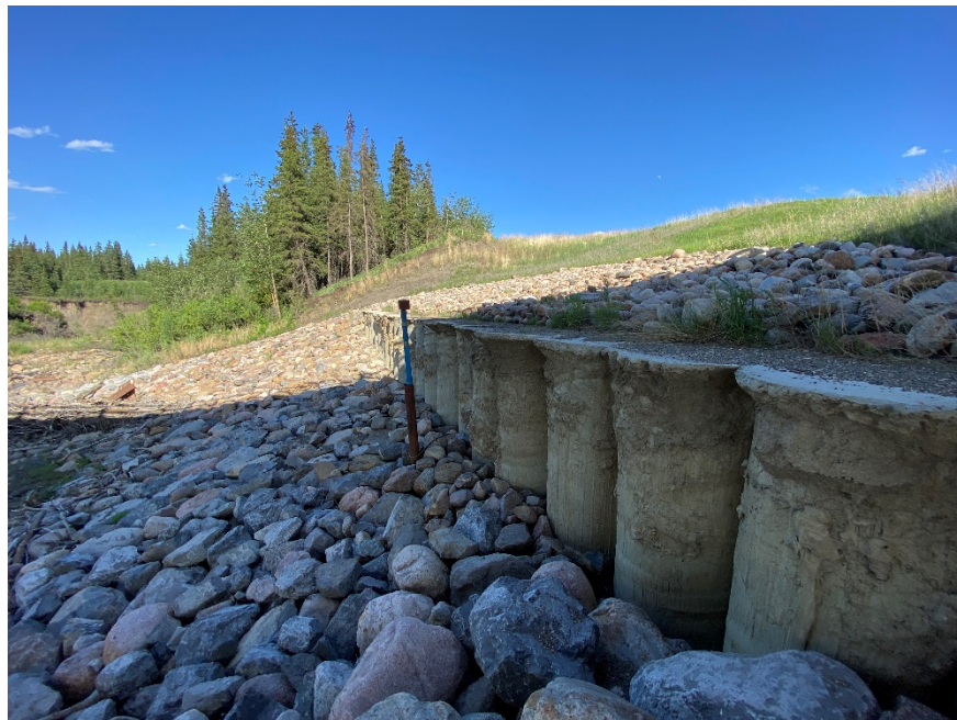
Photo 7. Looking east at riprap that settled below the east pile wall. Photo Credit: Don Proudfoot.
