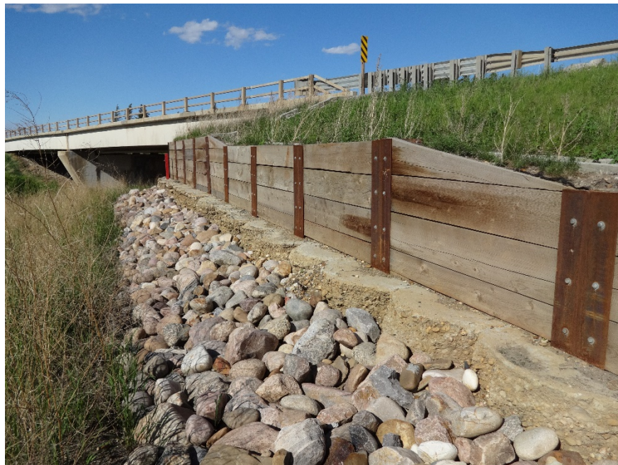
Photo 3. Looking northeast at riprap that appeared to have settled on the downslope side of the pile wall. Photo credit: Nicole Wilder.
