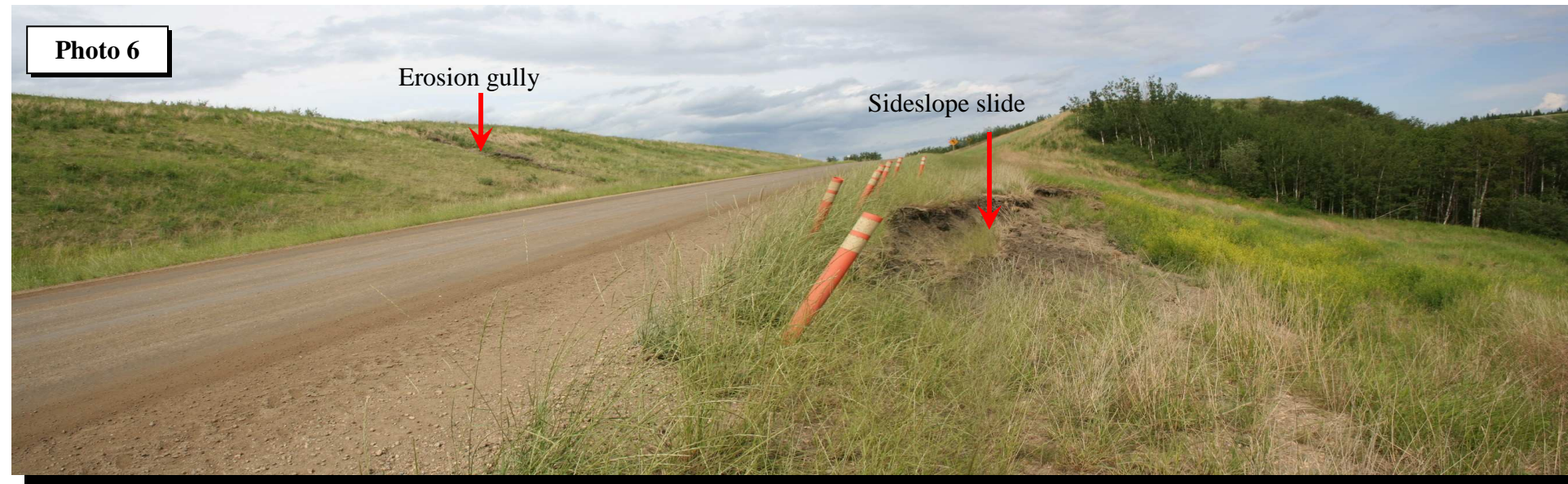
Looking upgrade north (away from Hwy. 49 Jct.) - Sideslope slides (right) has encroached to shoulder of northbound lane - Erosion gully formed at backslope (left) as a result of runoff from upland farm area
