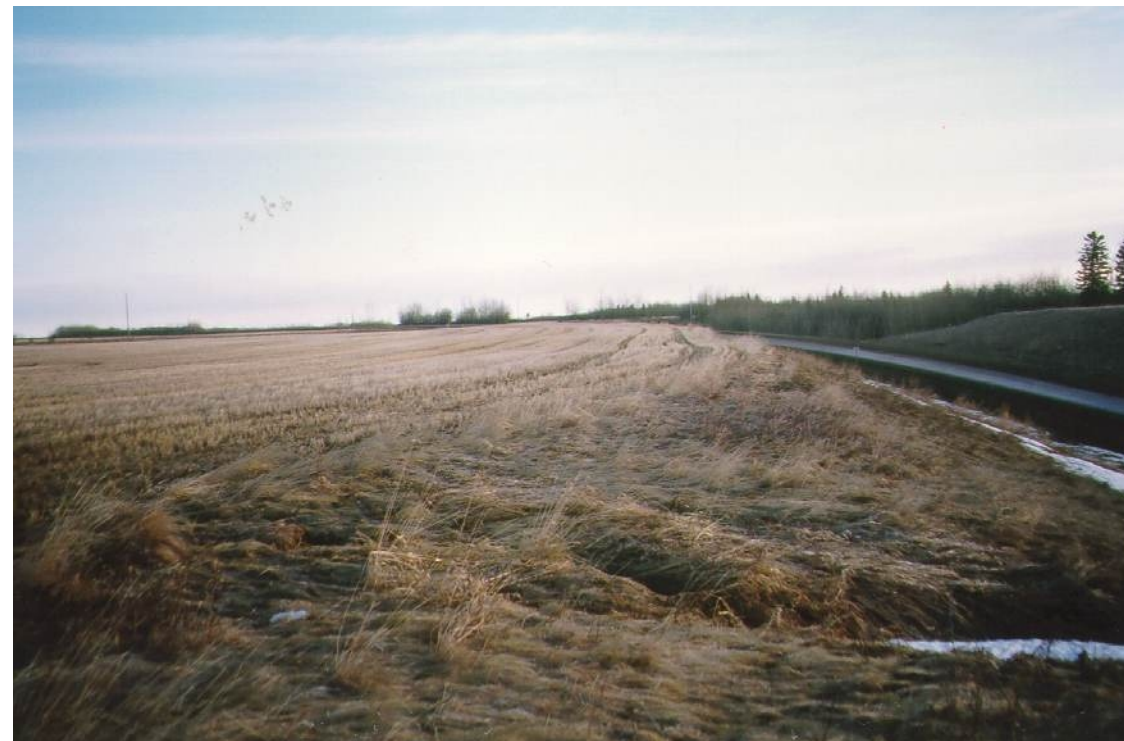
Photo 15 Looking north upgrade (along top of valley slope) 1) Surface water outfall down backslope to cause concentrated flow erosion 2) No swale or catchwater ditch (dyke) along perimeter of upland farm
