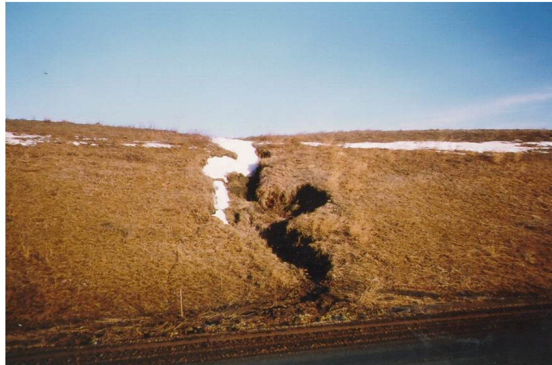
Photo 13 3 m depth erosion gully at backslope Effect of erosion from upland (farm) runoff
