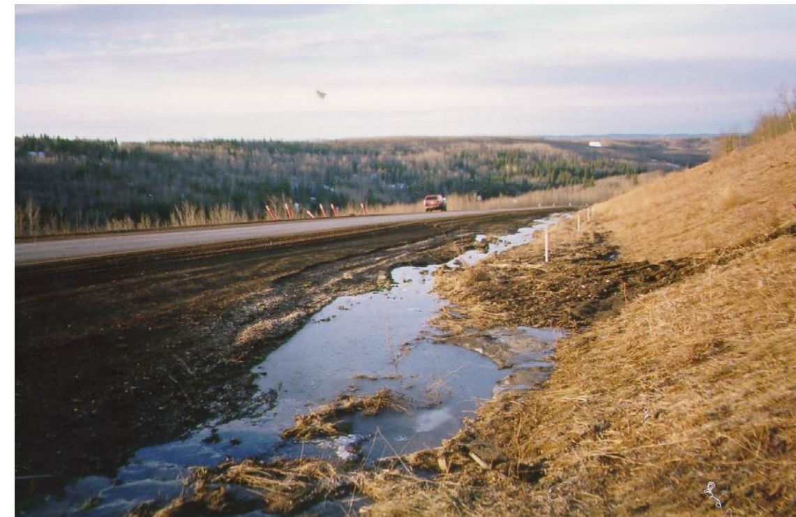
Photo 16 Toe of slope 1) Water ponding and erosion debris along backslope ditch
