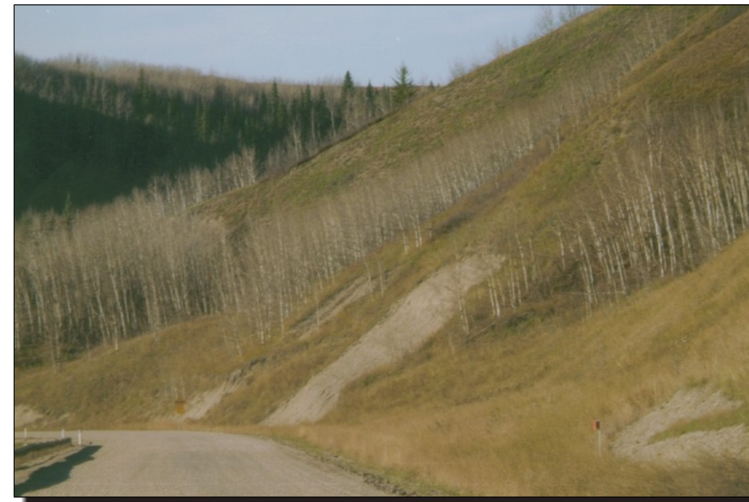
Photo 5d Steepening of backslope.
