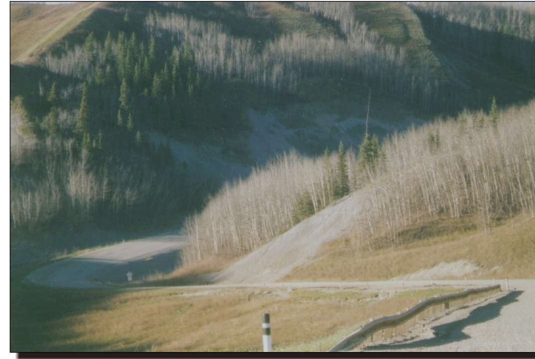
Photo 5c Sideslope slide transgressing highway centreline. Gravel road regraded to allow passage of traffic.
