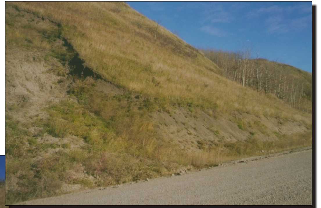
Photo 4c Another view. Steepening of slope toe from previous shifting of alignment.
