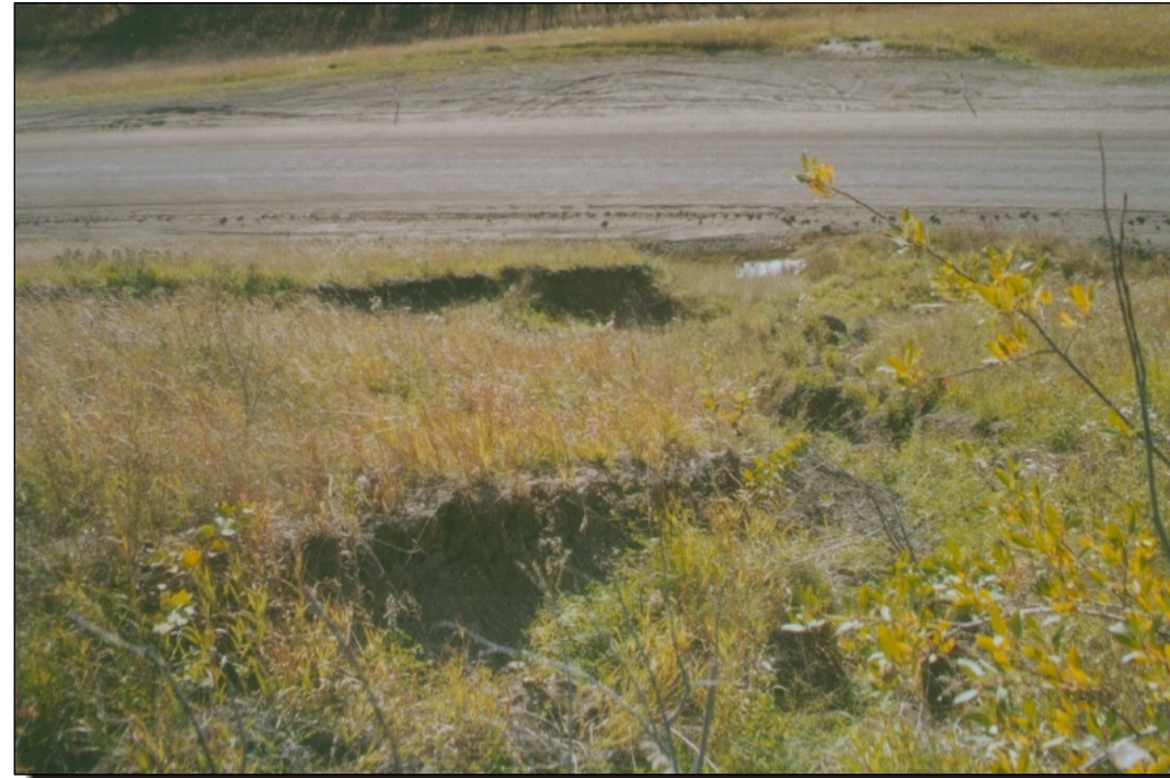
Photo 4a Looking downslope from upland. Centre portion of alignment. Backslope slide - erosion gulley formed from a breach of a low dyke along the upland edge causing snow melt runoff concentrated flow to erode down the backslope.
