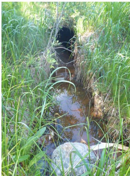
Photo 10: Ponded water at the culvert outlet near km 12+900.
