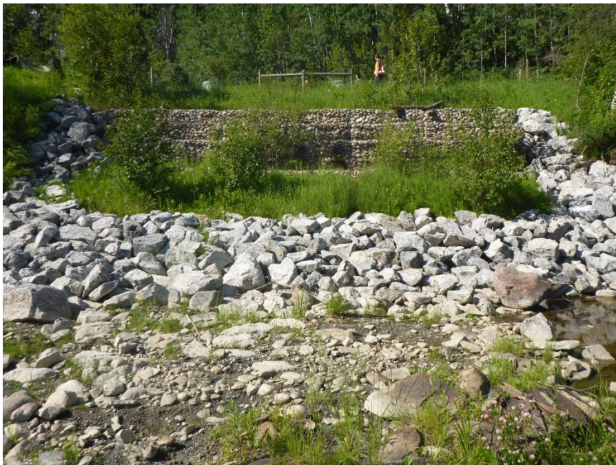
Photo 8: Some flow was observed out of the gabion outfall. Looking southwest.
