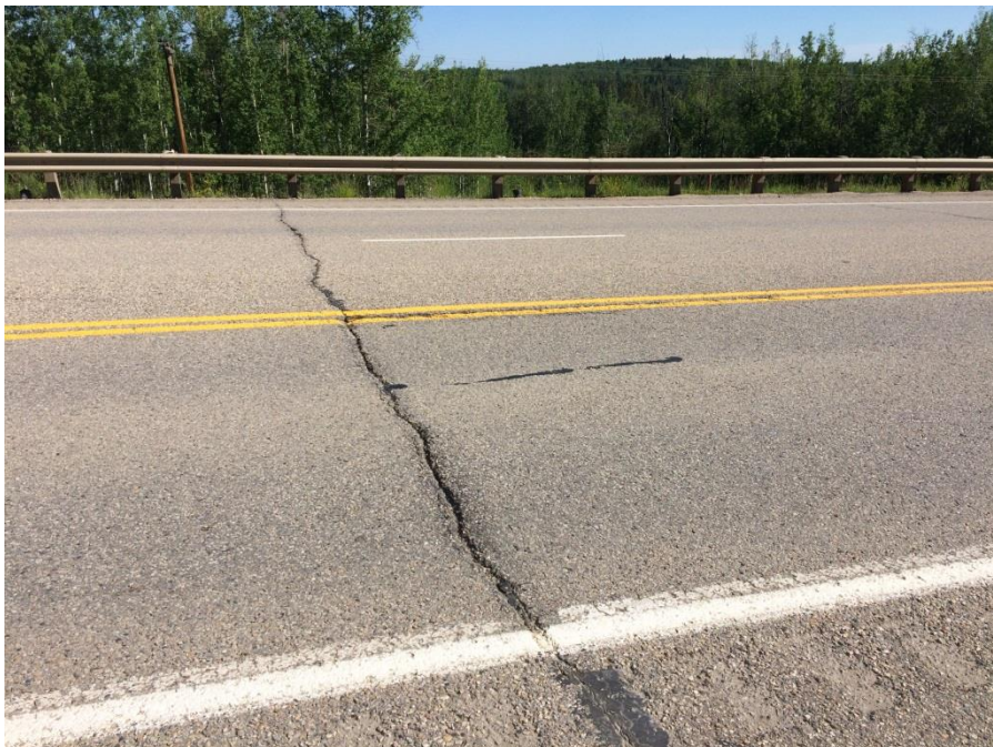
Photo 2: Transverse crack up to 70 mm wide. Looking north.
