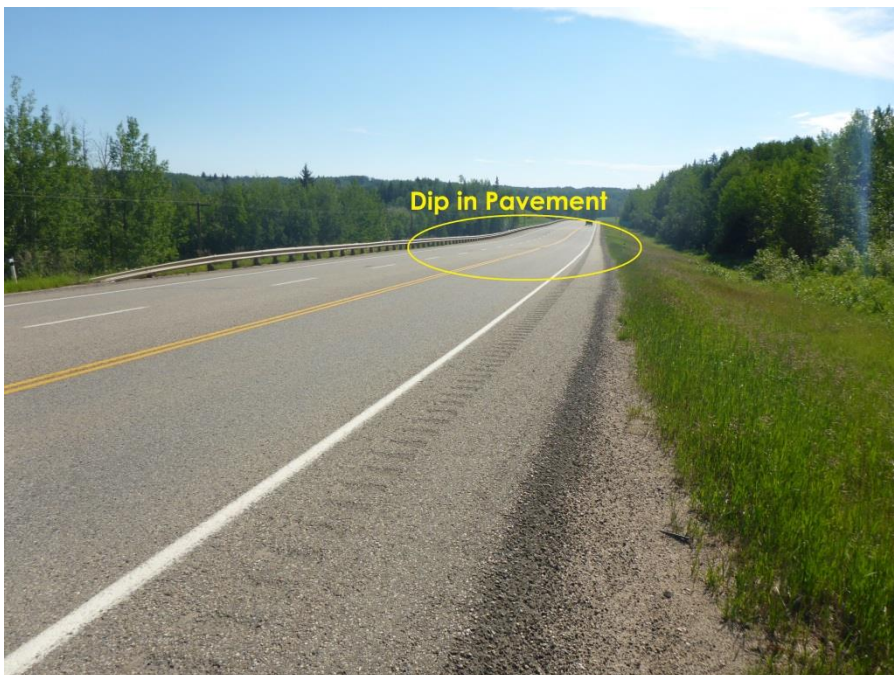
Photo 4: Slight dip in pavement at approximately 12+900 km. Looking east.
