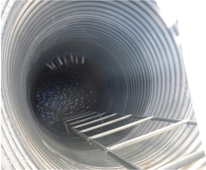
Photo 7: Estimated flow of approximately 1L/min in the west drainage gallery.
