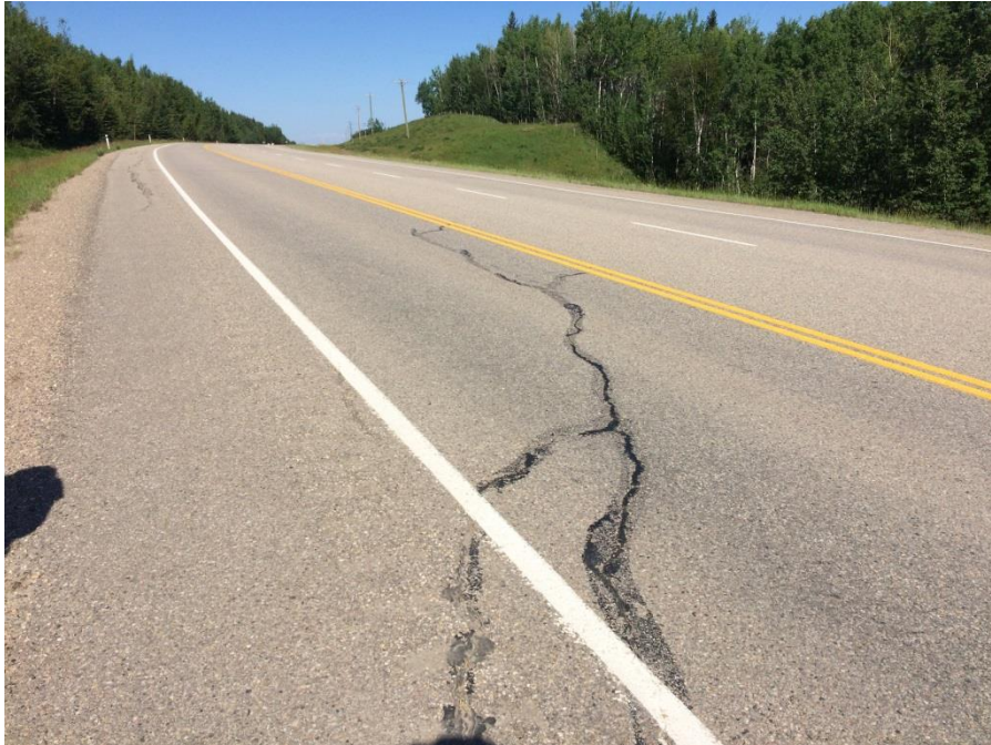
Photo 1: Sealed pavement crack north of SI01-1 on eastbound lane. Looking northwest.
