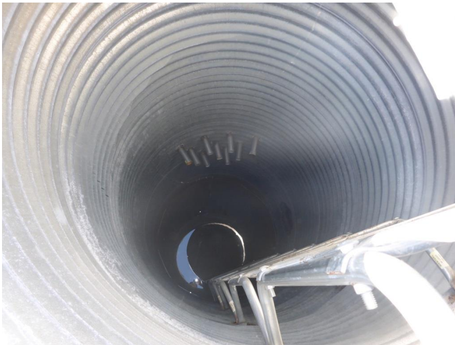
Photo 6: No flow in east drainage gallery.
