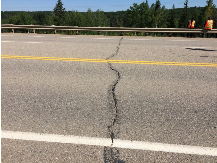
Photo 3: Transverse crack up to 100 mm approximately 10 m from the east culvert. Looking north.
