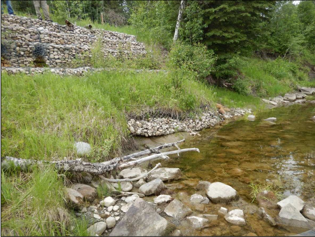
Photo 4: Erosion and deformation of gabion baskets along riverbank at toe of slope
