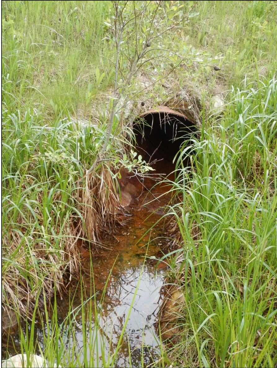
Photo 5: Ponding water at west culvert outlet
