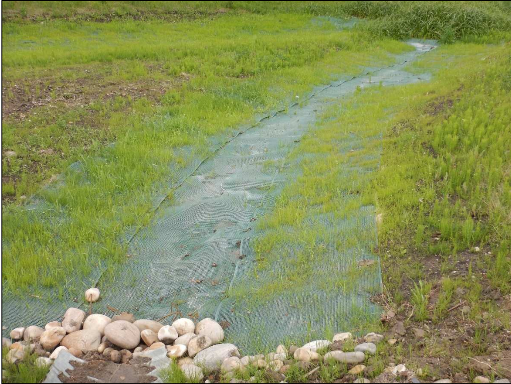
Photo 6: Erosion and sediment control installed along drainage path immediately west of the site
