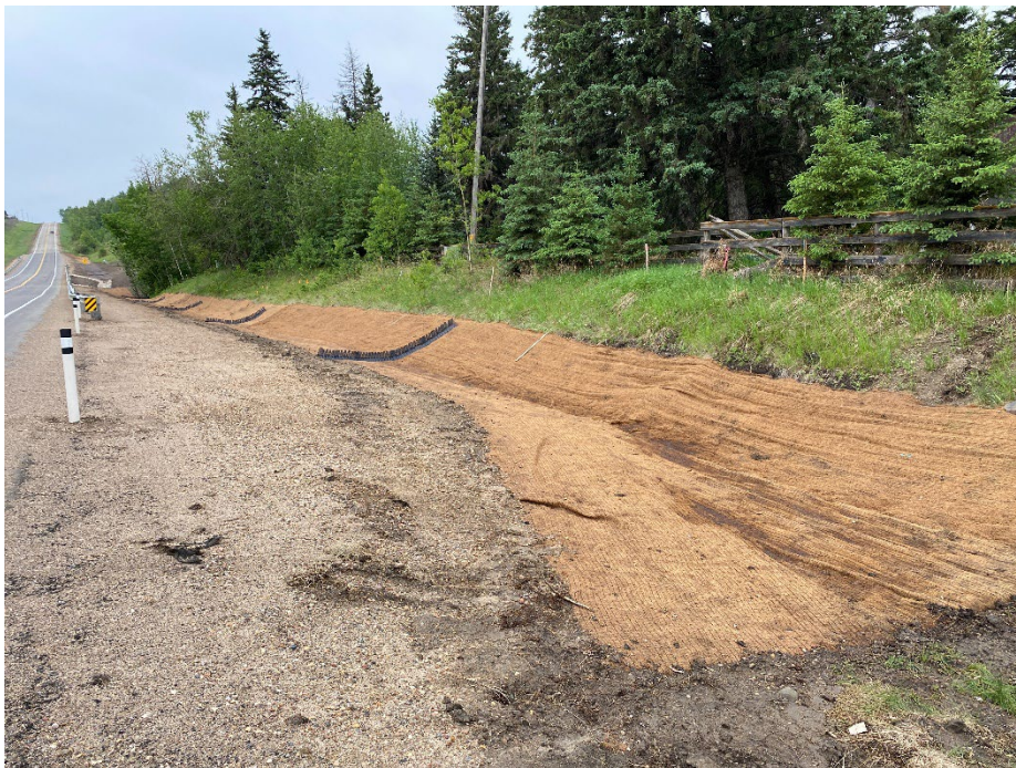
Photo 4: Erosion control blankets and georidges in west ditch. No vegetation observed in the ditch. Looking southwest.
