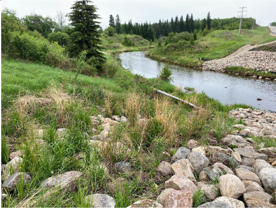
Photo 7: Failure on east side of north bank has been backfilled with riprap and finer soils. Well vegetated. Looking southeast.
