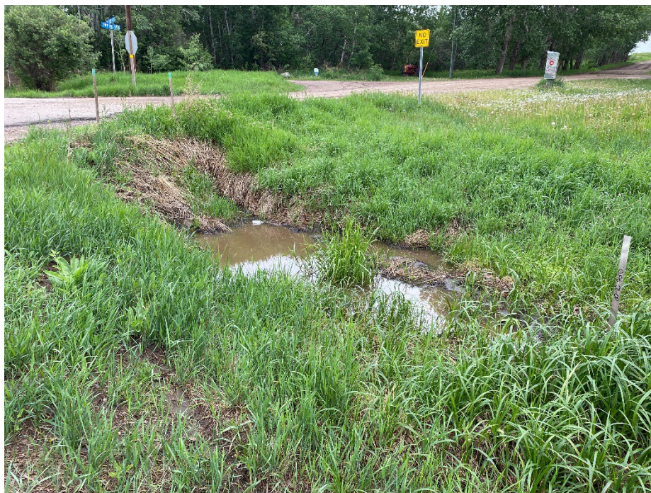
Photo 2: Ponded water in east ditch by culvert outlets. Looking northeast.
