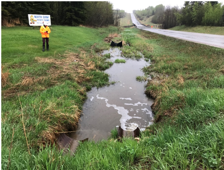
Photo 3: Erosion gully along east ditch. Looking south from culvert outlet.
