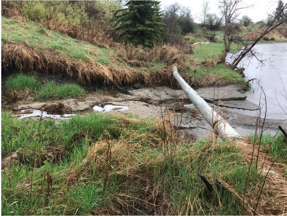
Photo 5: Irrigation pipe undermined by erosion and slump, approximately 6 m wide. Looking east.
