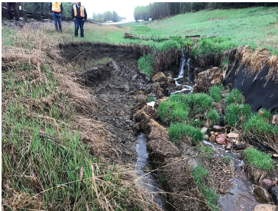
Photo 4: Slump adjacent to bridge abutment approximately 8 m to 10 m wide. Straw bales fell into slump from scarp retrogression. Looking north.
