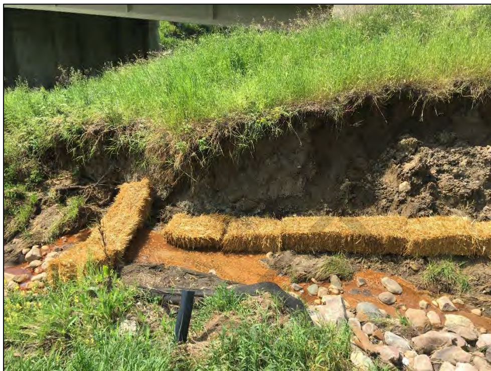
Photo 7: Water at base of eroded area, facing west.
