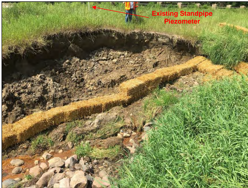
Photo 5: Upper section of eroded area, facing west.
