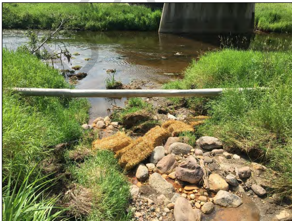
Photo 8: Undermined water pipe at lower section of eroded area, facing south.
