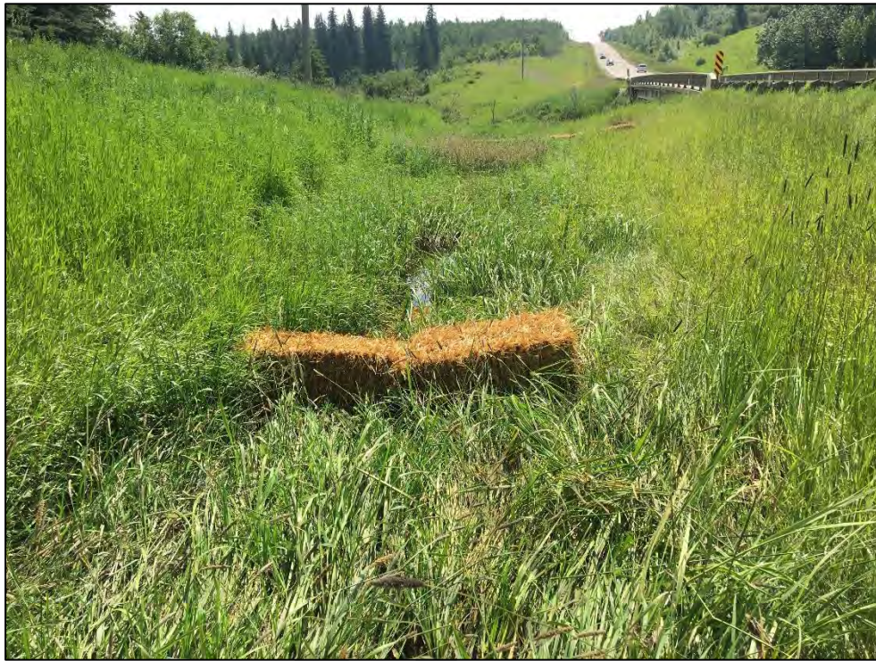
Photo 3: Standing water in ditch, facing south.
