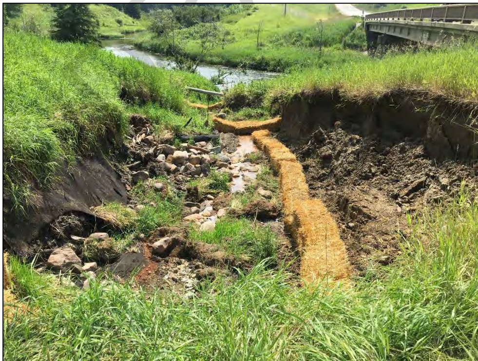
Photo 4: Upper section of eroded area, facing south.
