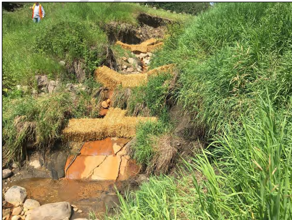
Photo 6: Upper section of eroded area, facing north.
