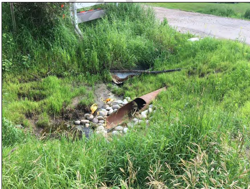
Photo 2: Inlet of culverts at North Bank Potato Farm access, facing south. Note that invert of CSP is above water level.
