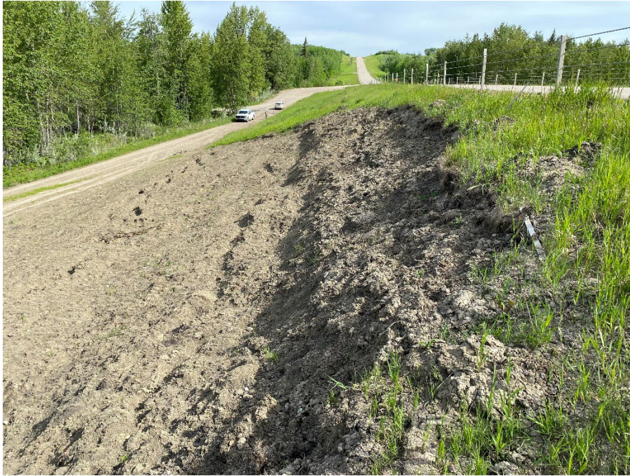
Photo 3: Backslope of failure regraded since previous inspection. Looking north.
