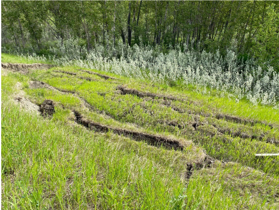
Photo 7: Toe bulge of northern slump on east sideslope. Looking northeast.
