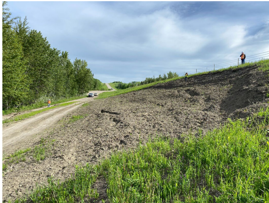
Photo 2: Failure at south extent of west side slope. Looking north.
