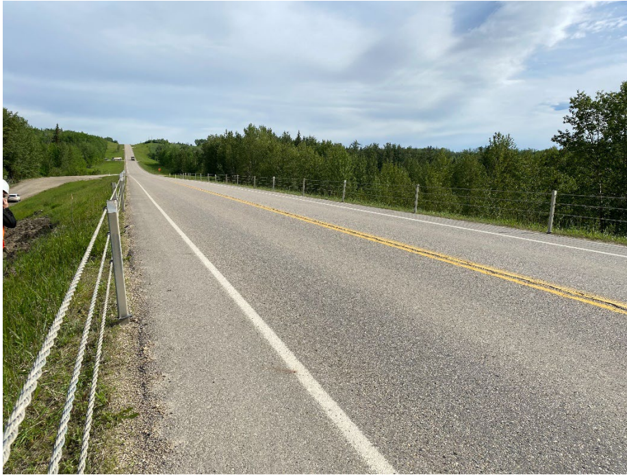
Photo 5: Highway surface above west sideslope failure. Looking northeast.
