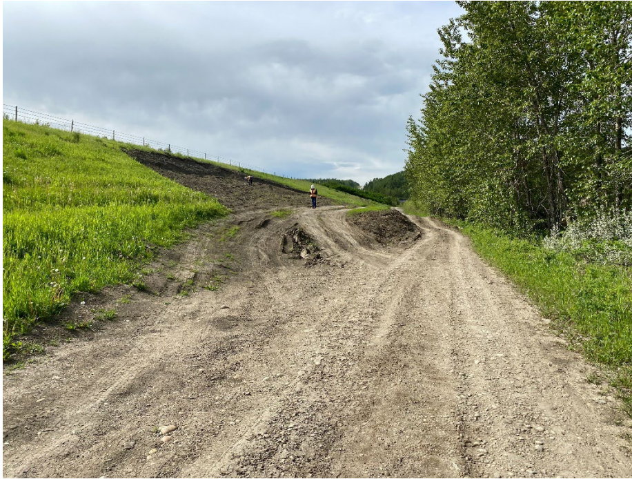
Photo 1: Failure at north extent of west side slope. Service road at landslide toe has been opened up. Looking south.
