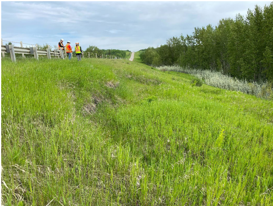
Photo 10: South slump on east sideslope relatively unchanged. Looking north.
