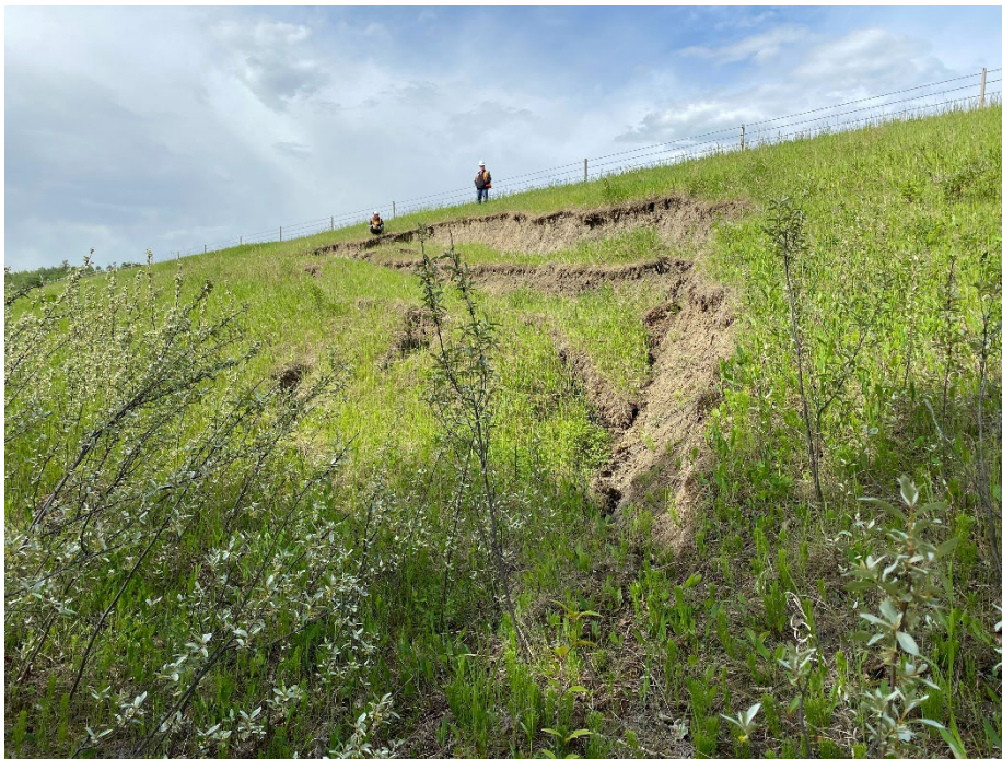
Photo 6: New slump on north end of east sideslope. Looking southwest from toe.
