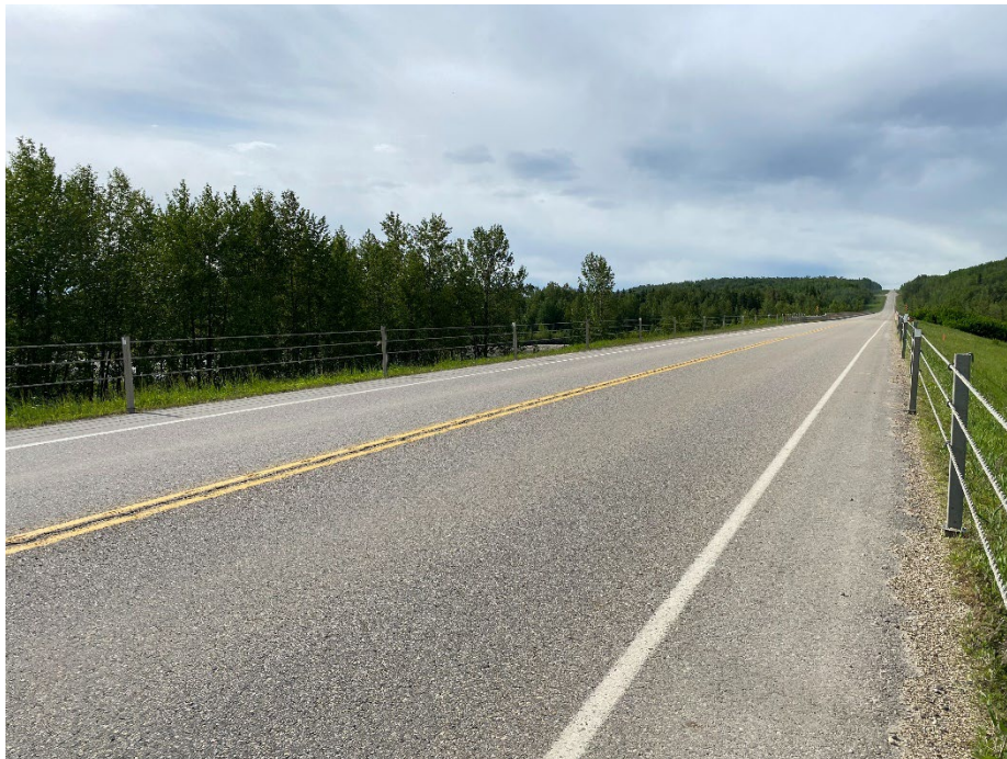
Photo 4: Highway surface above west sideslope failure. Looking southeast.
