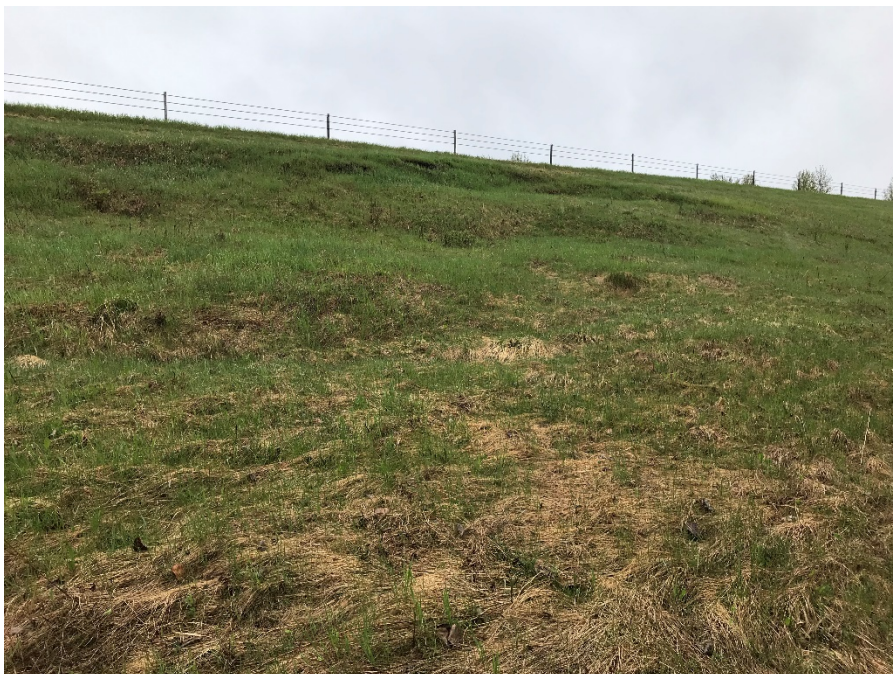
Photo 6: North slump on east slope looking west.
