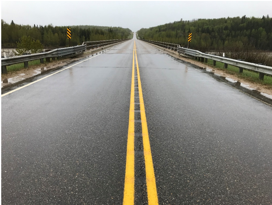
Photo 1: Pavement last milled and paved in 2016. Looking south.
