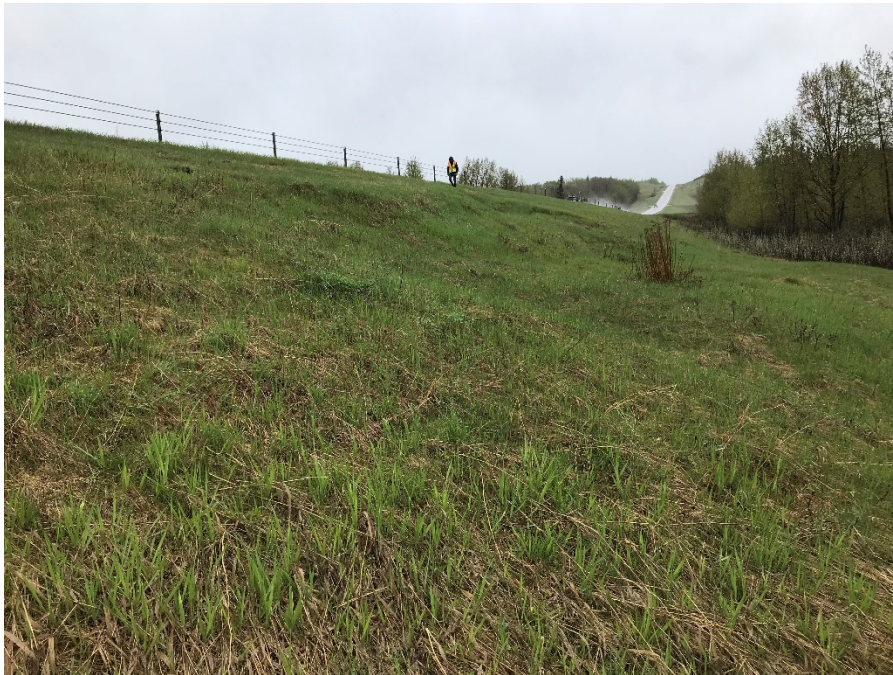
Photo 5: North slump on east slope looking northwest.
