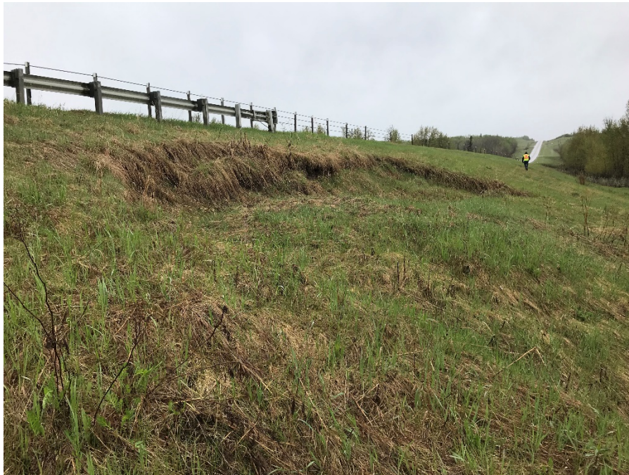
Photo 3: South slump on the east slope. Looking north.
