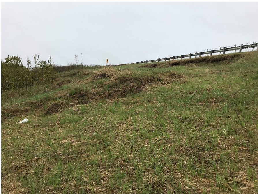
Photo 4: Toe bulge at south slump. Looking south.
