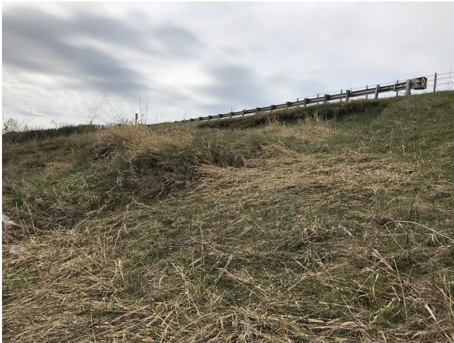
Photo 5: Toe bulge at south slump. Looking south.
