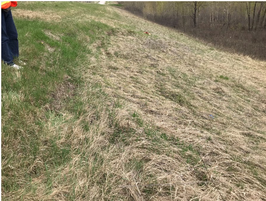
Photo 6: North slump on east slope looking northwest.
