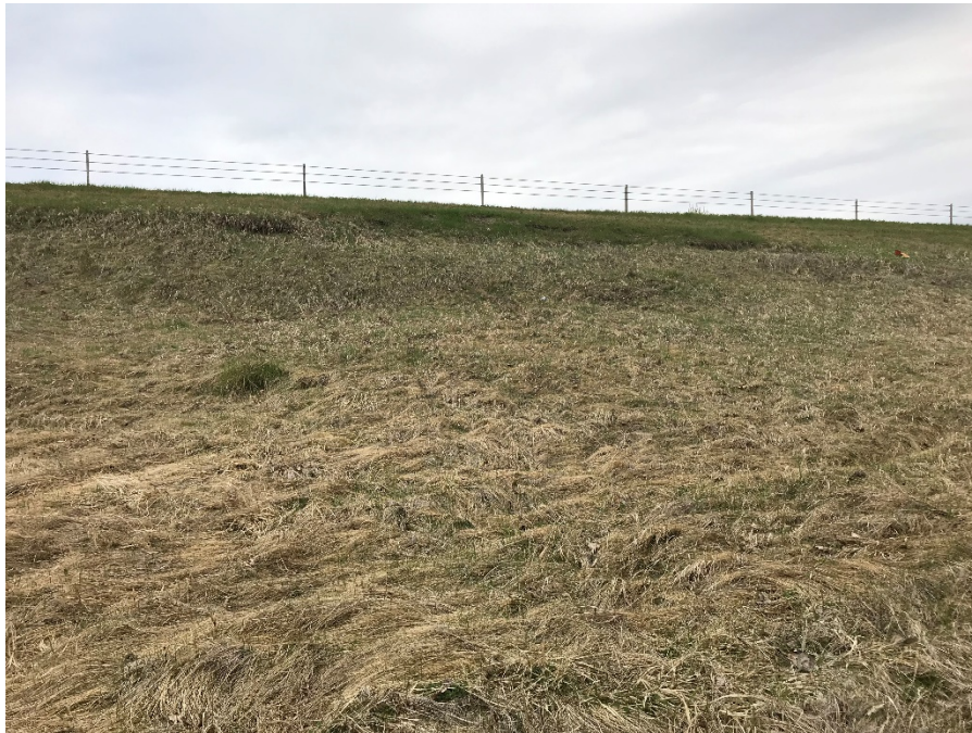
Photo 7: North slump on east slope looking west.
