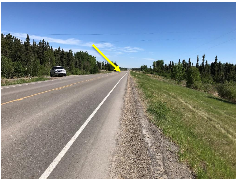
Photo 2: Pavement dip across from approach. Looking north.
