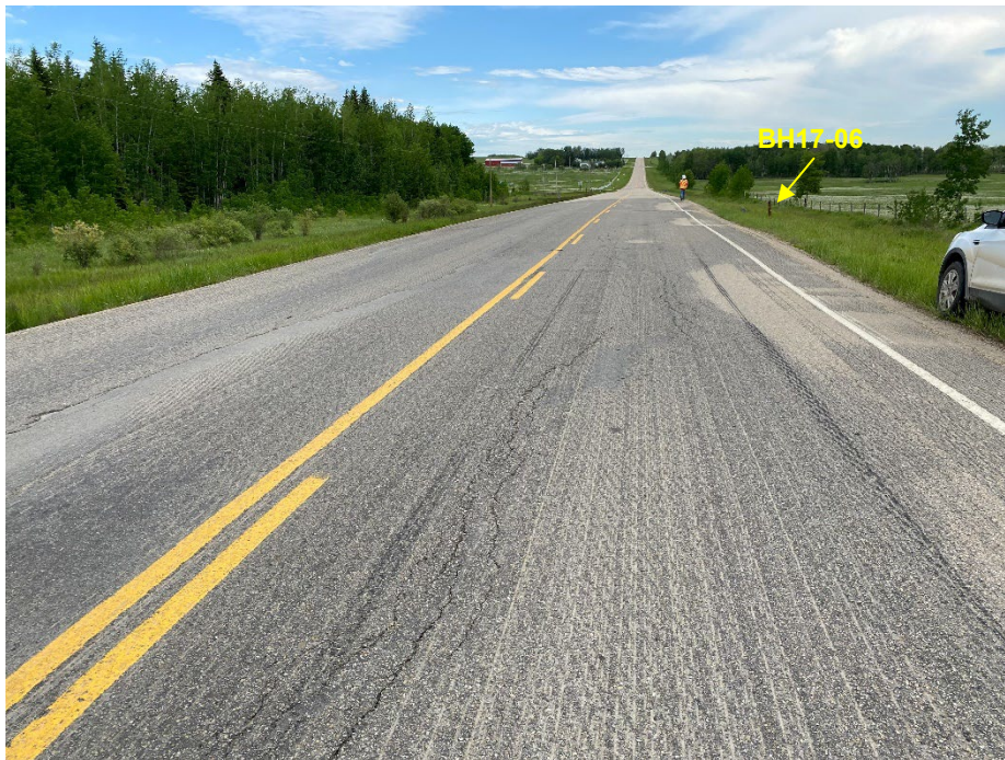
Photo 4: Pavement cracking on EBL. Looking east.
