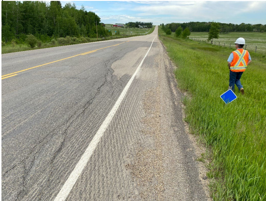
Photo 5: Pavement cracking on EBL. Looking east.
