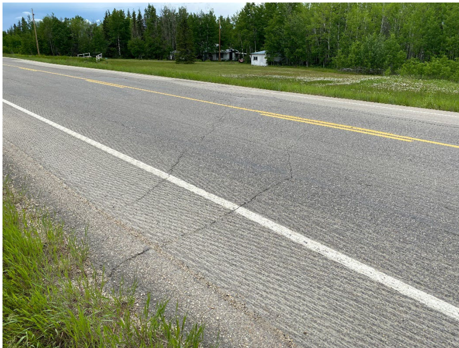
Photo 2: Diagonal cracking across milled pavement, looking northwest.
