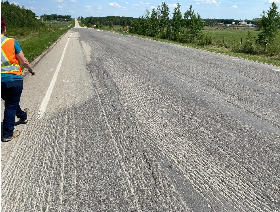
Photo 1: West limits of WBL pavement cracks. Looking east.
