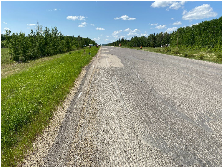
Photo 4: Pavement cracking on EBL. Looking west.
