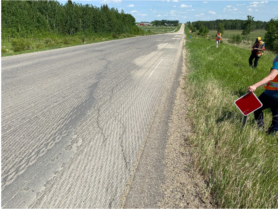
Photo 3: Pavement cracking on EBL. Looking northeast.
