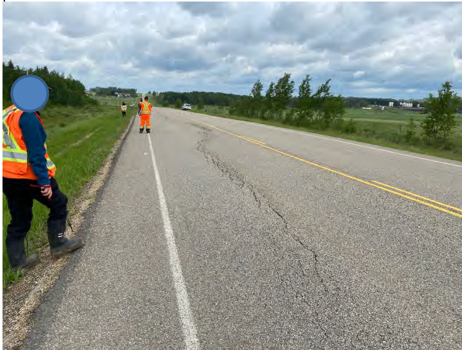
Photo 1: West limits of WBL pavement cracks. Approx. 25 mm dip. Looking east.
