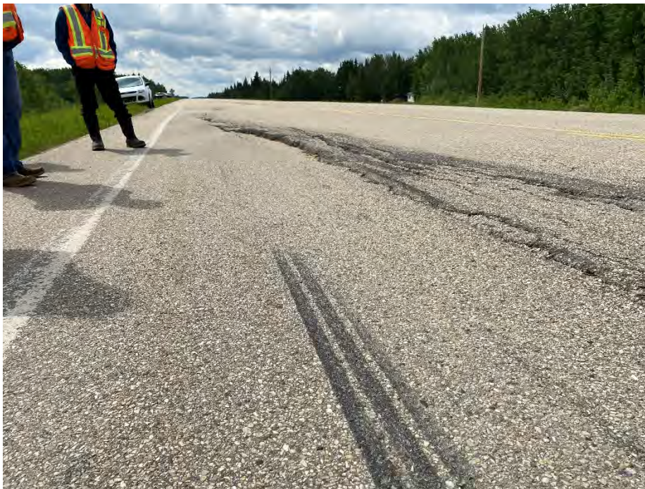
Photo 4: Pavement cracking on EBL with tire marks. Looking west.
