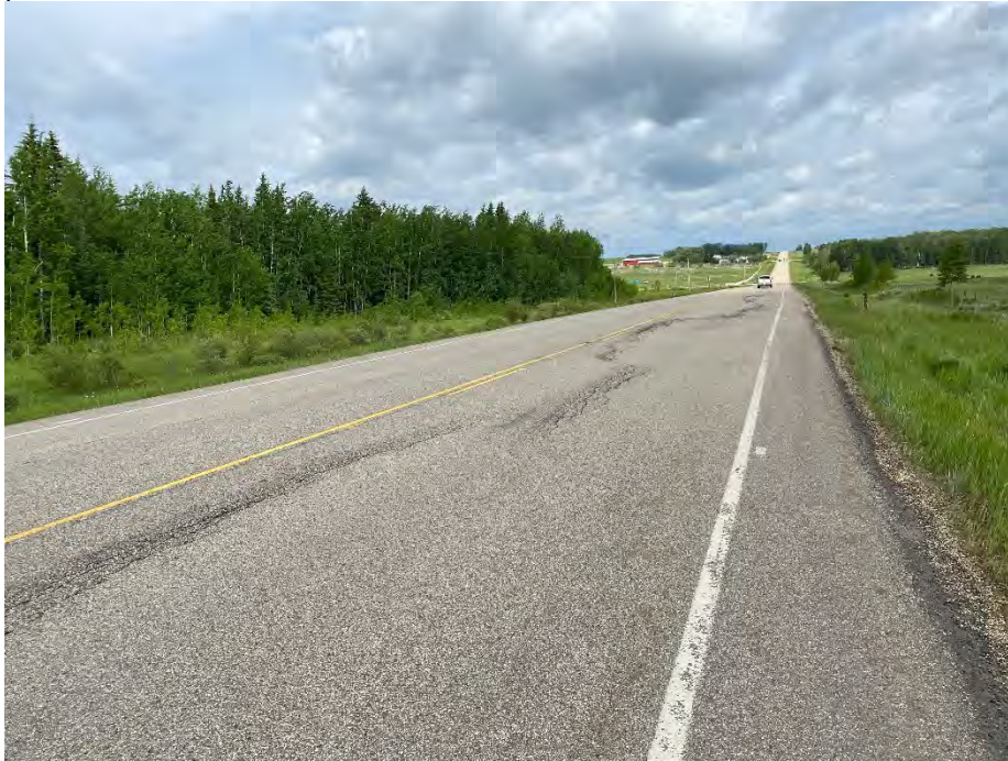
Photo 3: Pavement cracking on EBL. Looking east.
