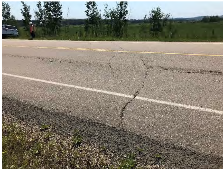
Photo 2: Diagonal pavement cracks approximately at km 2.55. Looking southeast.
