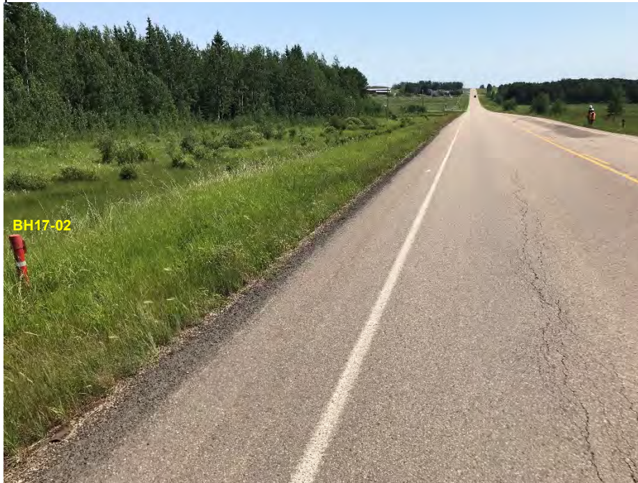
Photo 3: Faint cracks progressing east of BH17-02. Looking east.
