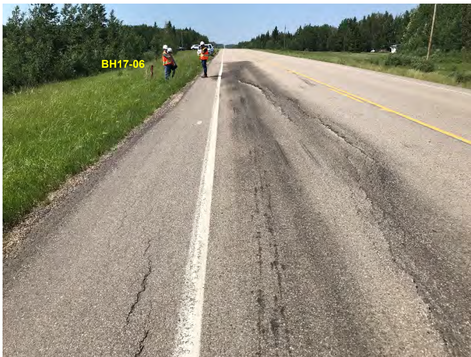
Photo 4: Pavement cracking on EBL. 70 mm to 90 mm differential. Tire marks apparent at drop location. Looking west.
