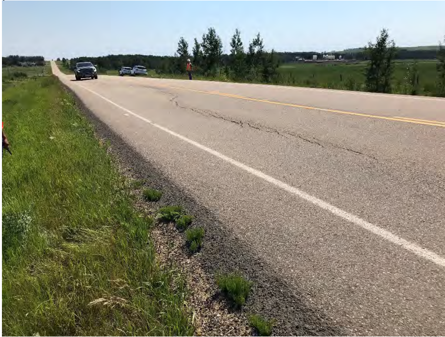
Photo 1: West limits of WBL pavement cracks. Approx. 25 mm dip. Looking southeast.
