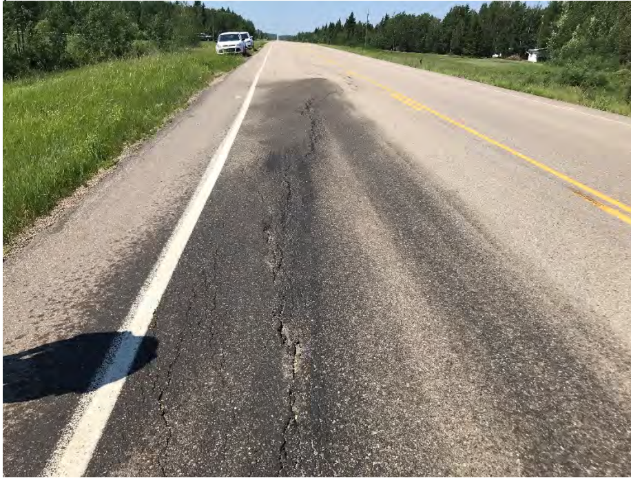
Photo 5: Pavement cracking on WBL with tire marks. Looking west.
