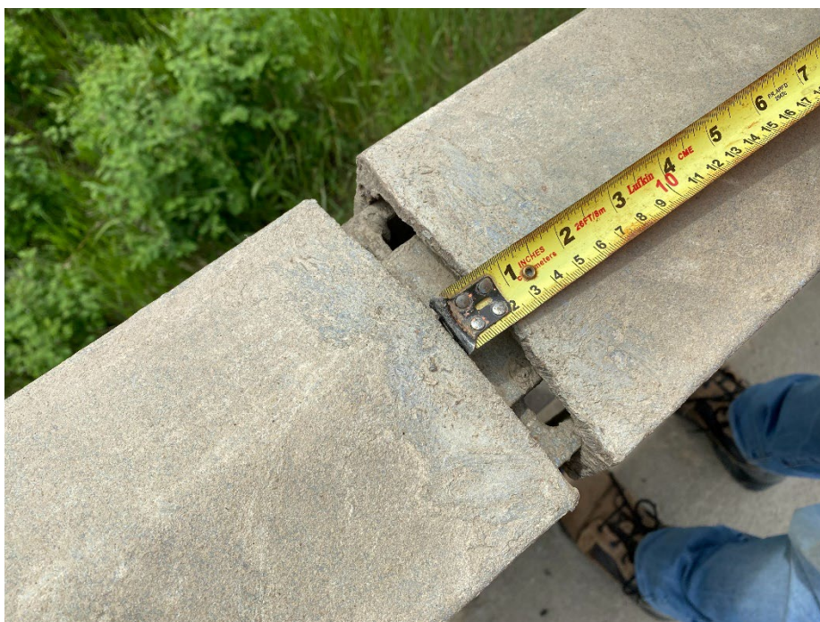
Photo 4: Guardrail separation at southwest corner of bridge. Looking southwest.
