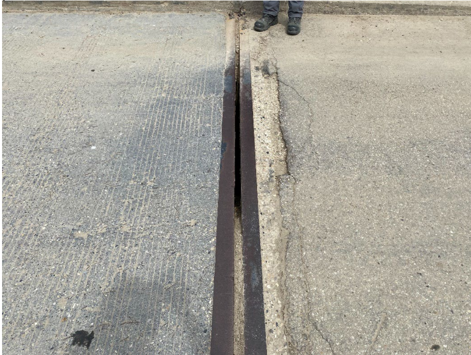
Photo 5: Gap at expansion joint with rubber falling out. Looking north.
