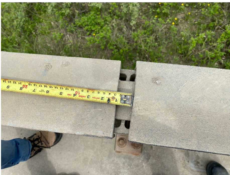
Photo 2: Guardrail separation at northeast corner of bridge. Looking north.
