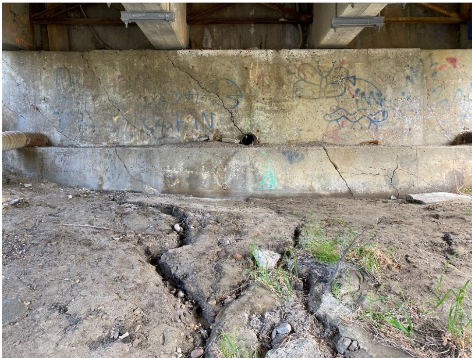
Photo 6: Cracking of east abutment and gullies on headslope. Looking east.
