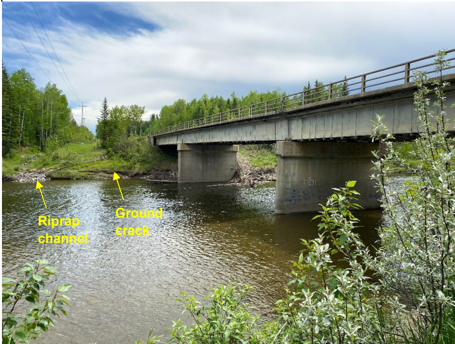
Photo 9: Riprap lined channel and ground crack north of east abutment. Looking east.
