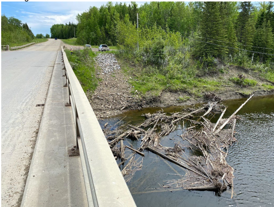
Photo 10: Riprap placed south of bridge along previous erosion channel. Driftwood collected near the east pier. Looking southeast.
