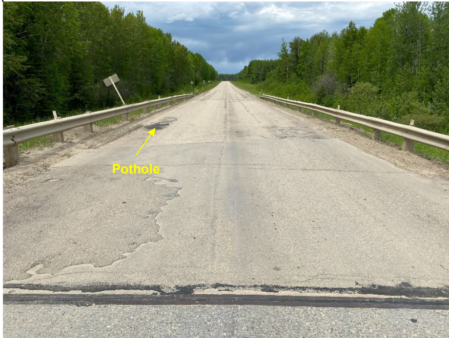
Photo 11: Pavement surface at west abutment. Looking northwest.
