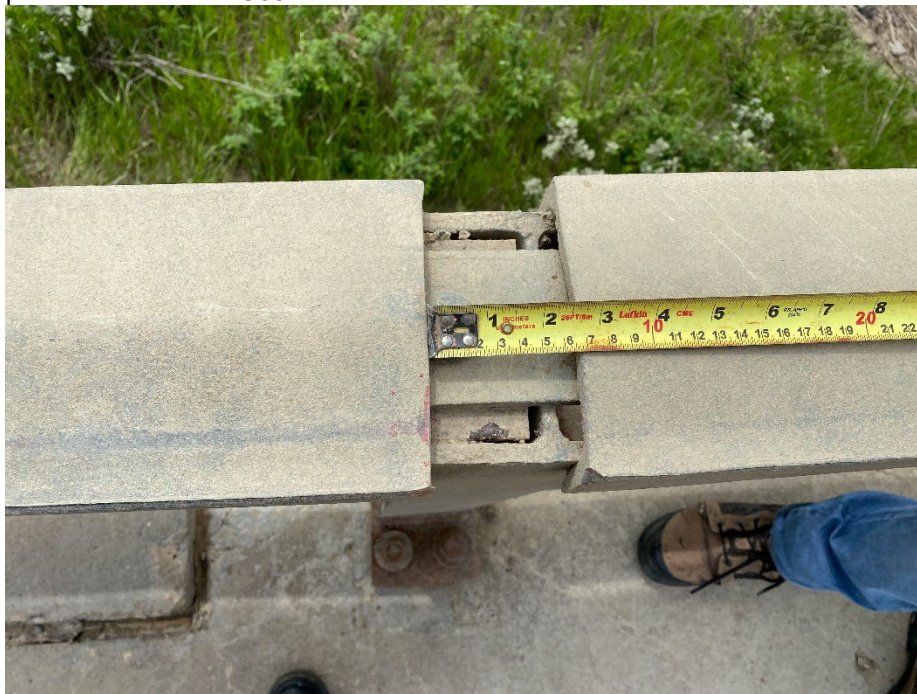
Photo 1: Guardrail separation at southeast corner of bridge. Looking south.
