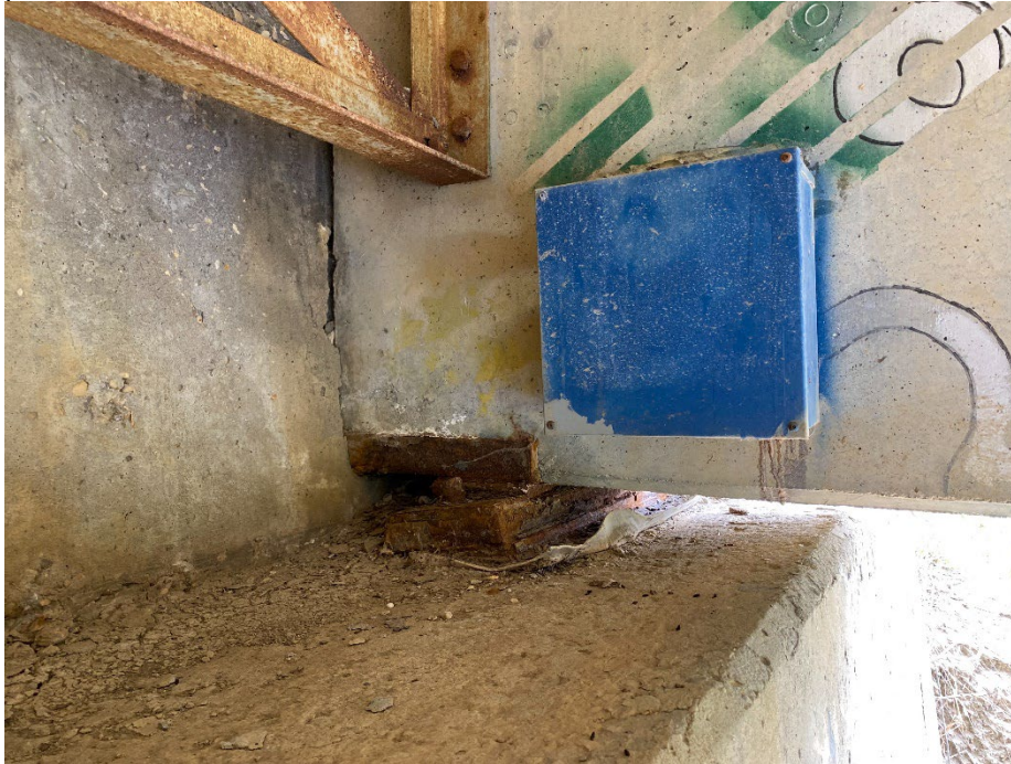
Photo 7: Girders in contact with east abutment. Movement of bearing plate. Looking south.
