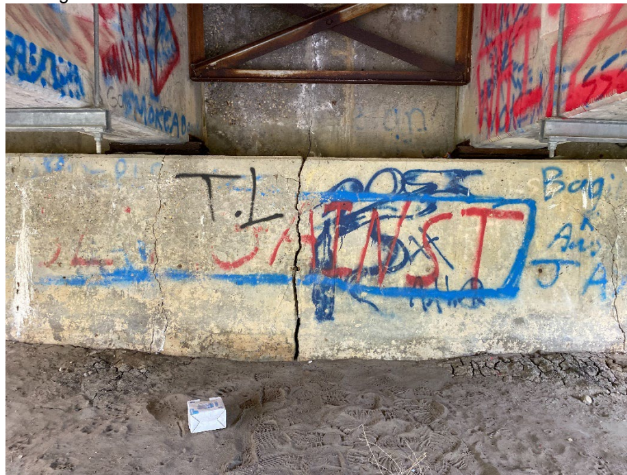
Photo 8: 20 mm crack at west abutment. Looking west.
