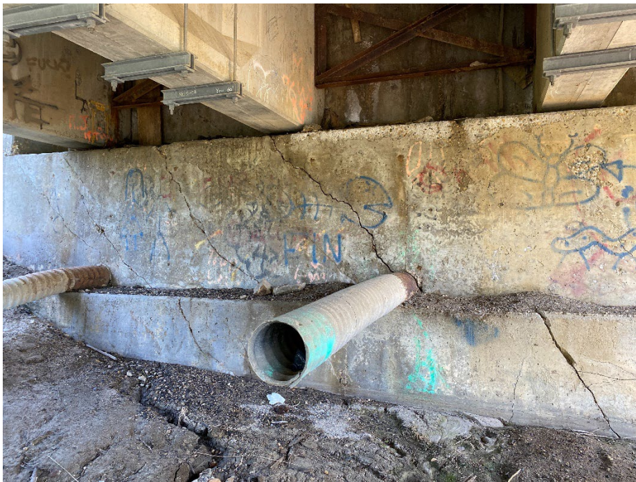
Photo 6: Cracking of east abutment. Looking northeast.
