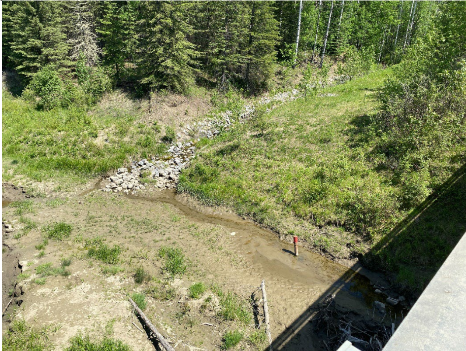
Photo 9: Riprap lined channel north of east abutment. Ground cracks near SI14-01. Looking northeast.
