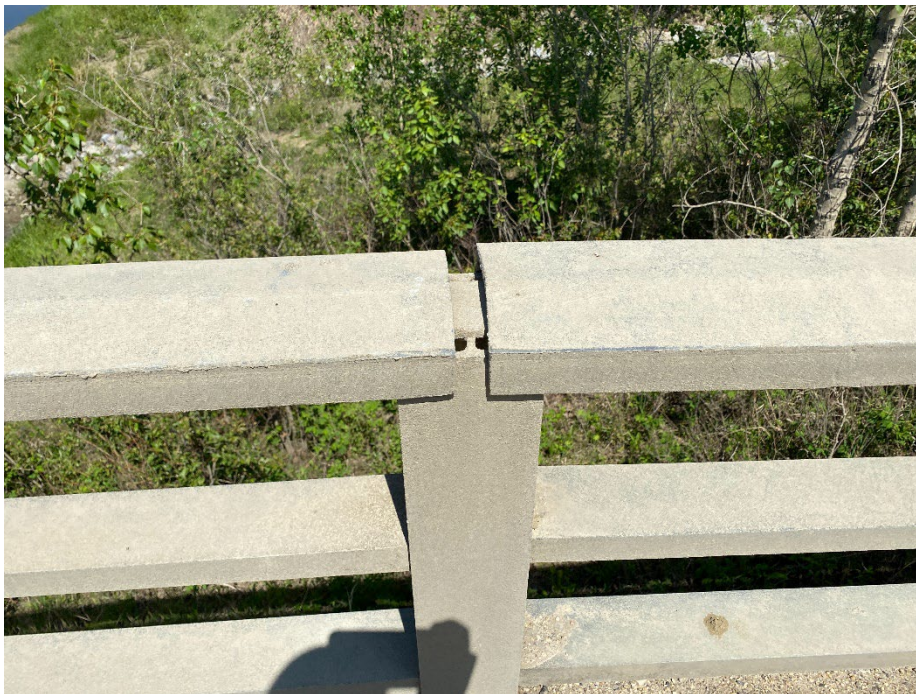
Photo 2: Guardrail separation at northeast corner of bridge. Looking north.
