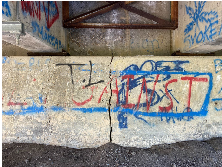
Photo 8: 20 mm crack at west abutment. Looking west.
