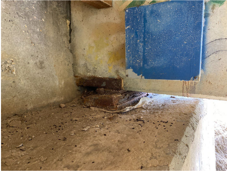
Photo 7: Girders in contact with east abutment. Movement of bearing plate. Looking south.
