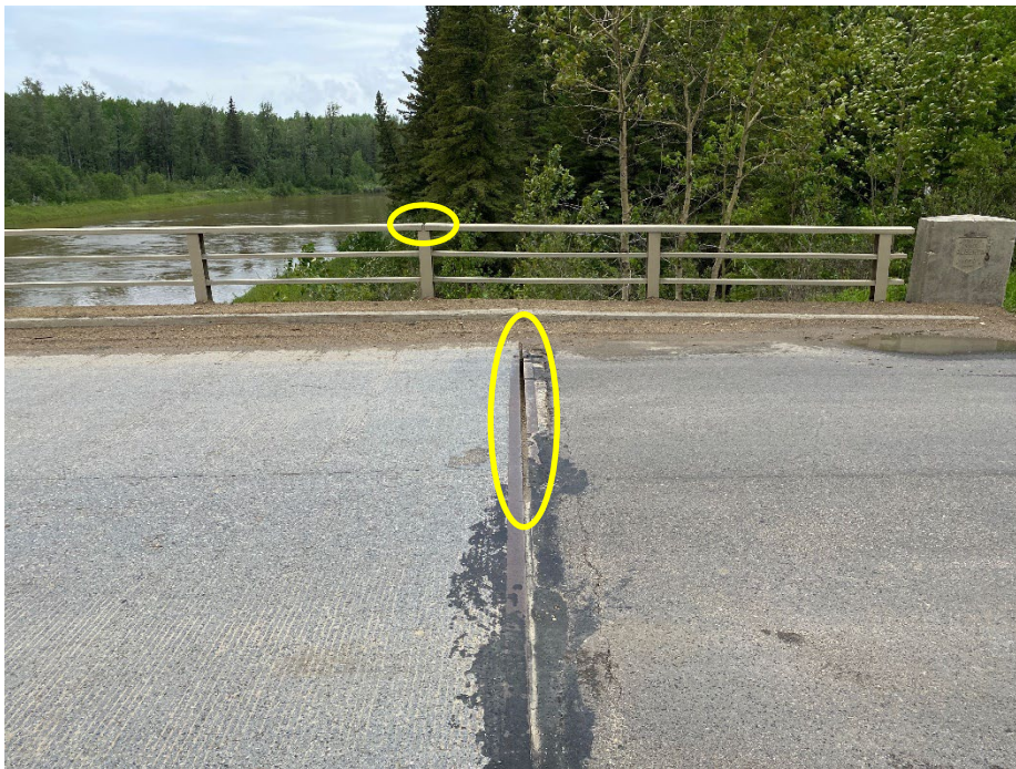
Photo 2: Guardrail separation at northeast corner of bridge and gap in expansion joint. Looking north.
