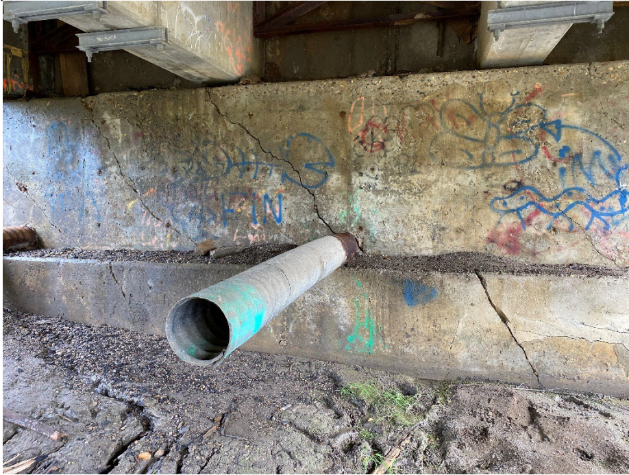
Photo 5: Cracking of east abutment. Looking northeast.
