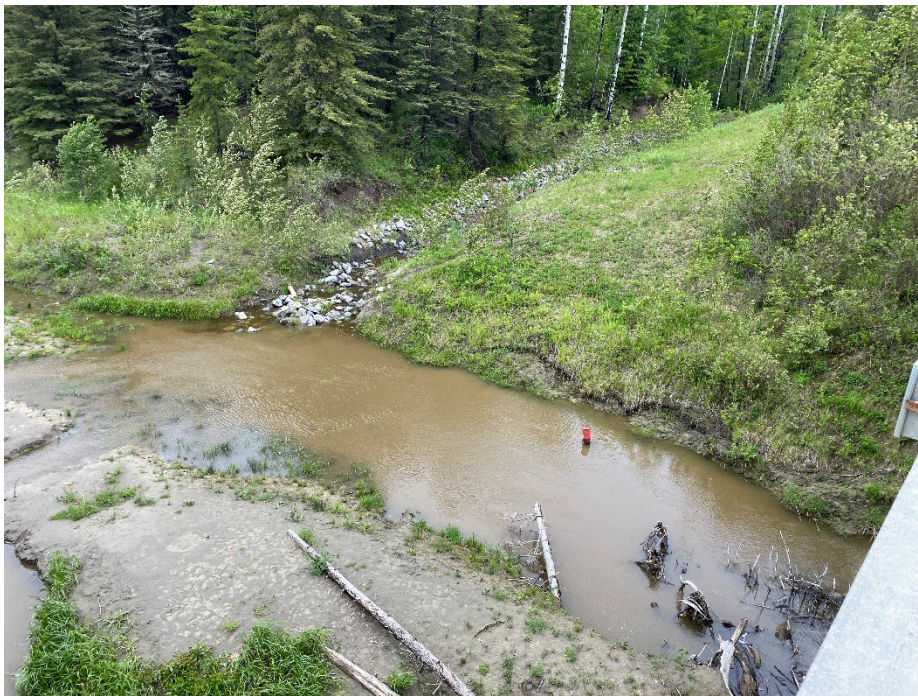
Photo 8: Riprap lined channel north of east abutment. Ground cracks near S114-01. Looking northeast.
