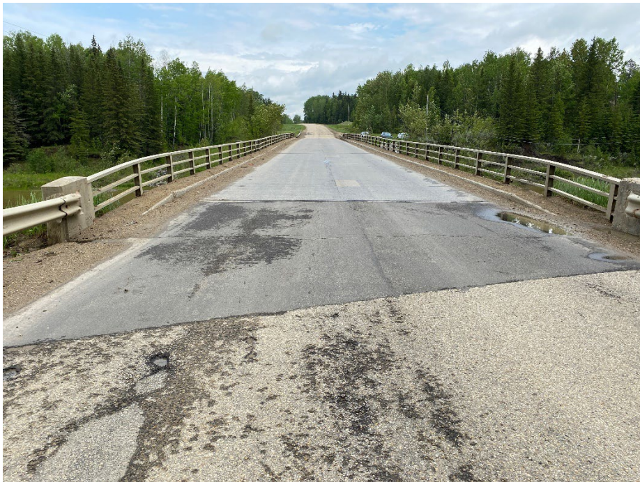
Photo 10: Pavement surface at west abutment. Looking east across bridge.
