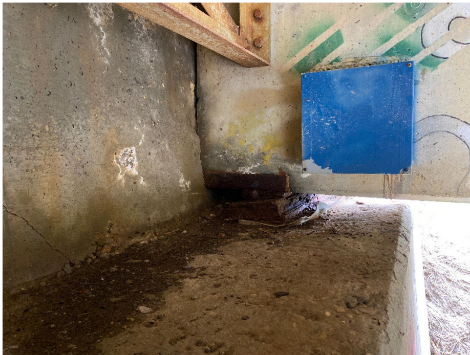
Photo 6: Girders in contact with east abutment. Movement of bearing plate. Looking south.
