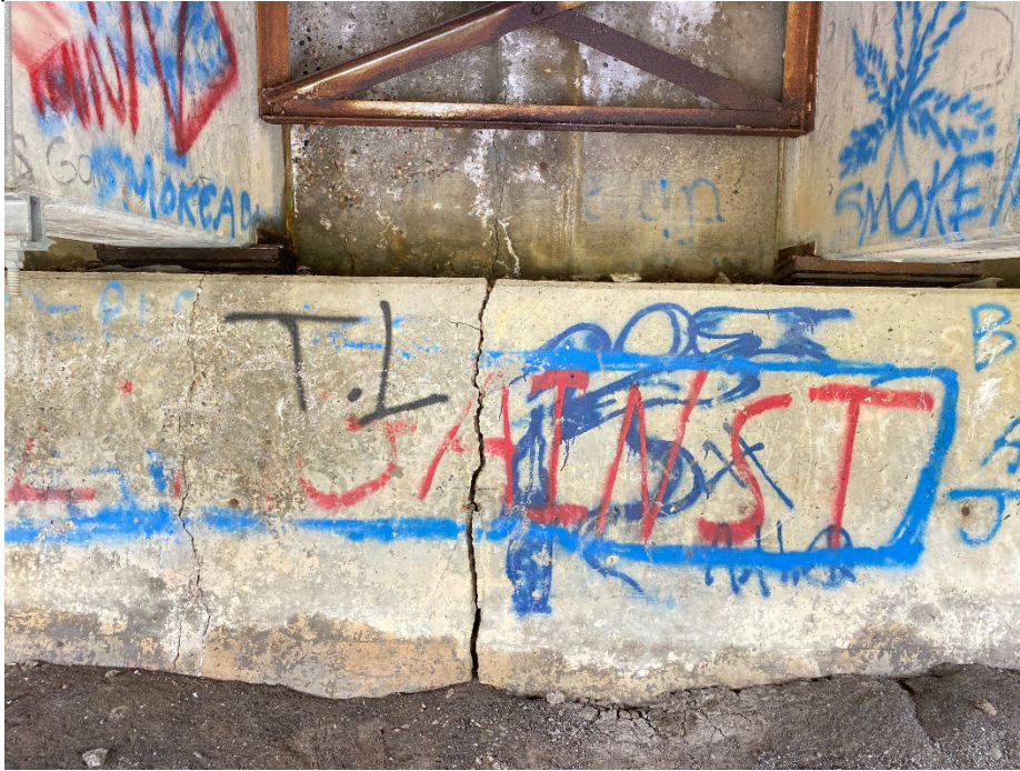
Photo 7: 20 mm crack at west abutment. Looking west.
