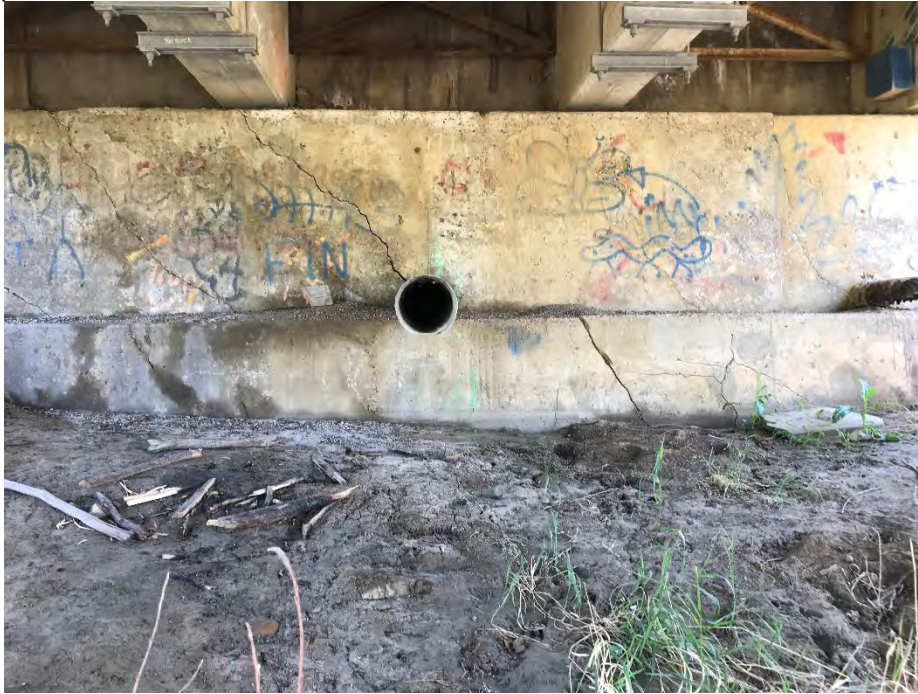
Photo 5: Cracking of east abutment. Looking east.
