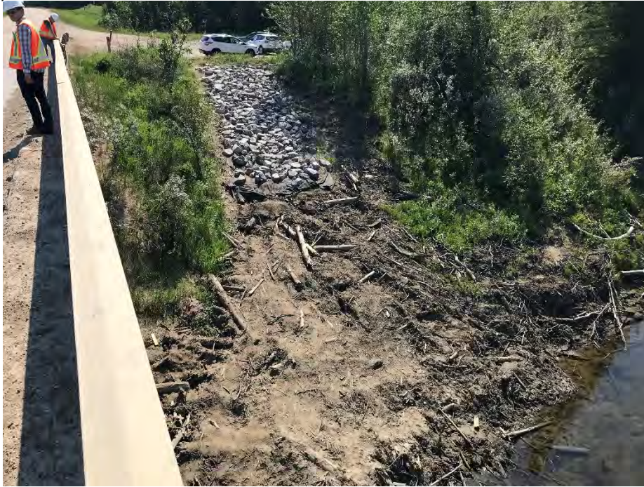
Photo 9: New riprap placed south of bridge along previous erosion channel. Looking southeast.
