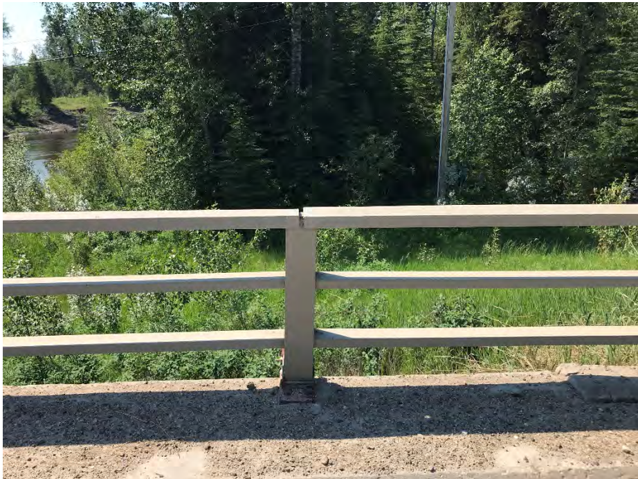
Photo 4: Guardrail separation at southwest corner of bridge. Looking south.
