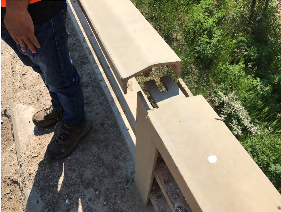
Photo 1: Guardrail separation at southeast corner of bridge. Looking southeast.
