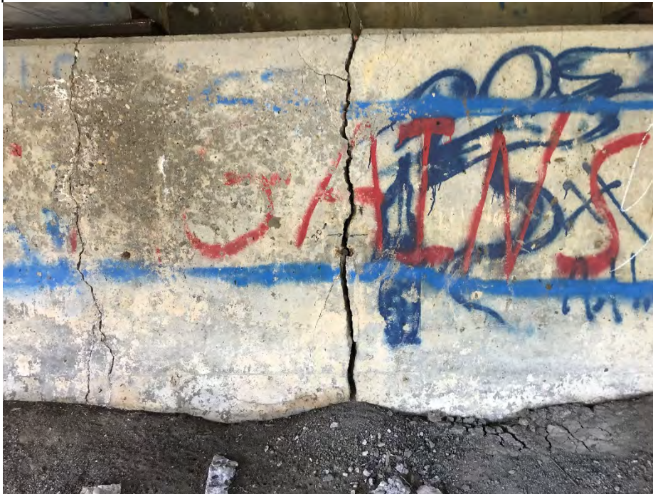
Photo 7: 20 mm crack at west abutment. Looking west.
