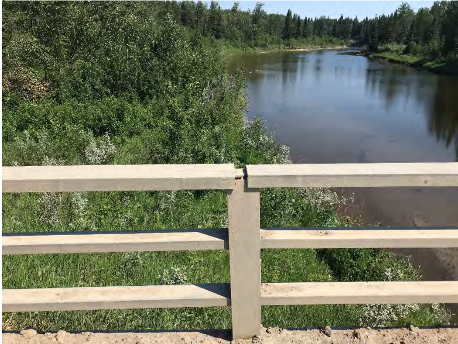
Photo 3: Guardrail separation at northwest corner of bridge. Looking north.
