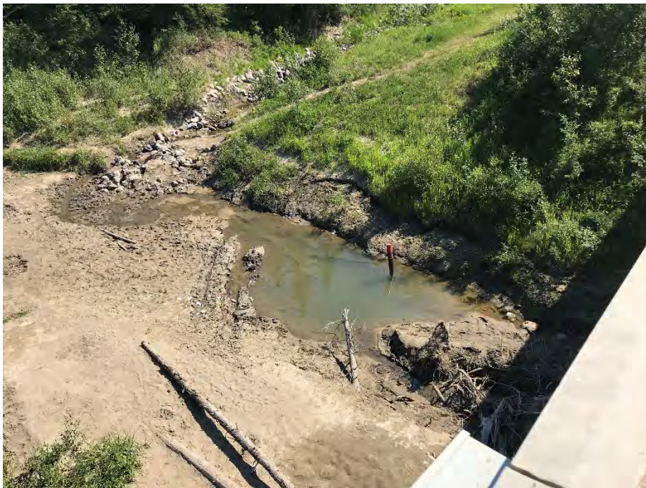
Photo 8: Riprap lined channel north of east abutment. Ground cracks near SI14-01. Looking northeast.
