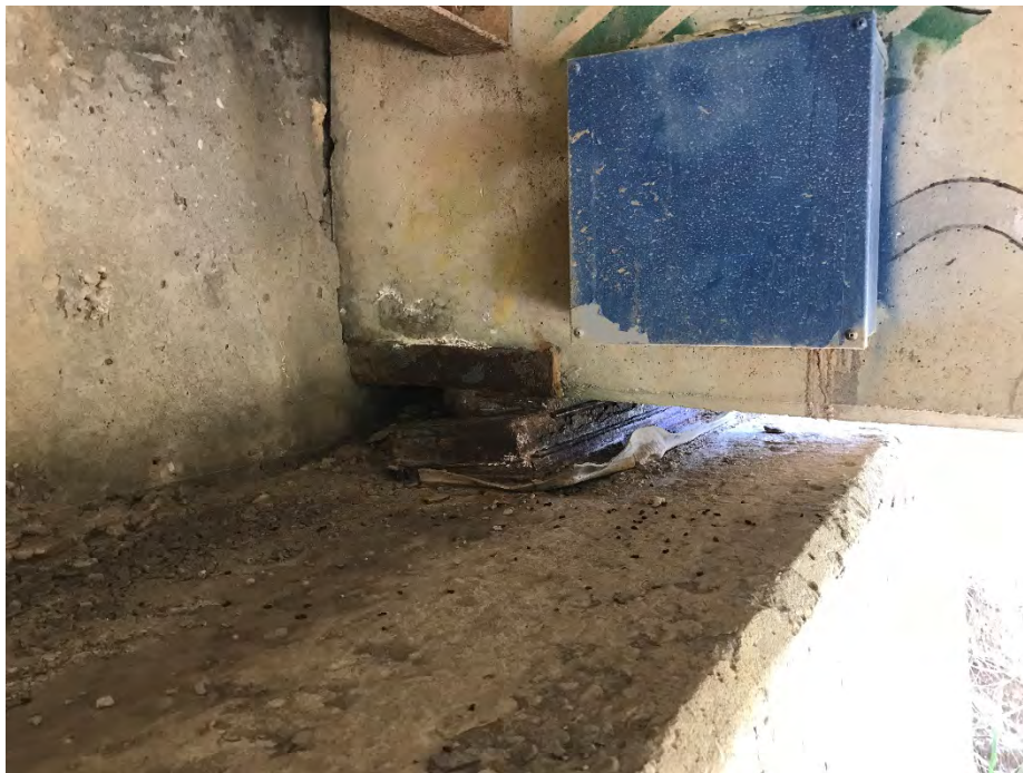
Photo 6: Girders in contact with east abutment. Movement of bearing plate. Looking south.
