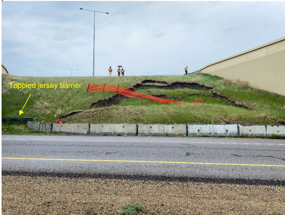
Photo 1: Slump on south embankment. Looking southwest.
