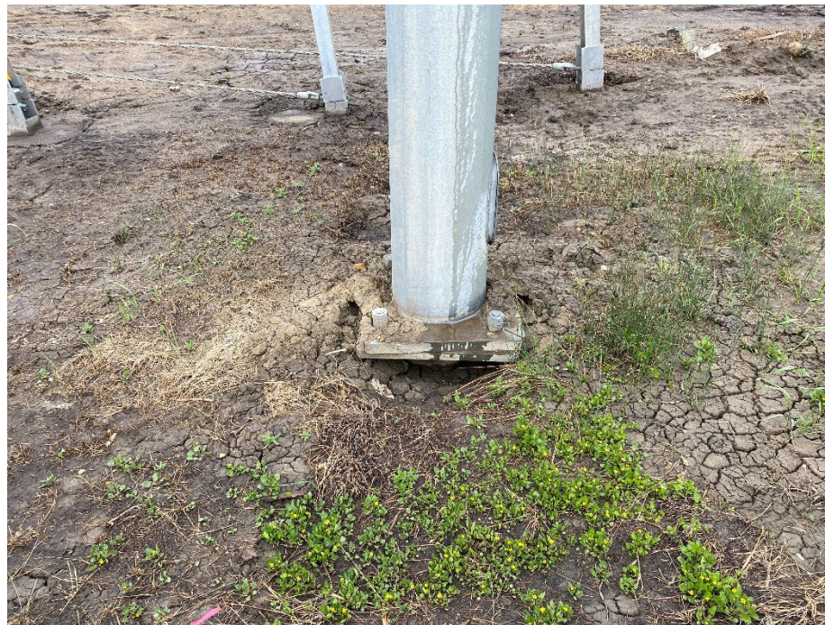
Photo 8: Scouring/settlement of ground around the light standard closest to the embankment. Looking west.
