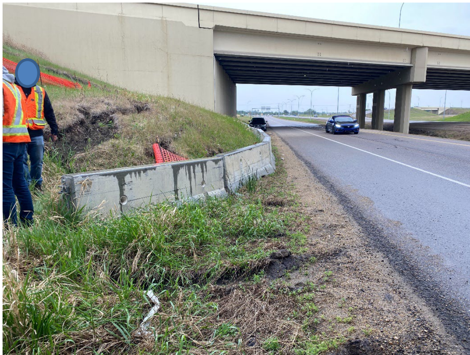
Photo 4: Toe bulge of slump with scarping/cracking. Looking northwest.
