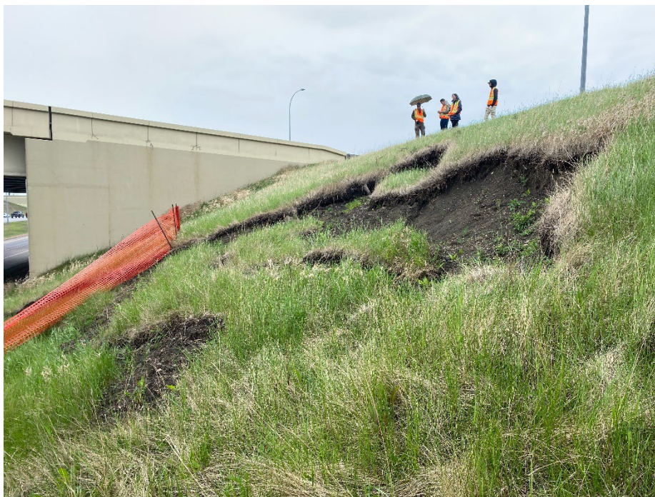
Photo 6: Retrogressing scarps near top of slump. Looking southeast.
