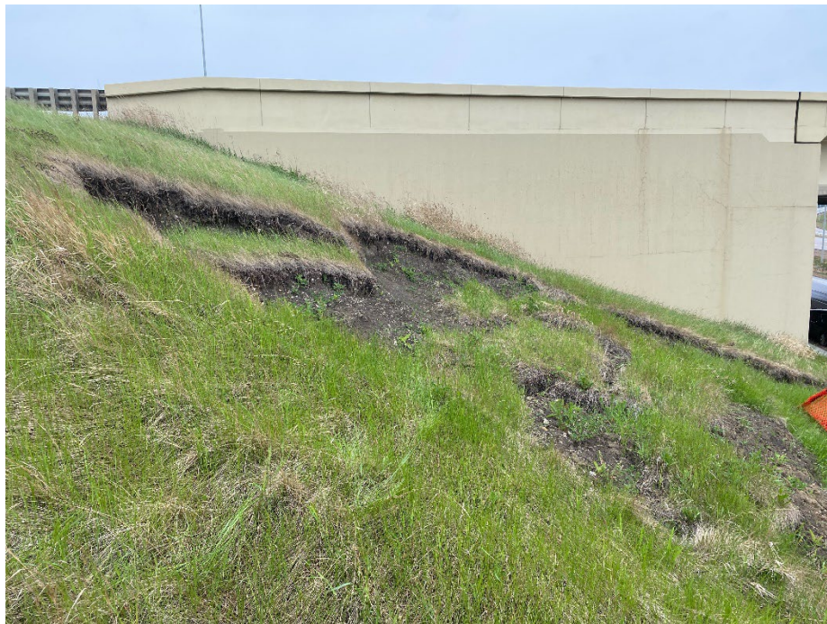
Photo 2: Slump on south embankment. Looking west.
