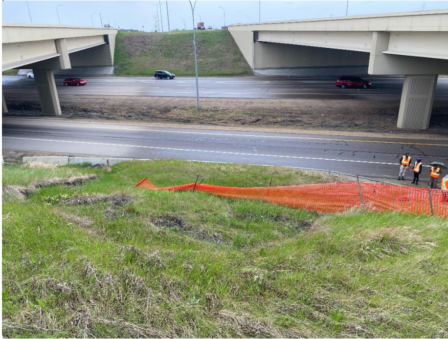
Photo 7: Slumping viewed from the crest of the embankment. Looking north.
