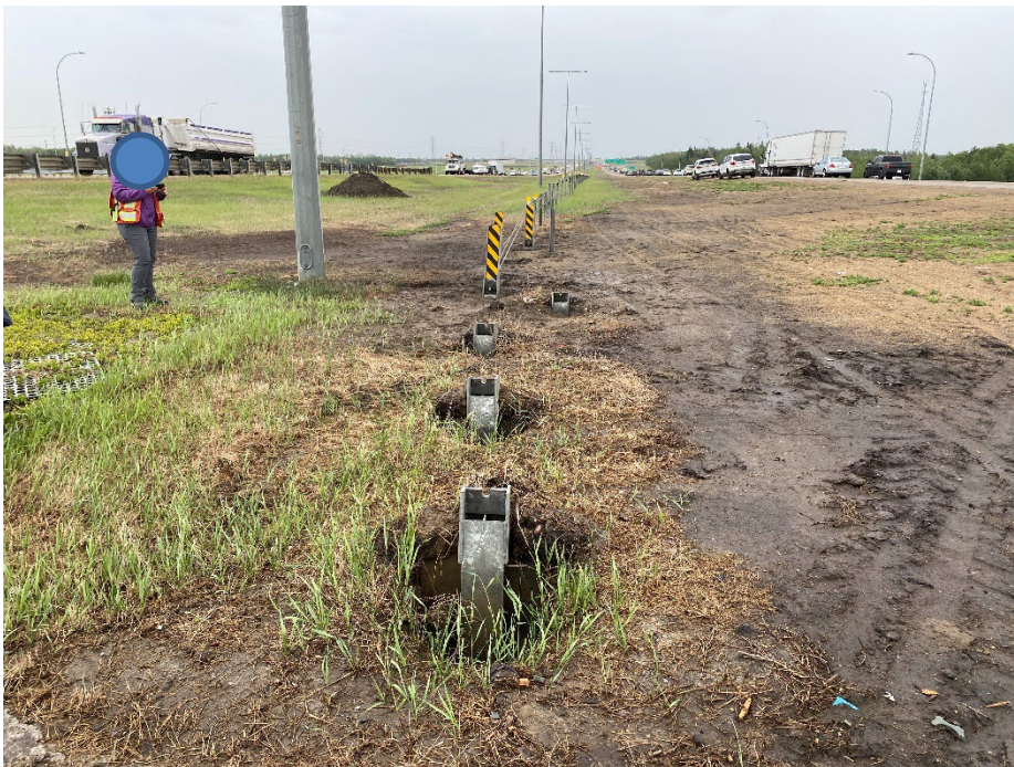
Photo 10: Abandoned posts for high tension cable barrier. Looking south.
