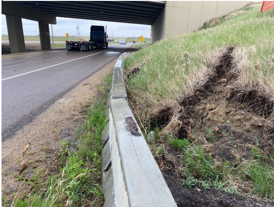
Photo 5: Toe of the embankment/slump. Looking southeast.
