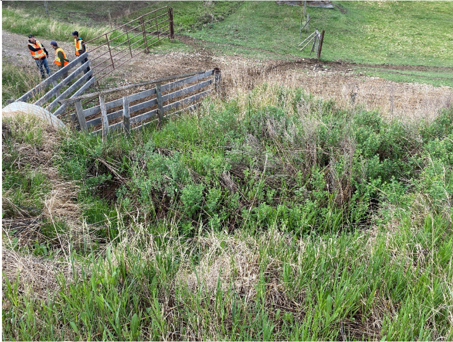
Photo 5: West slump next to culvert entrance. Looking south.
