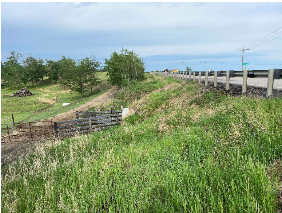
Photo 2: Slump across cattlepass culvert. Looking west
