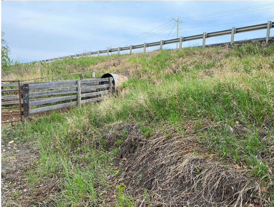
Photo 1: Slump and toe bulge at east side of cattlepass culvert. Looking northwest
