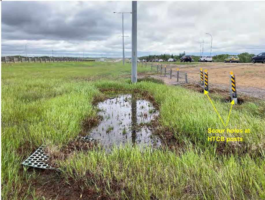
Photo 9: Ponding water at top of embankment. Looking south.
