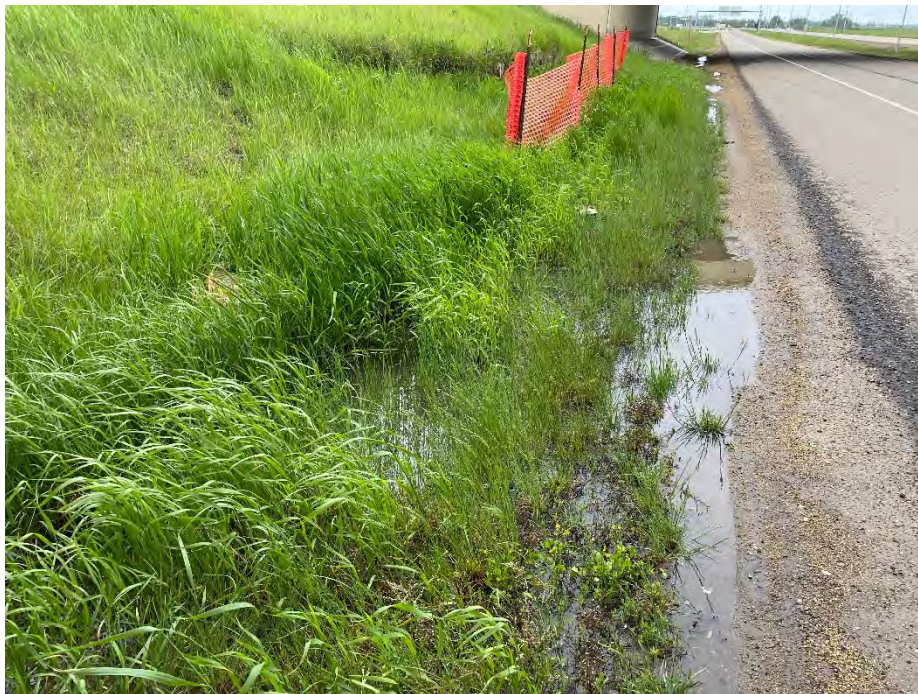
Photo 4: Ponded water on east side of embankment toe. Looking west.
