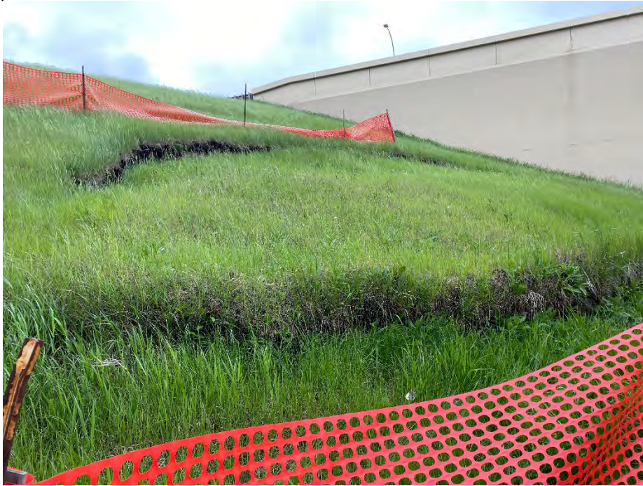
Photo 3: Slump on south embankment. Looking southwest.
