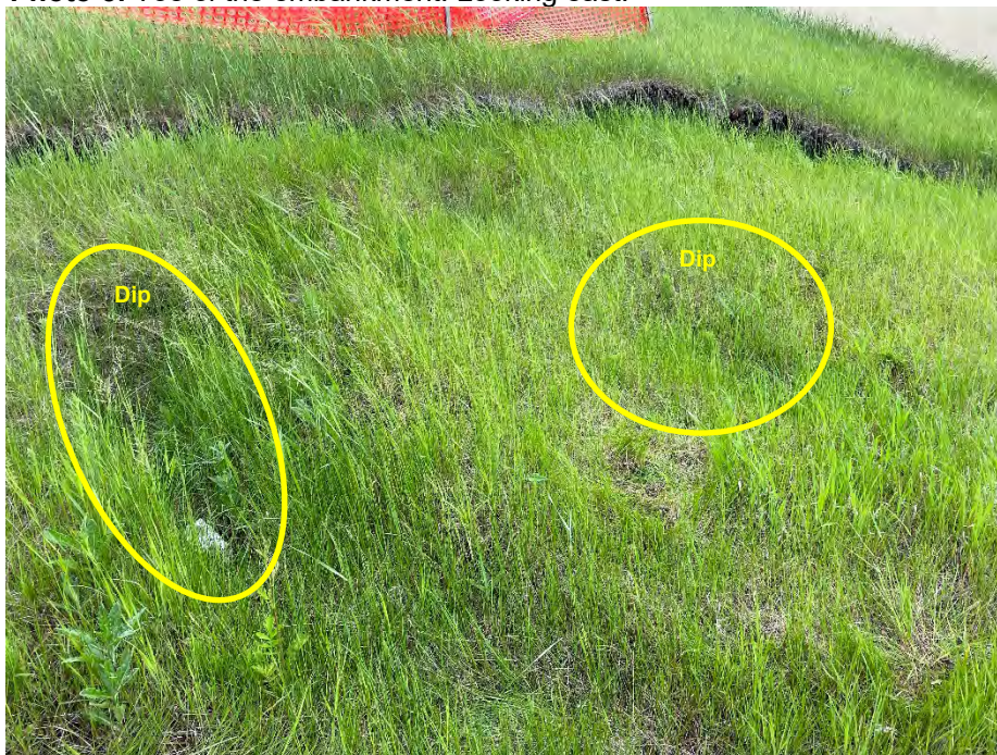
Photo 6: Dips in the ground below top of slump. Looking southwest.
