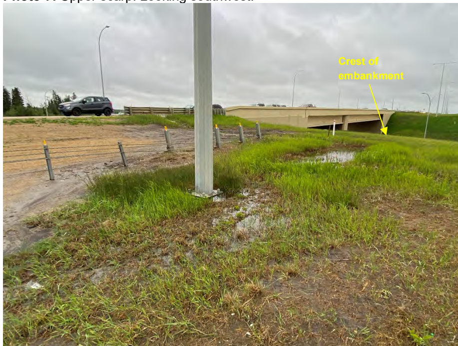
Photo 8: Water ponding at the top of the embankment. Looking northwest.
