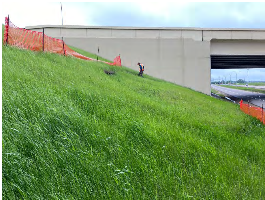
Photo 2: Slump on south embankment. Looking west.
