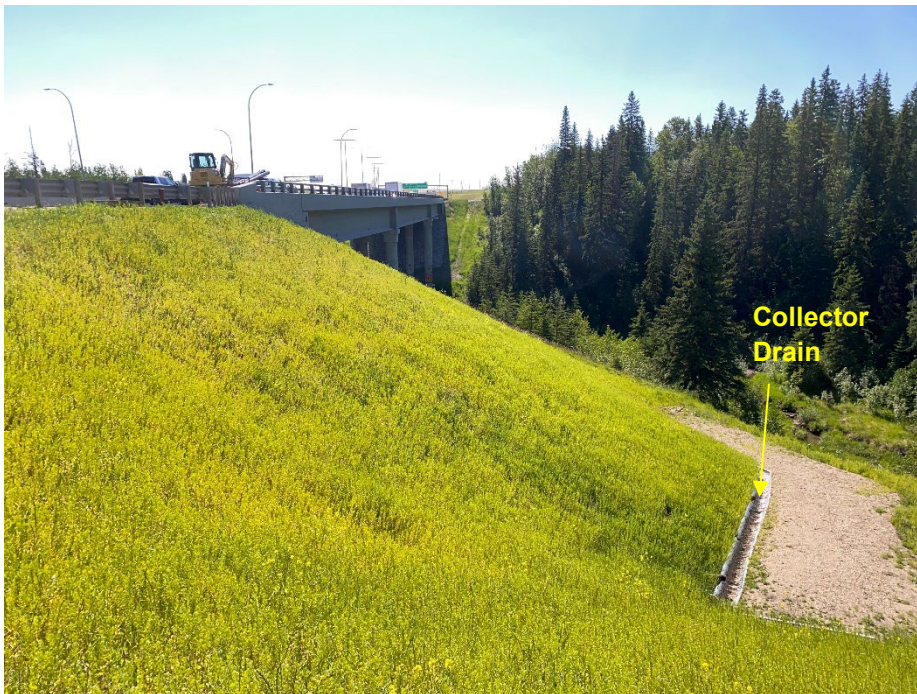
Photo 2: Soil nailed slope at north and south slide area, collector drain installed at toe of repaired slope. Looking southeast.
