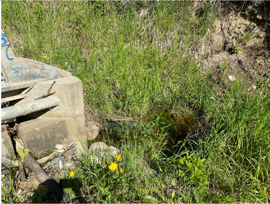
Photo 7: Water from separated pipe eroding the creekbank north of the west outfall. Looking north.
