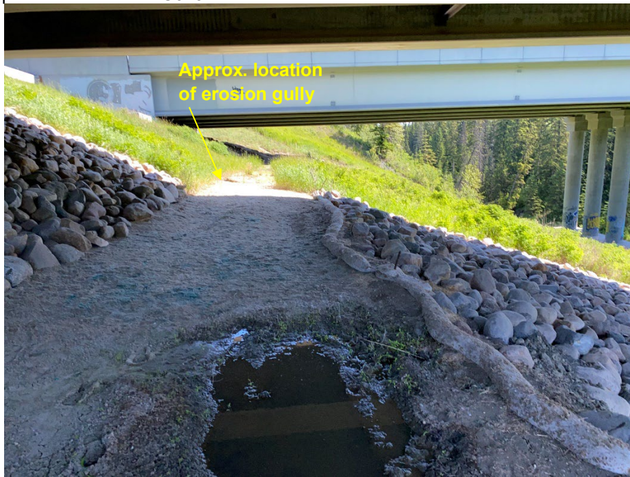
Photo 5: Erosion and ponded water on footpath near NW abutment for SBL. Looking northeast.
