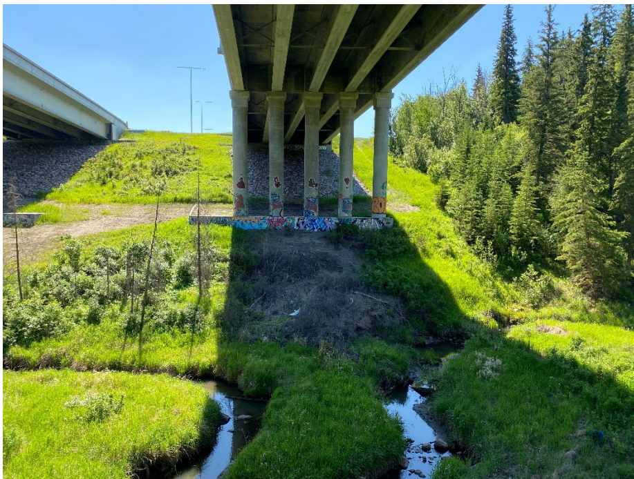
Photo 12: Dead vegetation on east bank below the AH southbound pedestal. Looking southeast.
