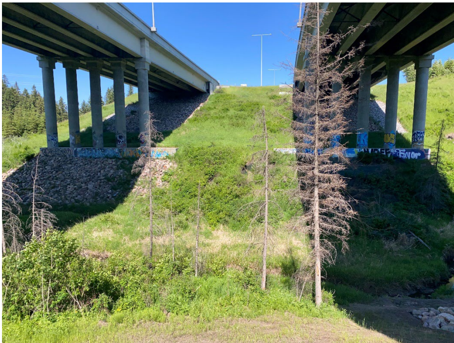
Photo 10: West slope with two slumps between pedestals and erosion mat exposed below northernmost pedestal. Looking northwest.
