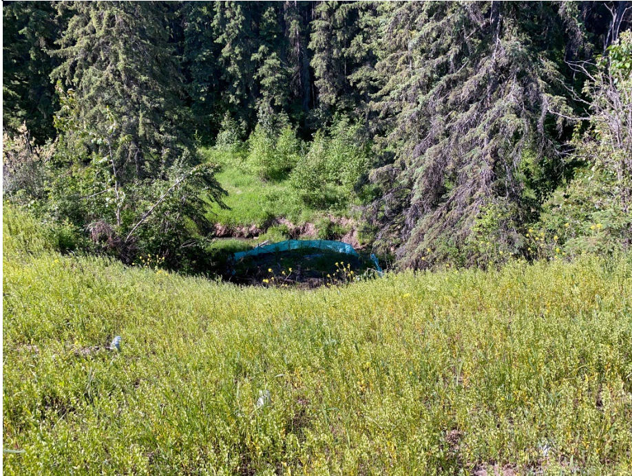
Photo 3: Repaired debris chute below soil nailed area north slide area. Looking southwest.
