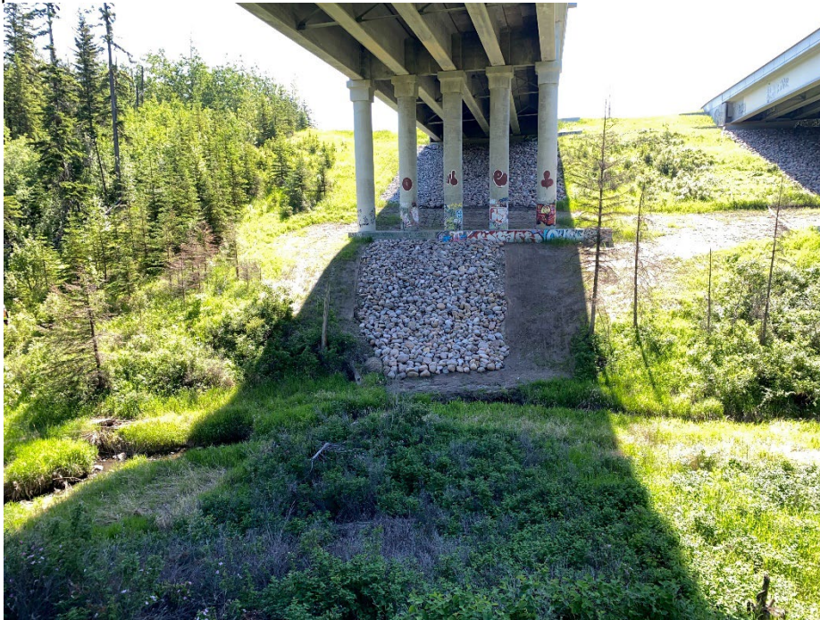
Photo 11: Repaired slope failure on east bank below AHD northbound pedestal. Looking southeast.
