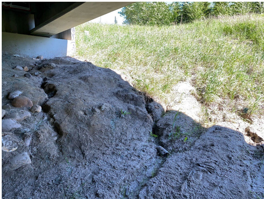
Photo 6: Erosion gullies at the north corner of NW abutment. Looking northwest.
