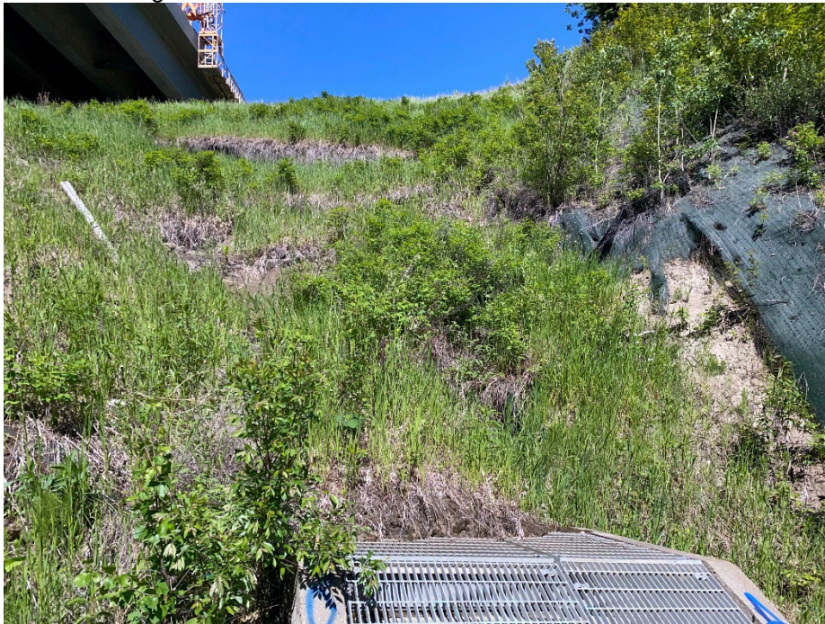
Photo 8: Erosion above west outfall. Looking west.
