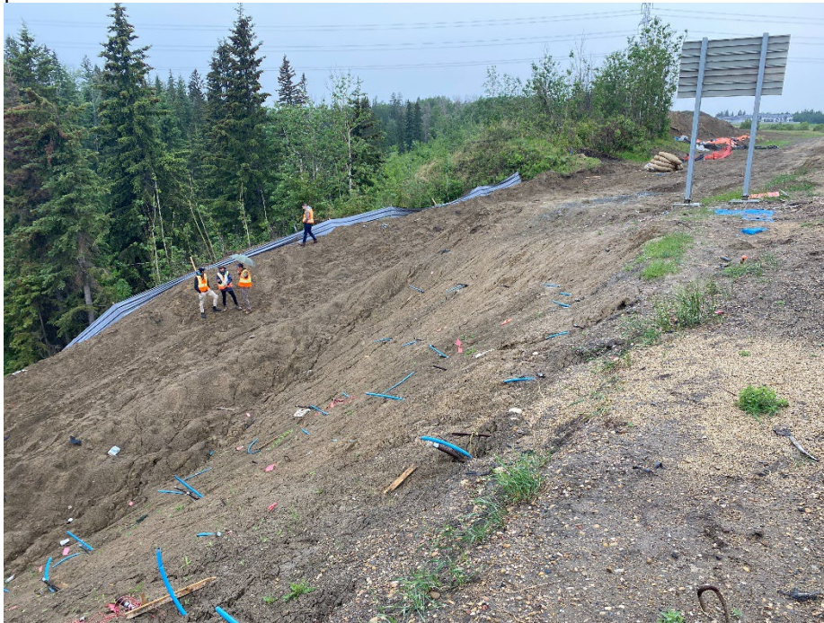
Photo 1: Soil nailed slope at north and south slides. Looking northwest.
