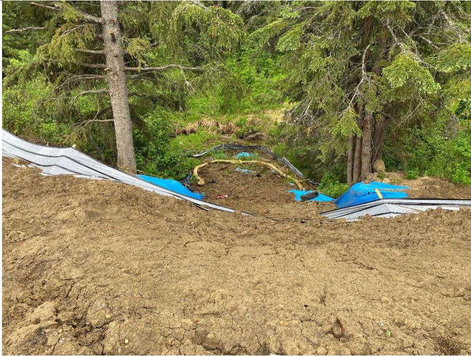
Photo 3: Debris chute below soil nailed area north slide area, repairs ongoing. Looking southwest.
