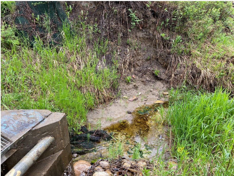
Photo 6: Water from separated pipe eroding the creekbank north of the west outfall. Looking northeast.
