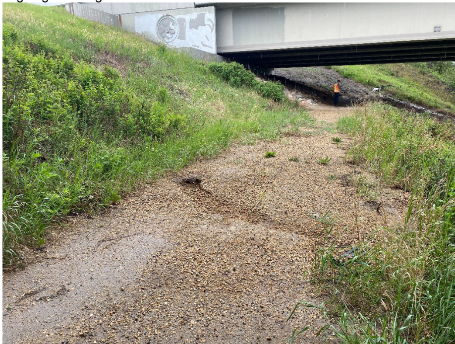
Photo 4: Erosion on footpath near NW abutment for SBL. Looking northeast.
