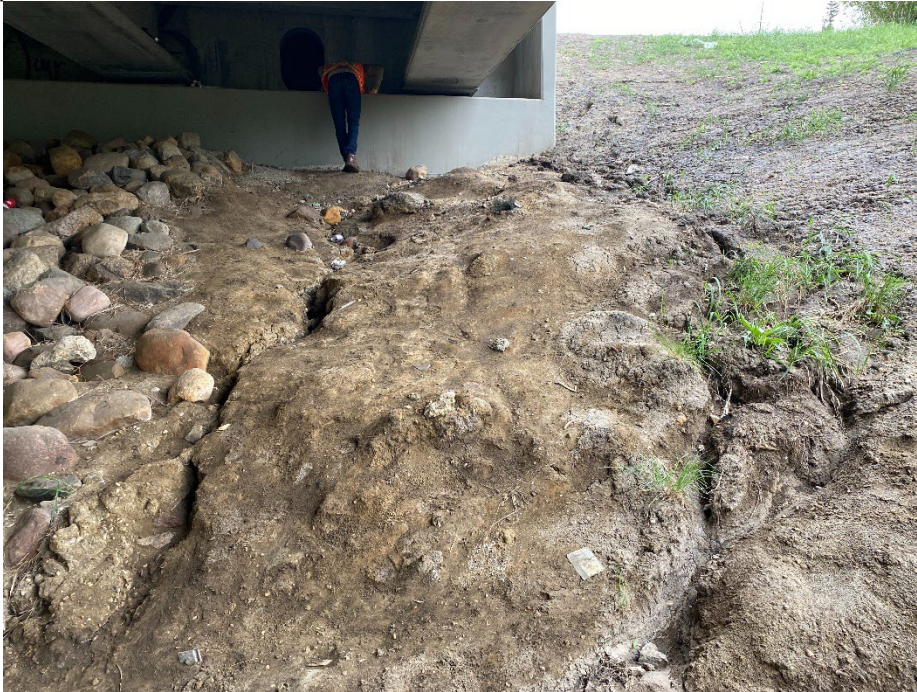
Photo 5: Erosion gullies at the north corner of NW abutment. Looking northwest.
