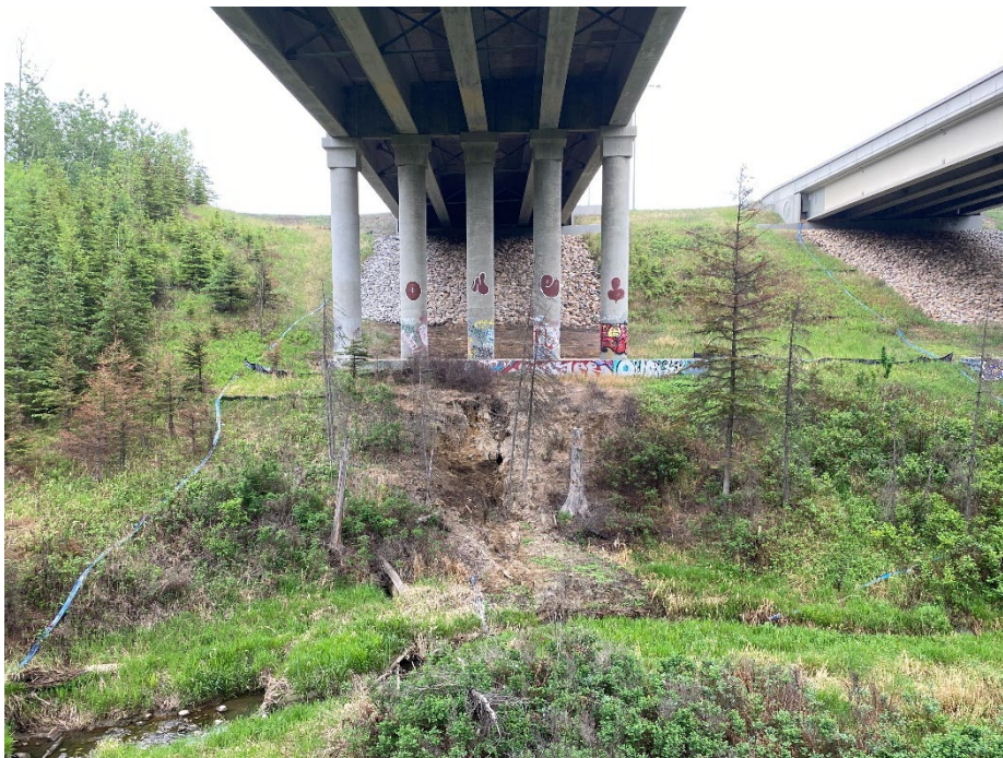
Photo 10: Slope failure on east bank below AHD NB pedestal. Looking southeast.
