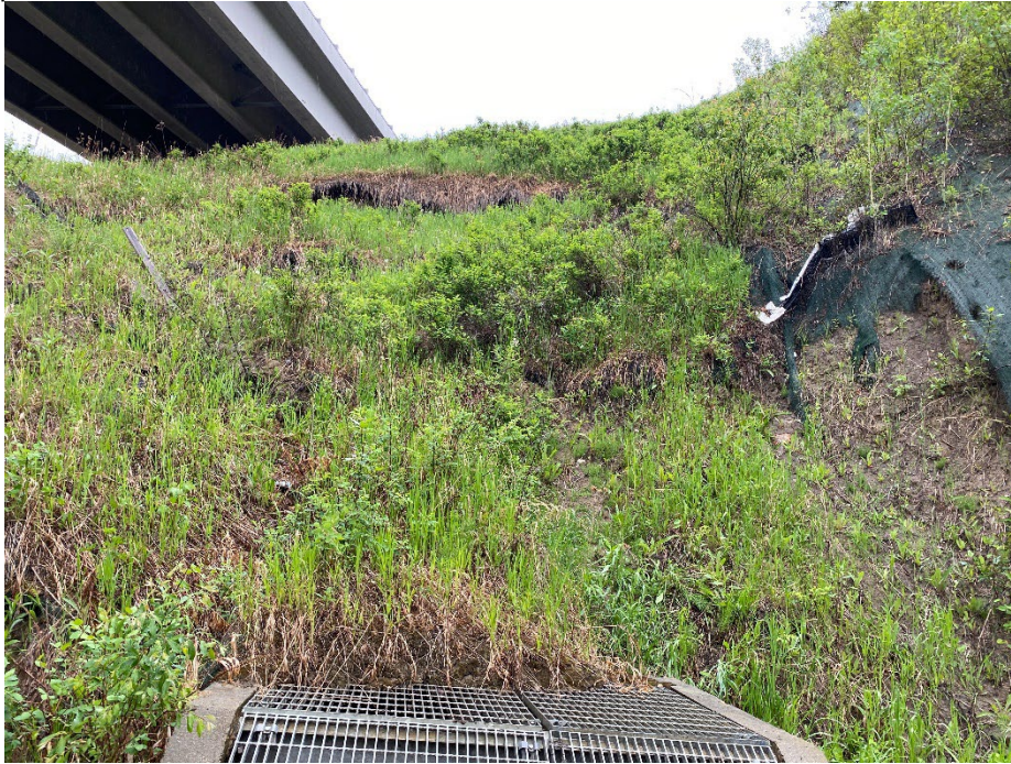
Photo 7: Erosion above west outfall. Looking west.
