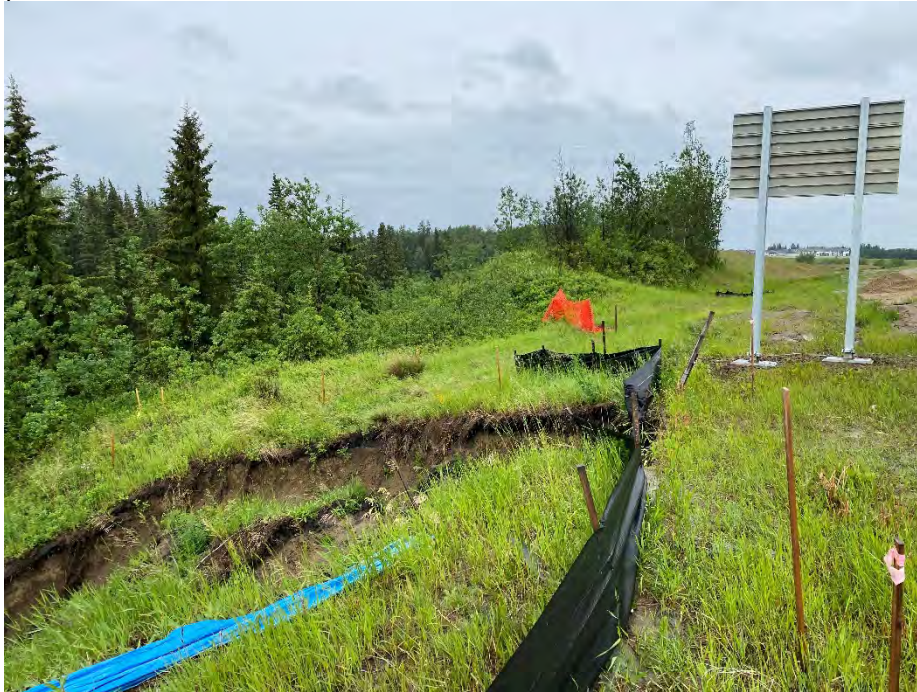
Photo 1: Distance from edge of scarp to sign pedestal is 2.6 m. Looking northwest.
