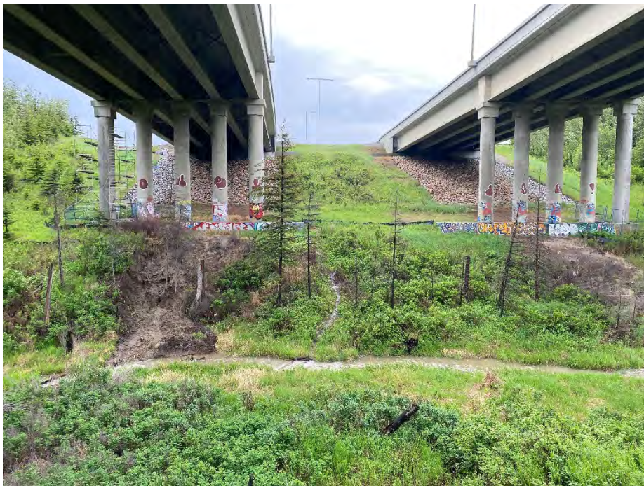
Photo 10: Slope failure on east bank below AHD NB pedestal, erosion below AHD SB pedestal. Looking southeast.
