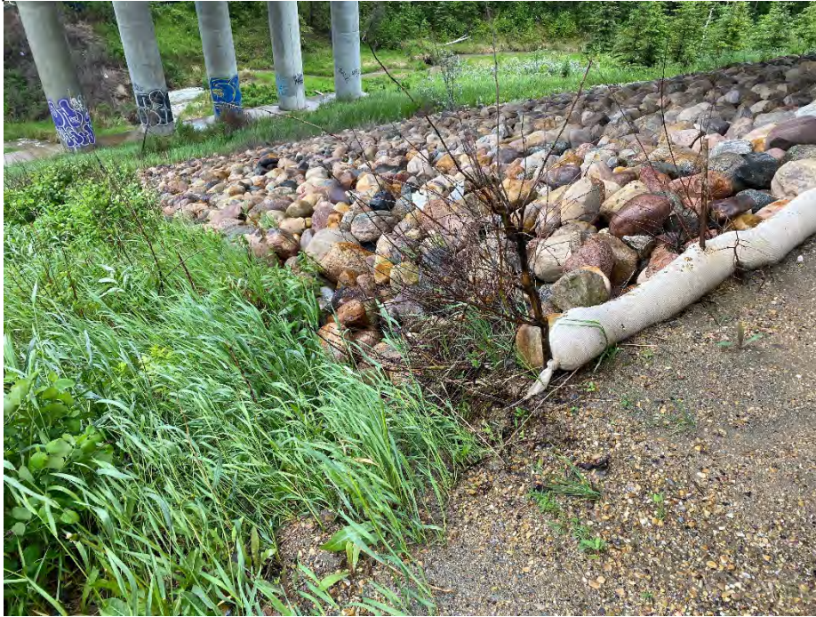
Photo 5: Erosion/slump retrogressed to footpath, increasing vegetation from 2021. Looking southeast.
