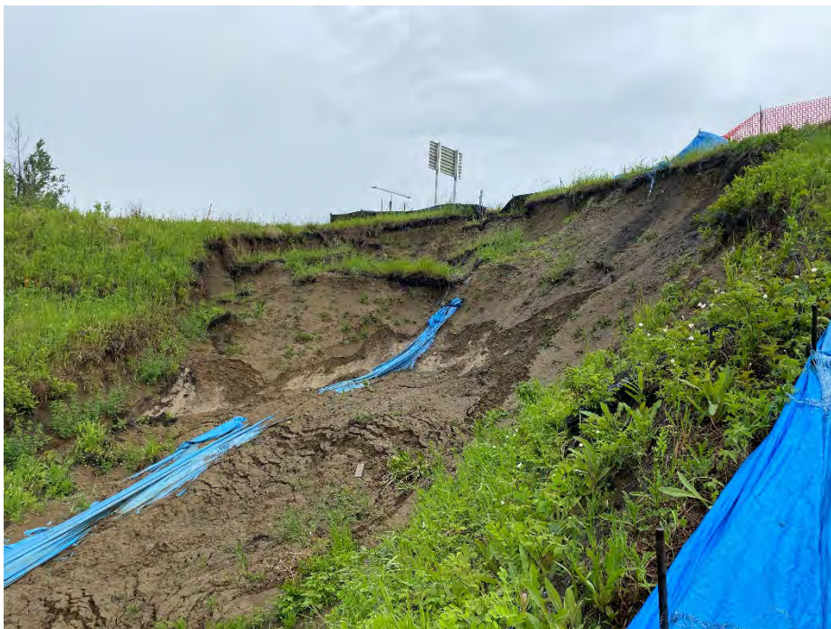
Photo 2: North slide. Looking north from midslope.
