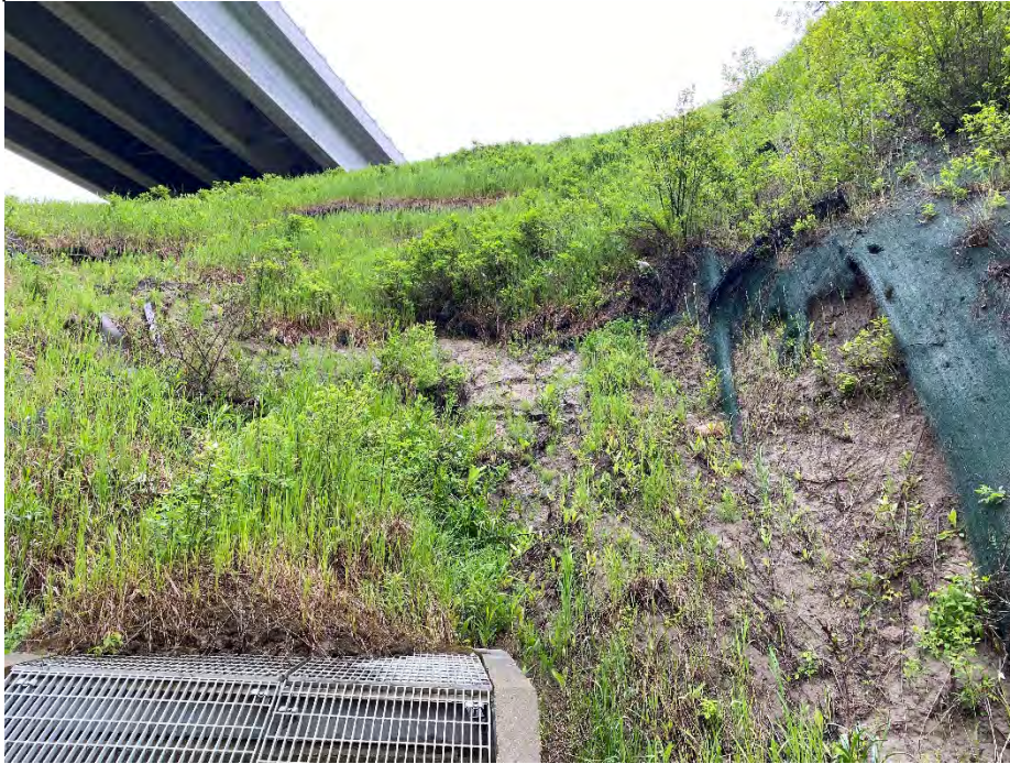
Photo 7: Erosion above west outfall. Looking west.
