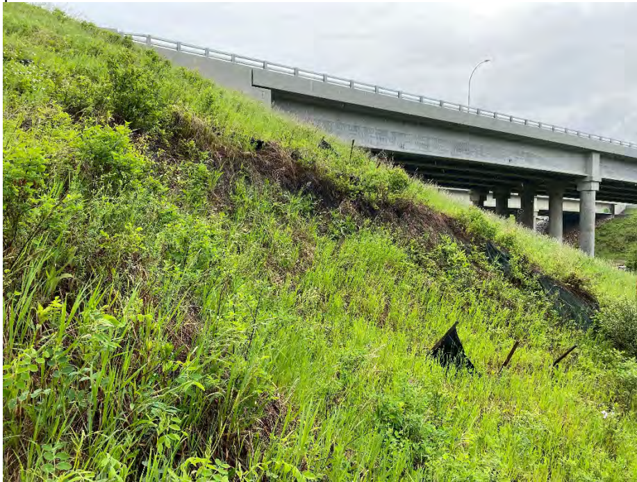
Photo 3: Scarp at south slide. Looking northeast.
