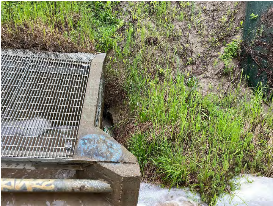
Photo 6: Erosion and wet soil behind west outfall. Looking northwest
