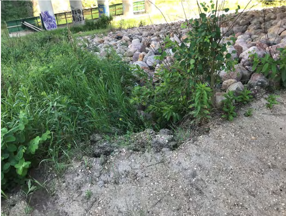
Photo 7: Erosion/slump retrogressing to footpath. Looking southeast.
