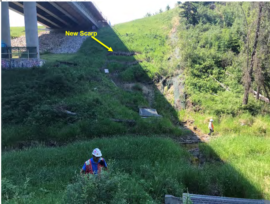
Photo 9: Erosion above west outfall. Looking west.
