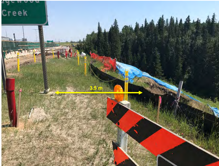
Photo 1: Edge of scarp approximately 3.5 m away from sign pedestal. Looking southeast.
