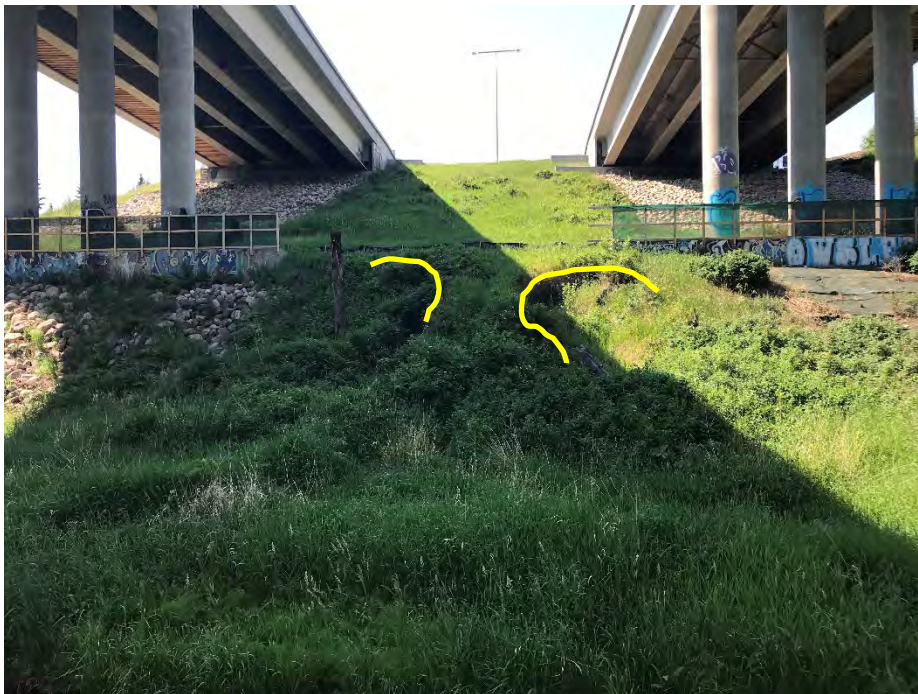
Photo 12: Two slumps between the two concrete pedestals for bridge piers. Looking northwest.
