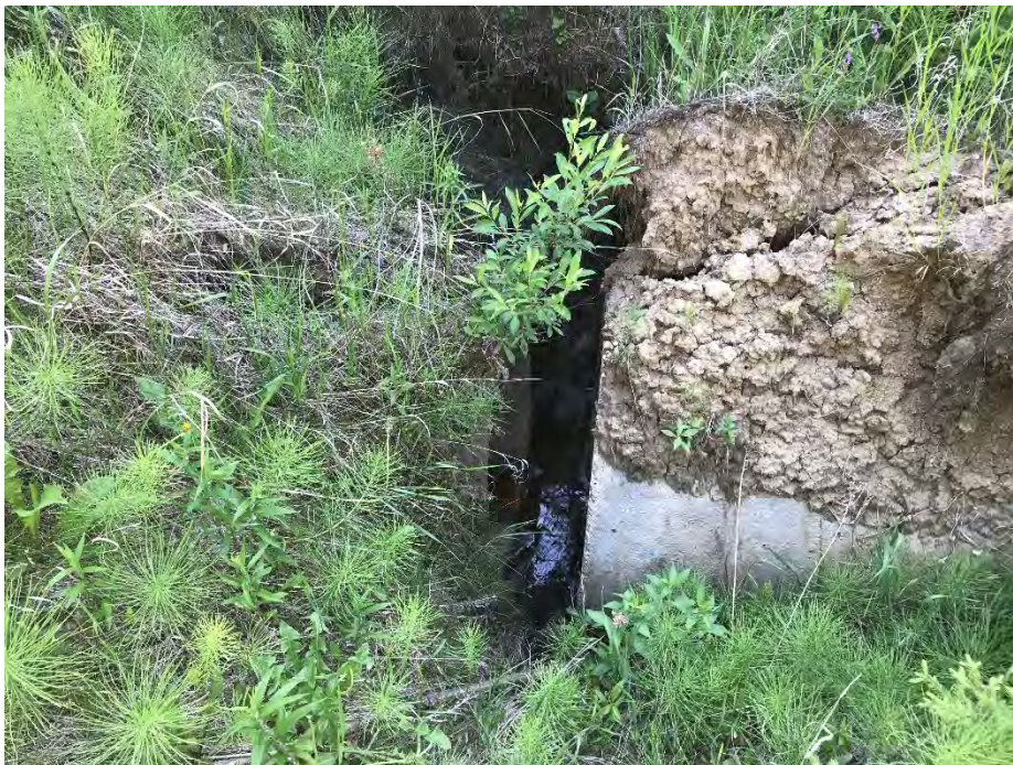
Photo 10: Separation behind east outfall. Looking south.
