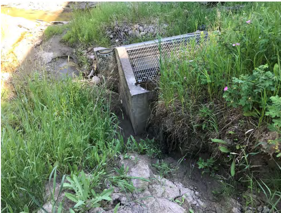
Photo 8: Erosion and wet soil behind west outfall. Looking east
